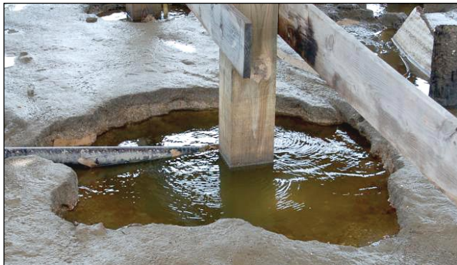
Figure 5. Local scour around foundation piles (Holly Beach, LA, Hurricane Ike).
