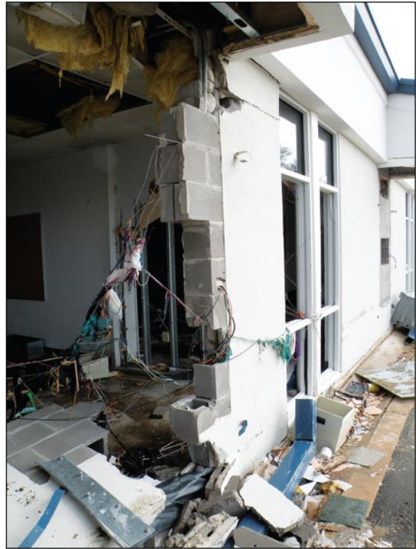
Figure 7. Damage believed to have resulted from Coastal A-zone conditions (Johnson Bayou, LA, Hurricane Ike).
