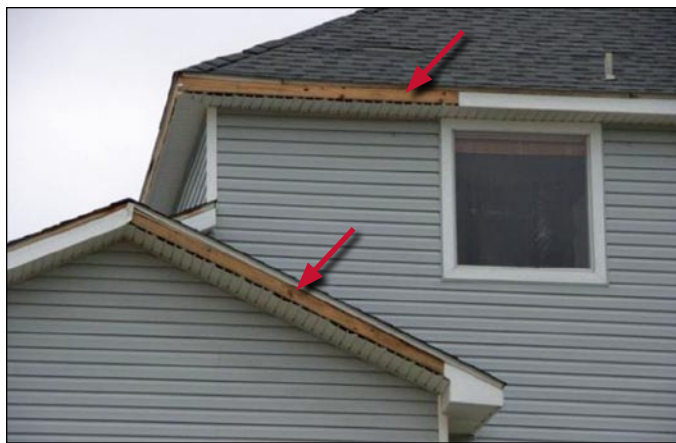
Figure 7. Loss of fascia cover exposes ends of vinyl soffit to direct entry of wind-driven rain.
