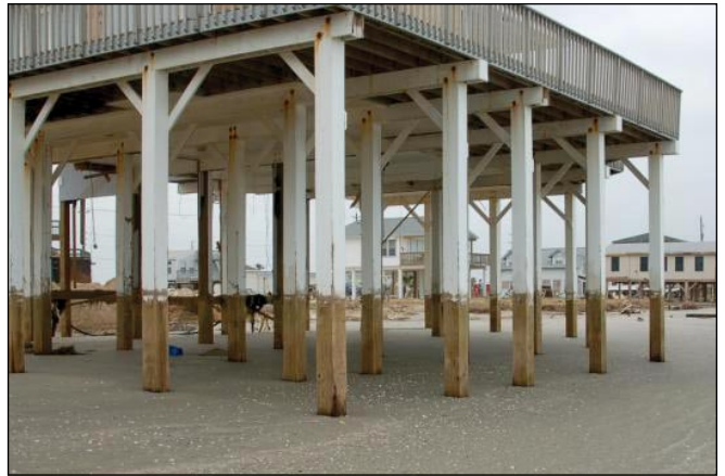
Figure 3. Storm-induced erosion beneath an elevated coastal building (Galveston Island, TX, Hurricane Ike).
