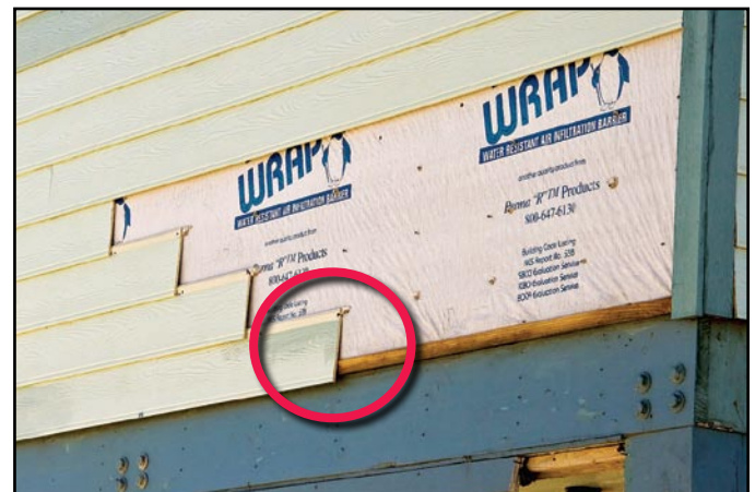
Figure 12. Blind nailed siding installed with exposed gap at bottom (red circle) is vulnerable to failure.
