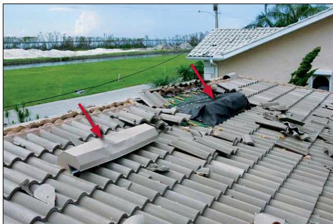
Figure 11. Two off-ridge vents are shown in this photograph. The vent that is covered with roofing felt flipped up and allowed a substantial amount of water to enter the residence. Carpeting, kitchen cabinets, and a large amount of gypsum board had to be replaced because of the water intrusion.
