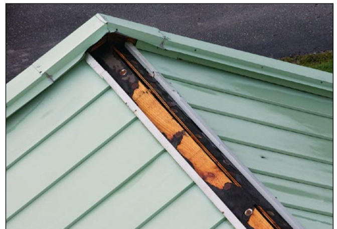
Figure 9. The ridge flashing fasteners were placed too far apart. A significant amount of water leakage can occur when ridge flashings are blown away.
