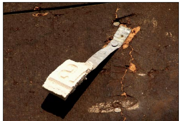
Figure 6. This tie was embedded in the mortar, but the bond was poor.
