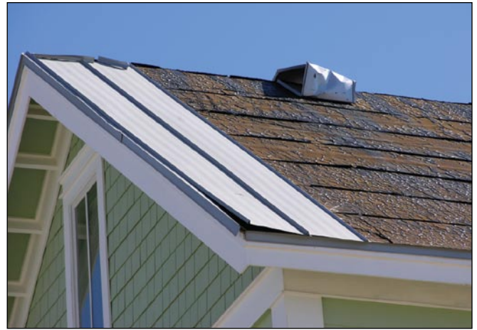
Figure 3. These architectural panel system have snap-lock seams. One side of the seam is attached with a concealed fastener. Although a large number of panels blew away, the underlayment did not.
