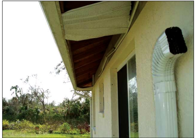
Figure 1. Missing soffit material.
