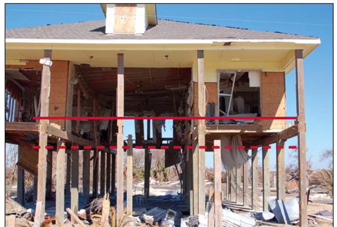
Figure 2. Bolivar Peninsula, TX, V-zone house constructed with the lowest floor (bottom of floor beam) at the BFE (dashed line). The estimated wave crest level during Ike (solid line) was 3 to 4' above the BFE at this location.
