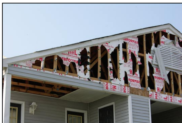
Figure 7. The vinyl siding at this gable was installed over plastic foam insulation. Without wood sheathing, the wind pressures on the vinyl are increased. Also, if the siding blows away, the foam insulation is very vulnerable to blow-off. With loss of the foam insulation, wind-driven rain can freely enter the attic, saturate the ceiling insulation, and cause collapse of the ceiling.
