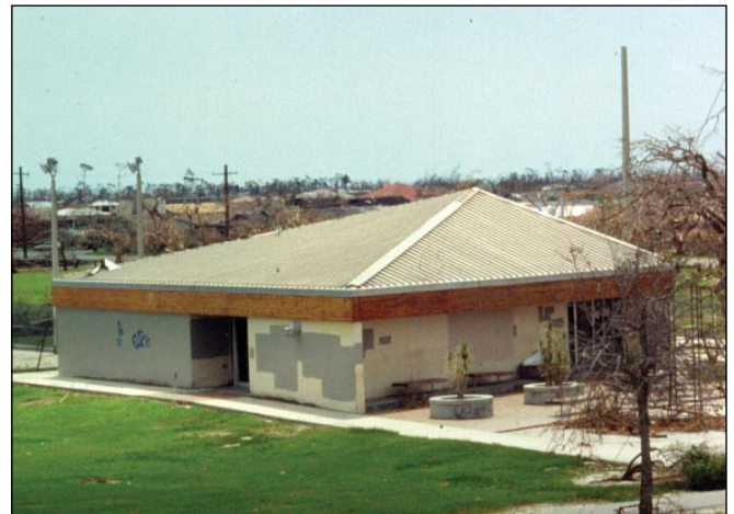
Figure 2. This structural standing seam roof system survived Hurricane Andrew (Florida, 1992), but some hip flashings were blown off. The estimated wind speed was 170 mph (peak gust, Exposure C at 33 feet).
