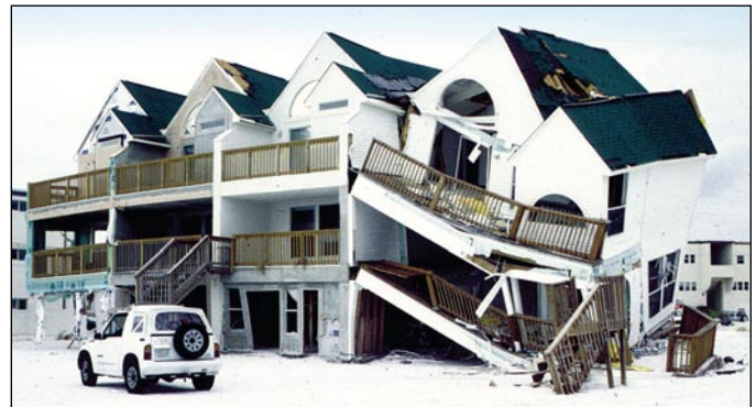
Figure 1. Failure of wood-frame walls used to support a coastal building, which was subjected to shallow flooding, small waves, and floating debris (Fort Walton Beach, FL, Hurricane Opal).
