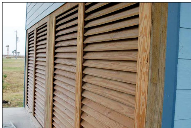
Figure 1. Wood louvers installed beneath an elevated house in a V zone are a good alternative to solid breakaway walls.
