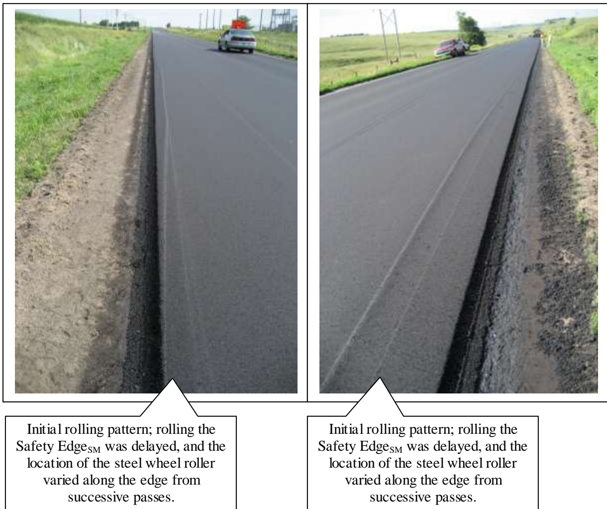
Figure 18. Initial rolling pattern; edge of the breakdown roller varied along the Safety Edge SM , prior to finish rolling.
