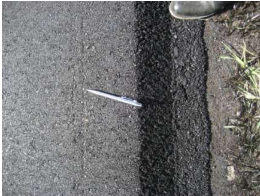
Figure 22. Longitudinal mark left by delaying the breakdown rolling of the Safety Edge SM ; image taken after finish rolling.
