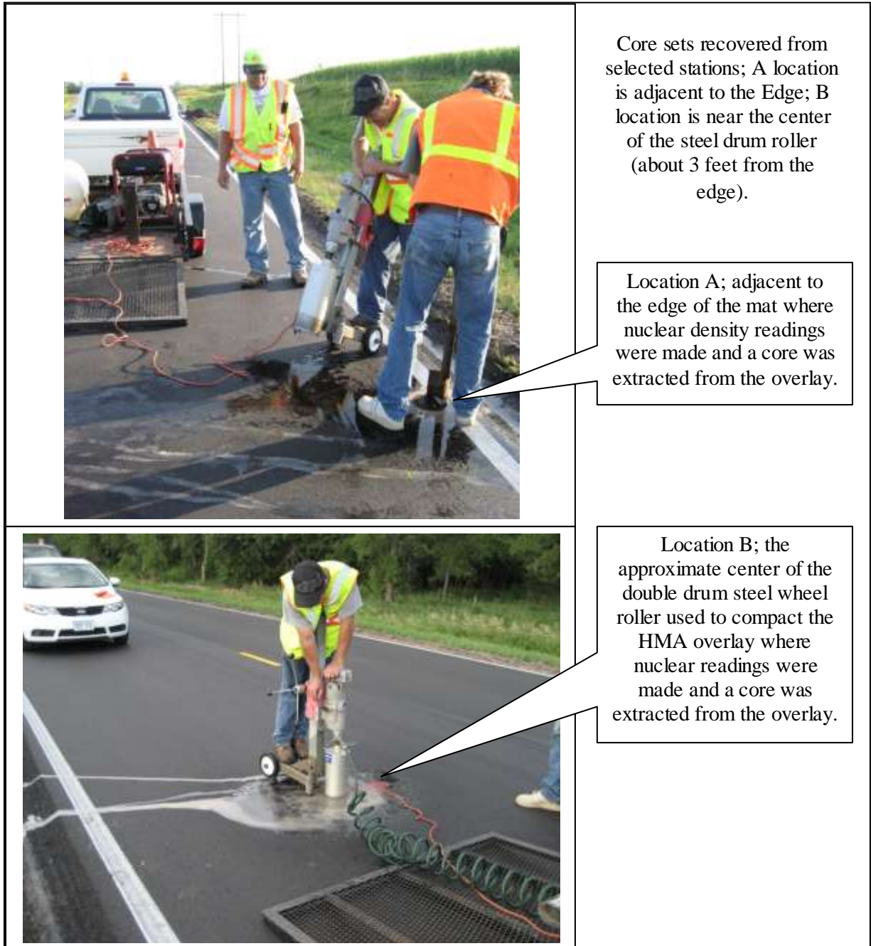
Figure 9. Photos show location of cores and nuclear density tests made with the Troxler gauge (nuclear density readings were taken and then the overlay was cored).
