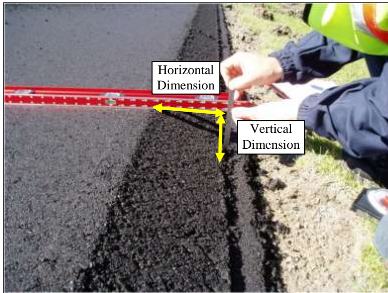
Figure 2. Slope measurement technique.
