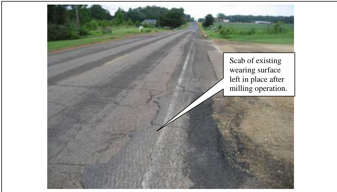
Figure 3. General overview of the existing HMA pavement after milling; heavily distressed area with cracking (view is towards the east).
