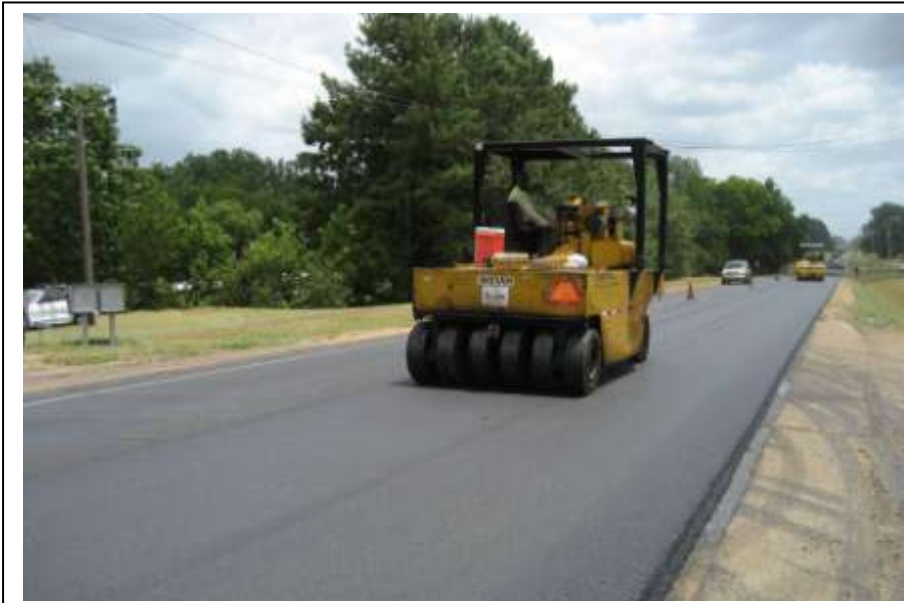
Ingram pneumatic or rubber tired roller (5x6 tires) that was used in the intermediate position.
