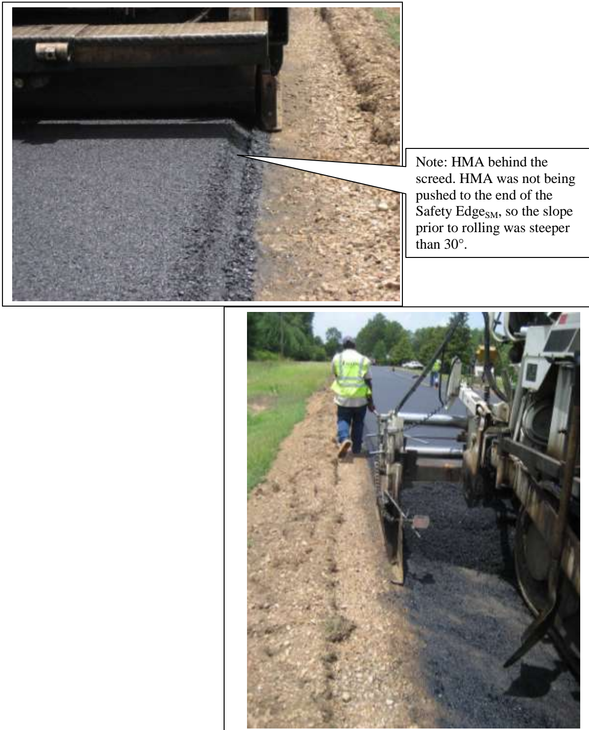
Figure 22. HMA under and behind the screed; the HMA was not being pushed to the end of the Safety Edge SM , which resulted in a steeper slope prior to rolling.
