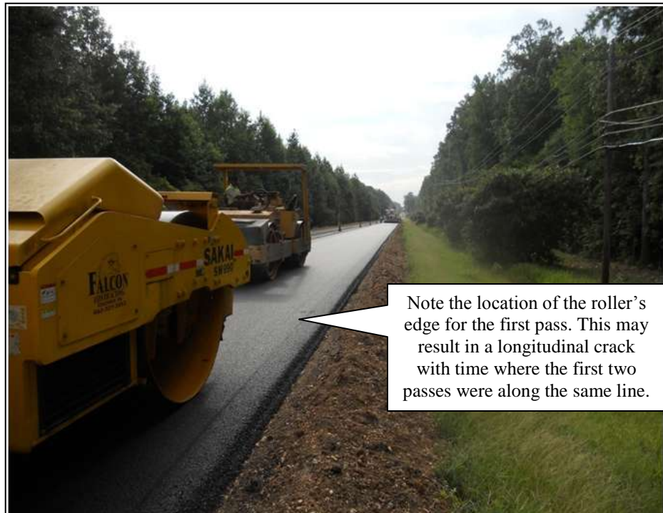
(b) First pass of Sakai roller is about 6 to 12 inches away from edge of the mat.
