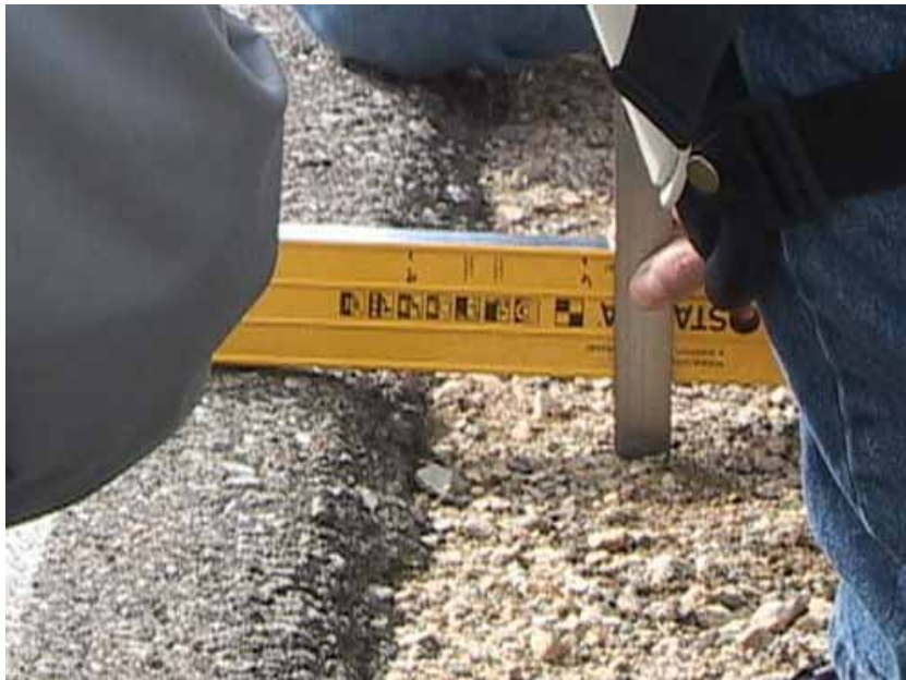
Figure 11. Photo. Measurement of pavement-edge drop-off height.
