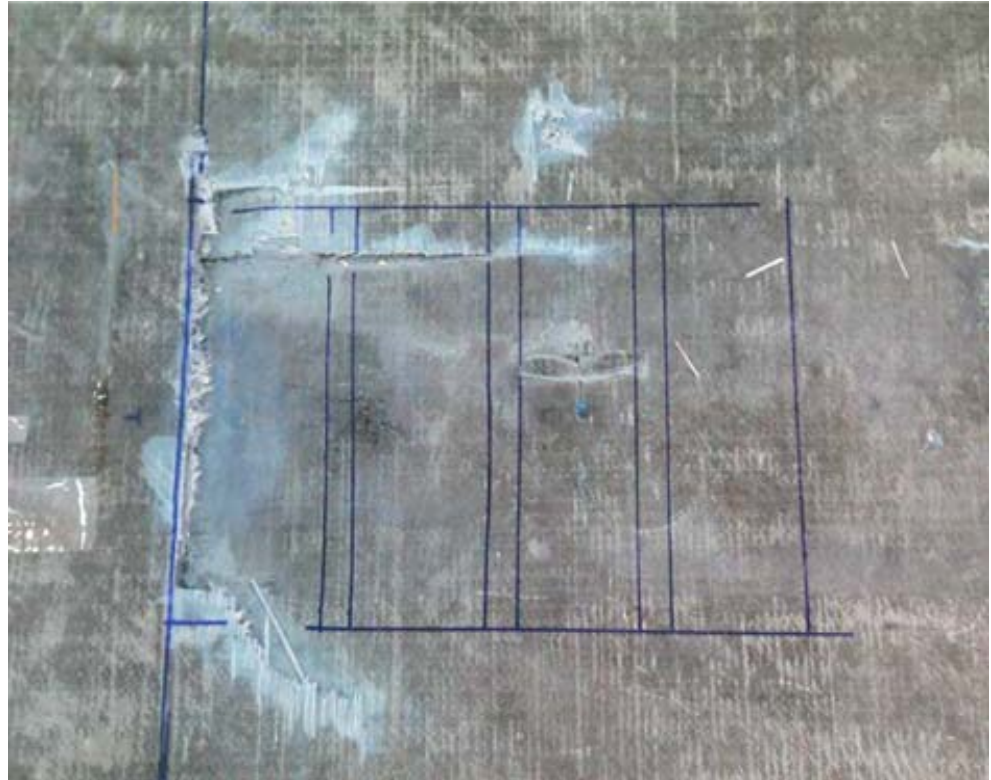
Figure 6.6.19 Cracks and Discoloration Around Punched Area
