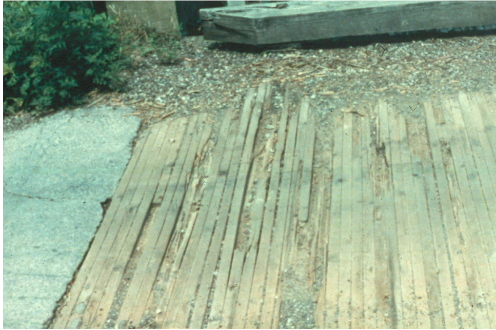
Figure 7.1.8 Wear and Weathering on a Timber Deck
