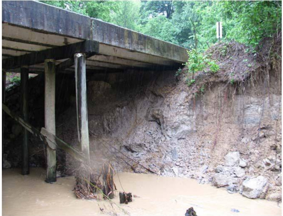
Figure 13.2.17 Lateral Stream Migration Endangering an Abutment
