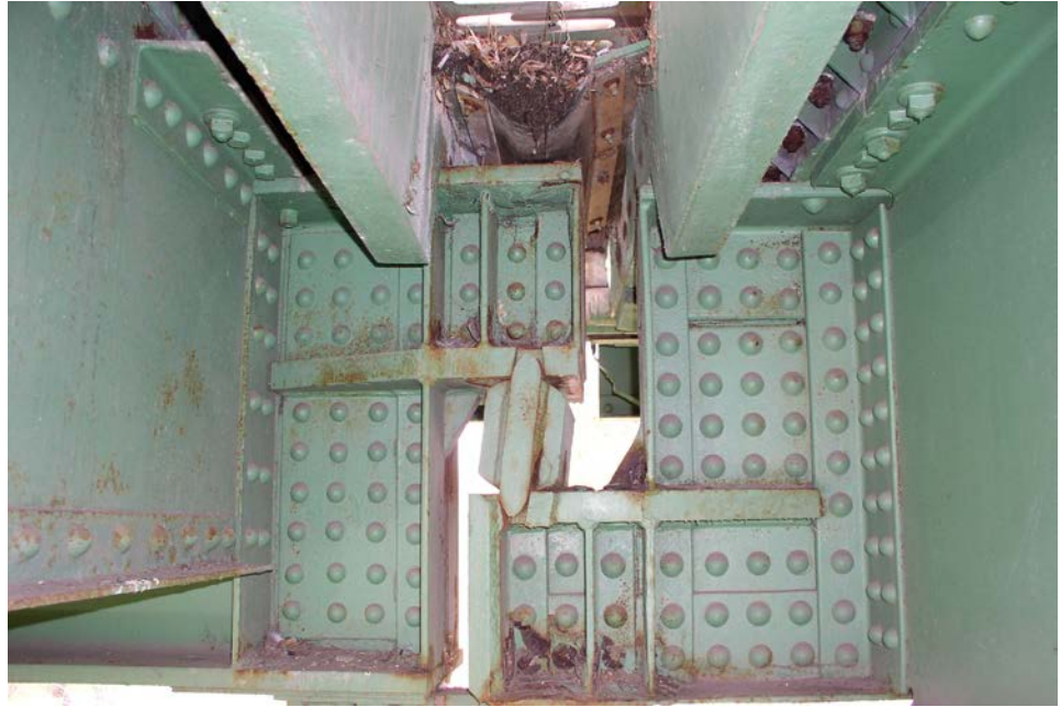
Figure 7.5.32 Drainage Trough with Debris Accumulation
