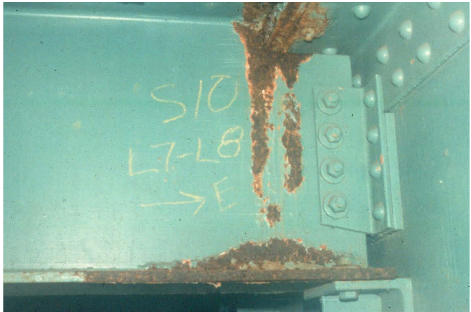
Figure 10.4.54 Corroded End of Stringer
