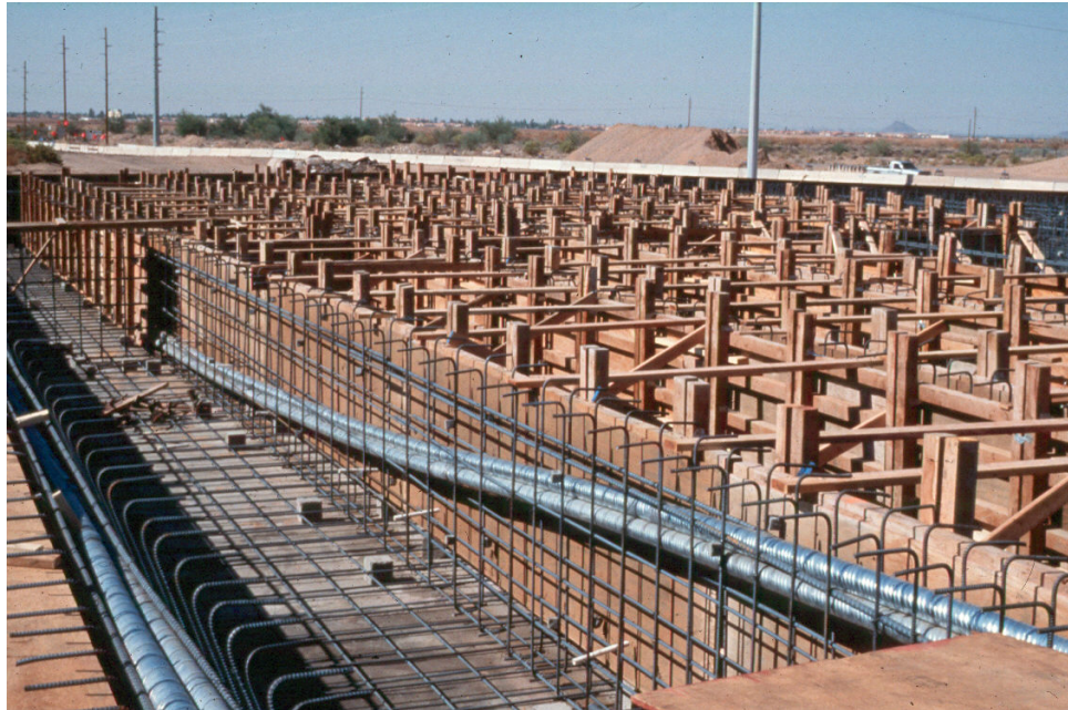
Figure 9.11.41 Post-tensioning Tendon Duct
