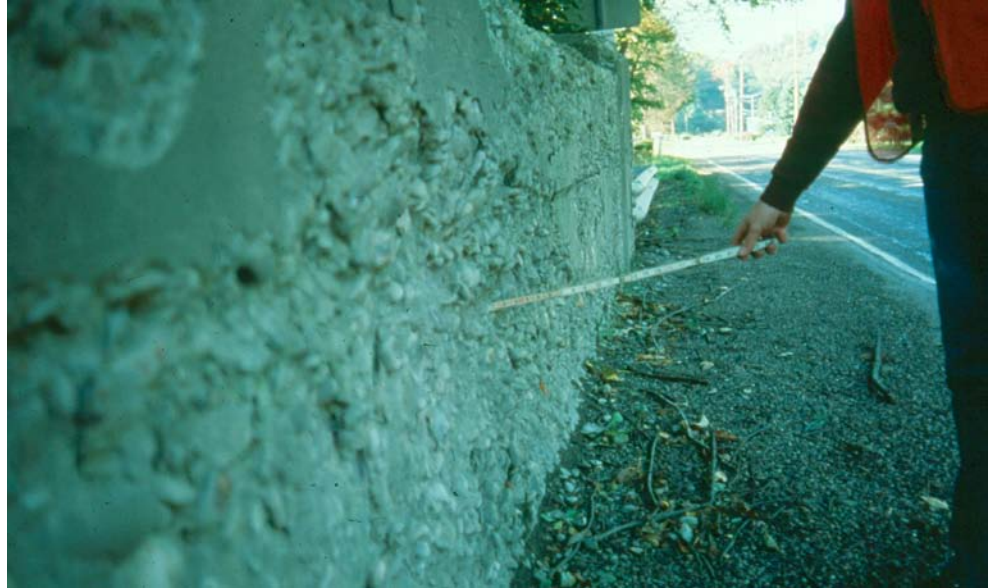
Figure 9.3.9 Close-up of an Interior Face of a Through Two-Girder with Heavy Scaling due to Deicing Agents
