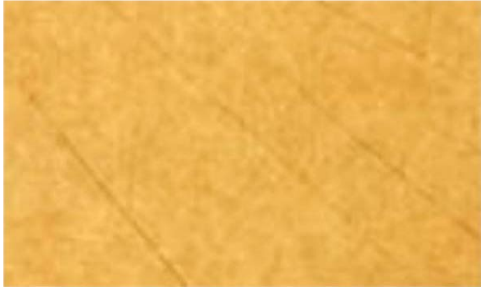
Figure 6.6.18 Scratches on FRP Surface
