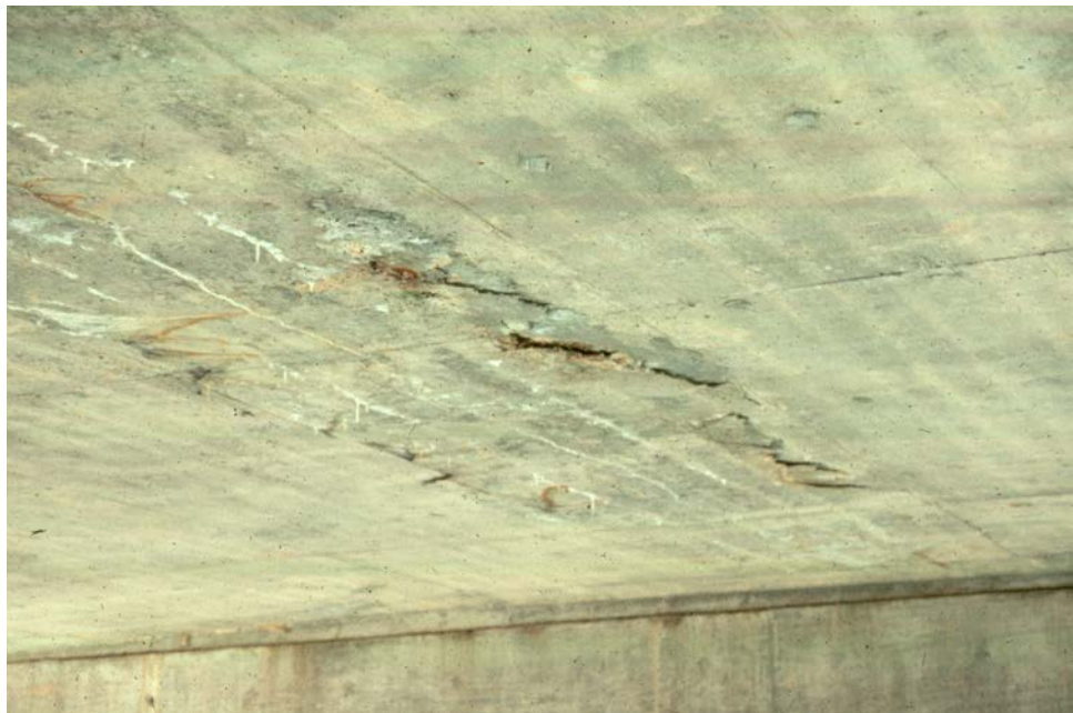
Figure 9.1.8 Concrete Slab Tension Zone: Delamination, Efflorescence, Rust, and Stains
