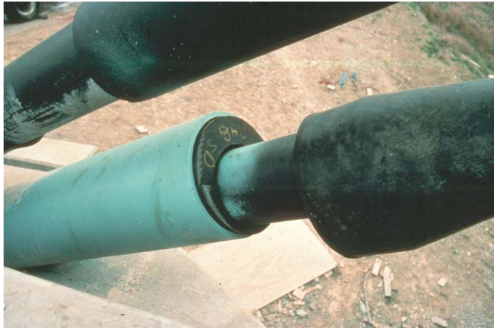
Figure 16.1.52 Neoprene Boot at Steel Anchor Pipe Near Anchor
