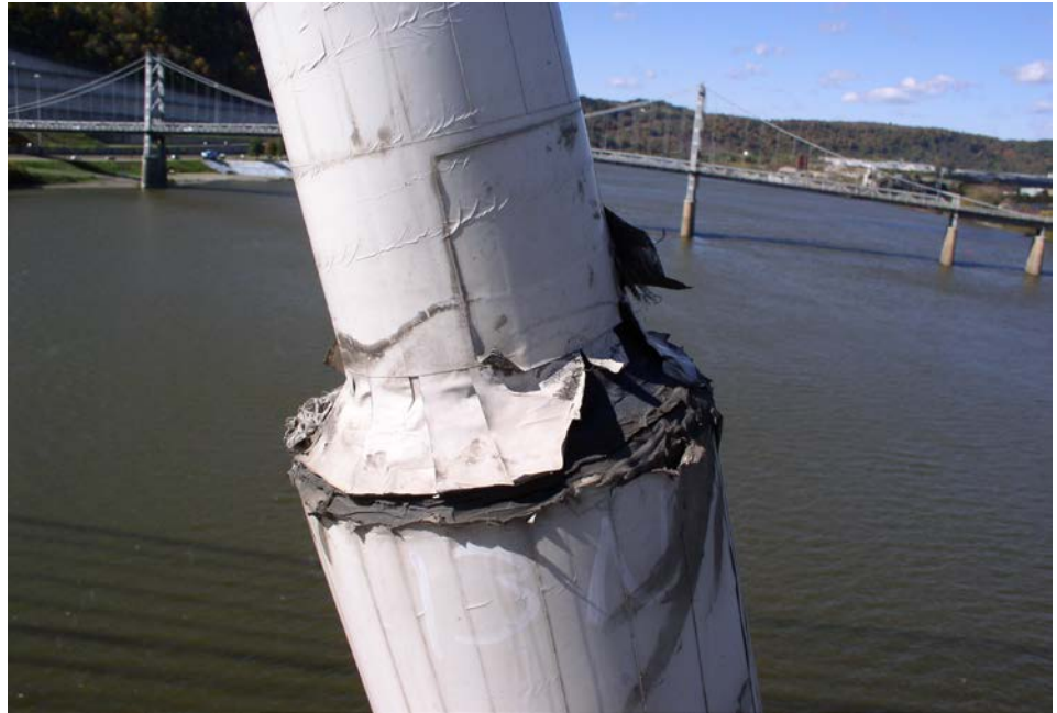
Figure 16.1.38 Tape and Rubber Seal Torn Around Cable Allowing Water Penetration into Top of Sheath
