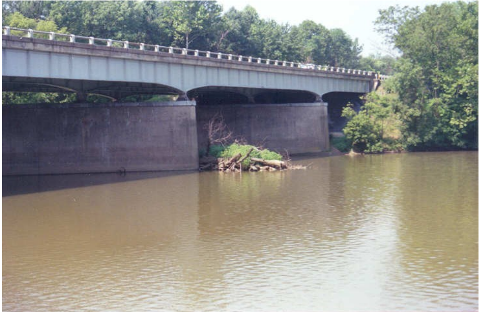
Figure 13.3.11 Buildup of Debris At Pier
