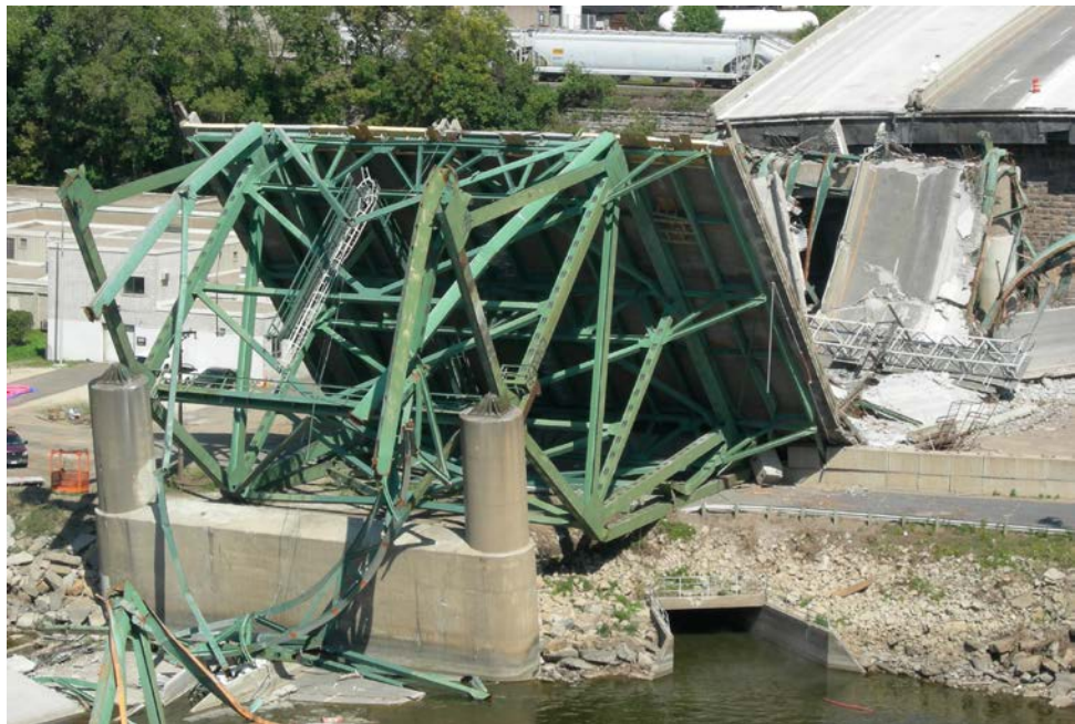
Figure 6.4.3 I-35W Mississippi River Bridge Collapse
