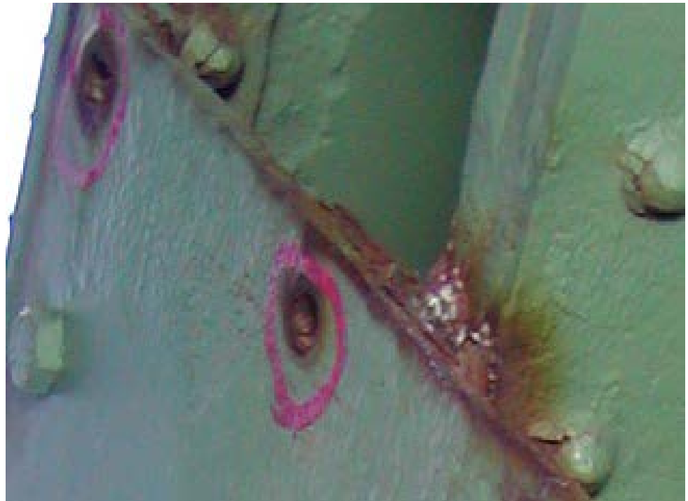
Figure 10.8.29 Missing Bolts on Gusset Plate
