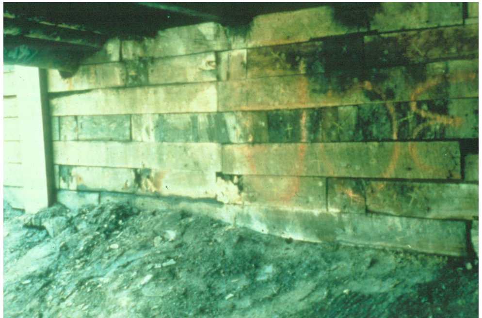
Figure 12.1.36 Decay caused by insects in Timber Abutment
