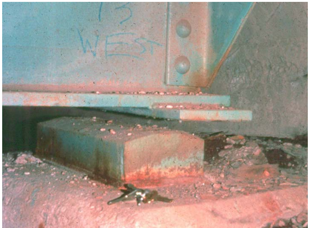
Figure 11.1.31 Uplift at Bridge Bearing
