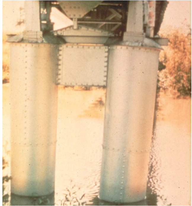
Figure 12.2.49 Tipping of Bent due to Scour/Undermining
