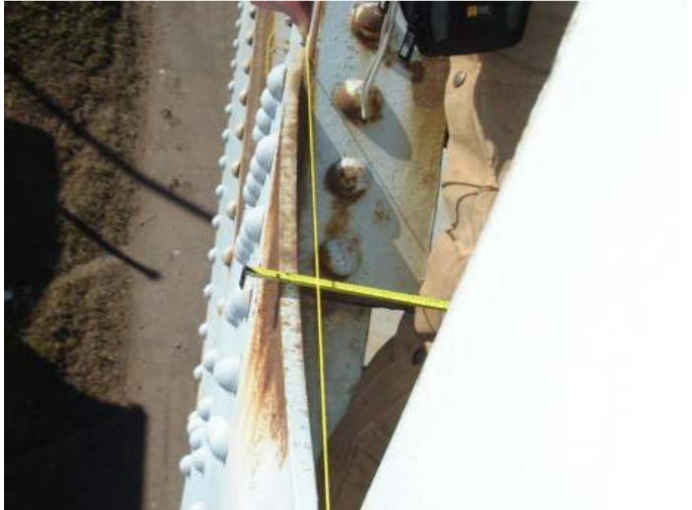
Figure 10.8.33 Inspector Measuring Out-of-Plane Distortion Using String Line and Tape Measure
