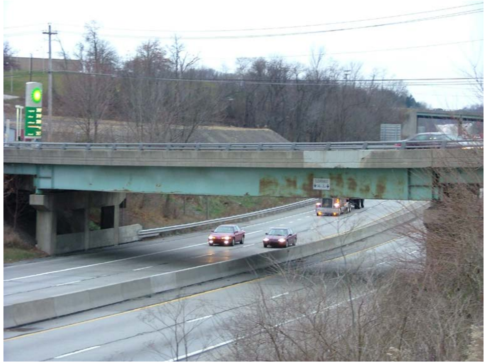
Figure 6.3.25 Roadway Spray Zone Deficiency
