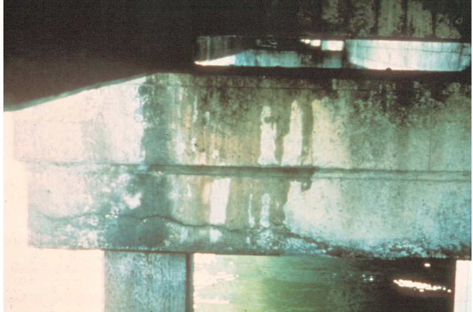
Figure 12.2.31 Crack in Concrete Bent Cap
