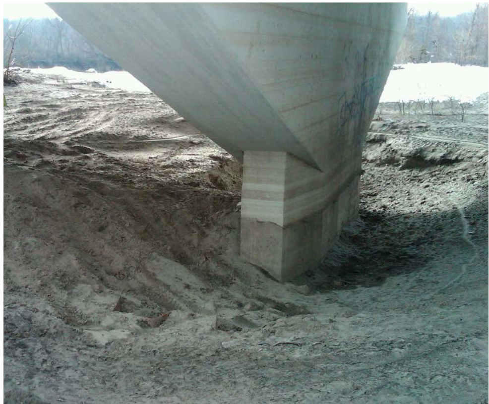
Figure 13.2.14 Local Scour at a Pier
