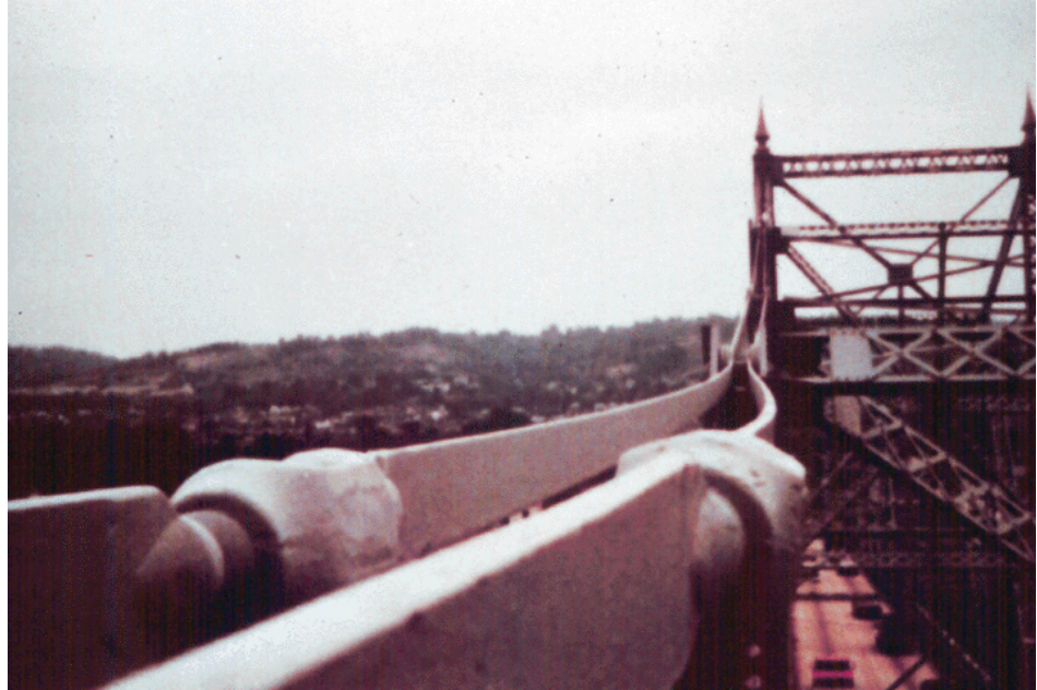
Figure 10.9.21 Bowed Eyebar Member
