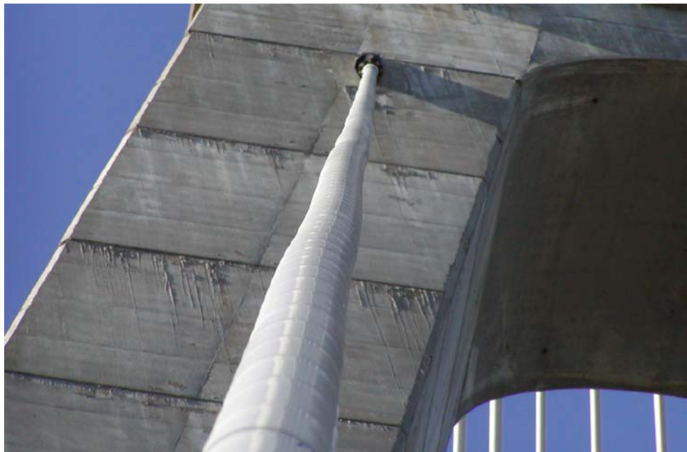
Figure 16.1.45 Bulging of Cable Sheathing
