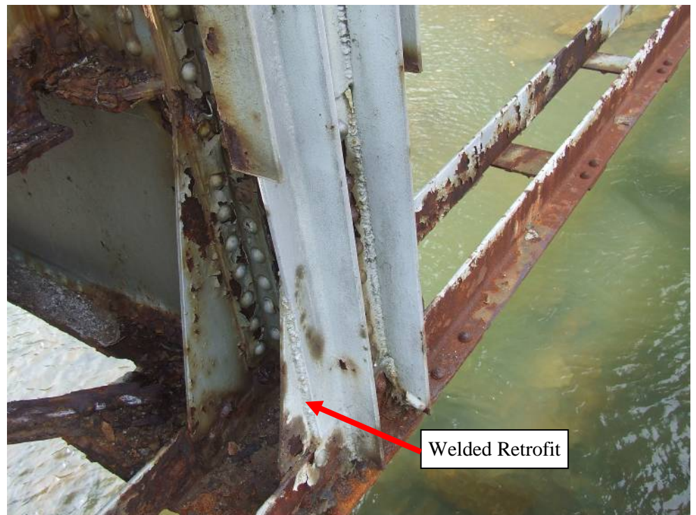
Figure 10.8.31 Poorly Designed Welded Retrofit
