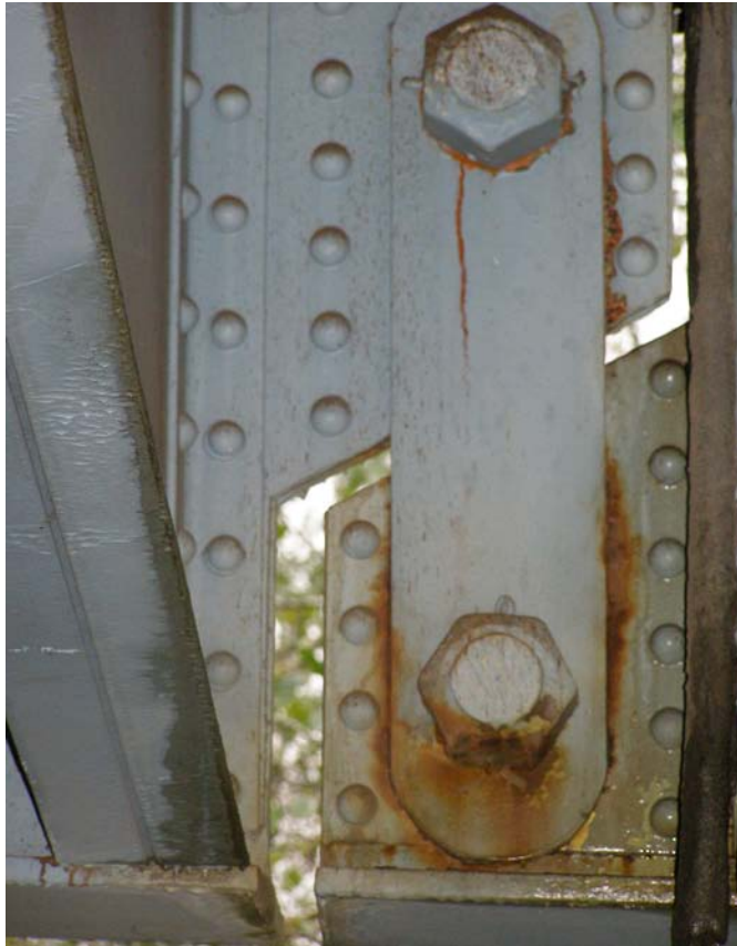
Figure 10.7.20 Rust Stains from Pin Corrosion
