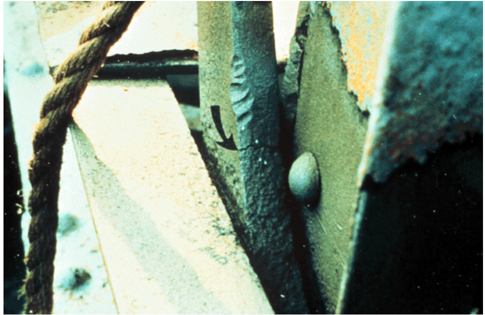
Figure 10.9.19 Close-up of the Forge Zone on an Eyebar (Arrow denotes crack)
