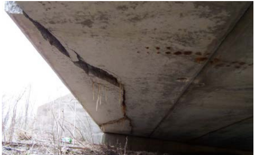
Figure 9.10.18 Close-up of Box Beam Collision Damage
