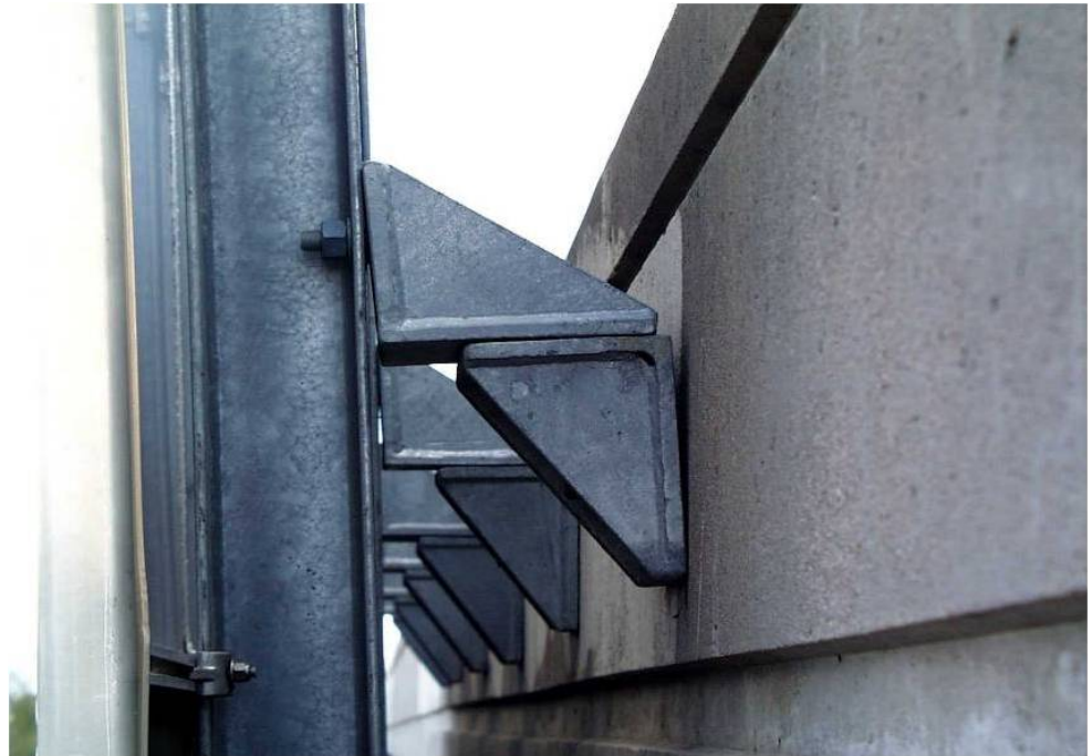
Figure 7.5.35 Sign Mount with Loose Adhesive Anchorage
