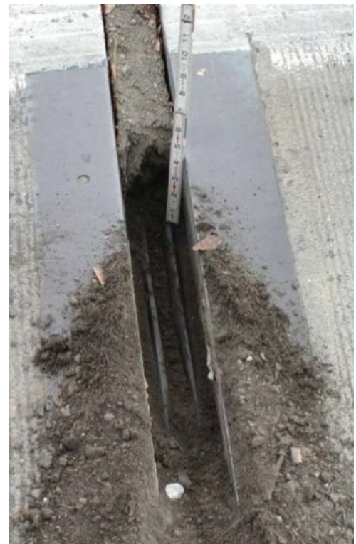
Figure 7.5.25 Dirt in a Compression Seal Joint
