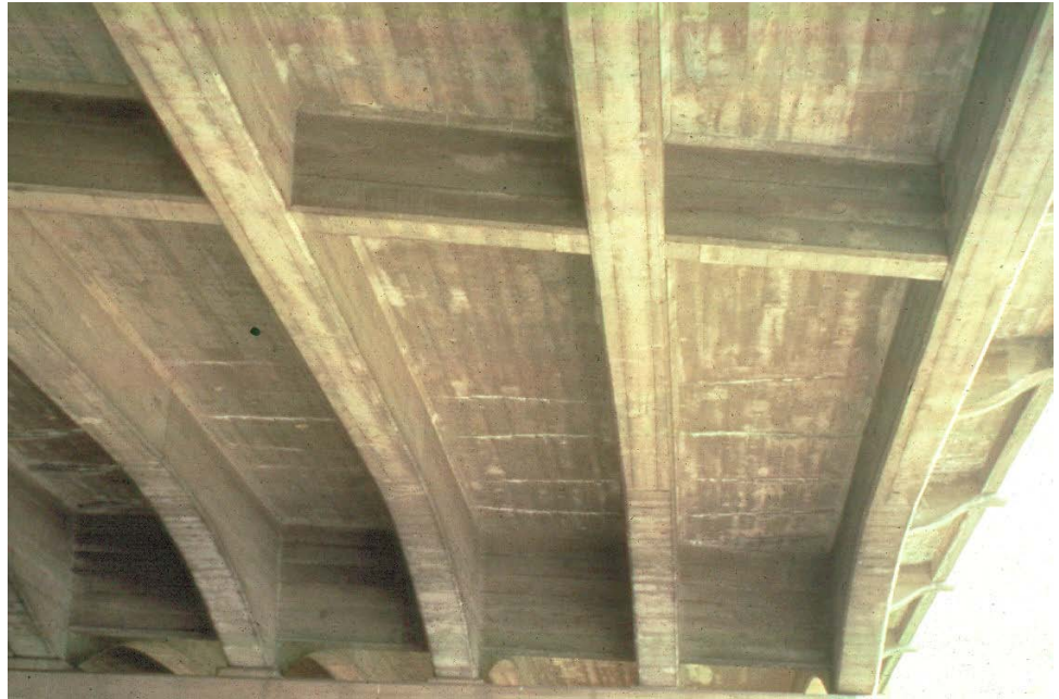
Figure 9.2.14 Flexure Cracks in Tee Beam Flange/Deck
