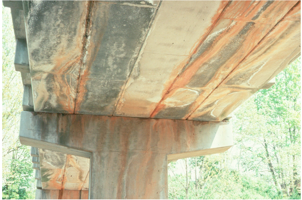
Figure 9.10.17 Joint Leakage and Rust Stain
