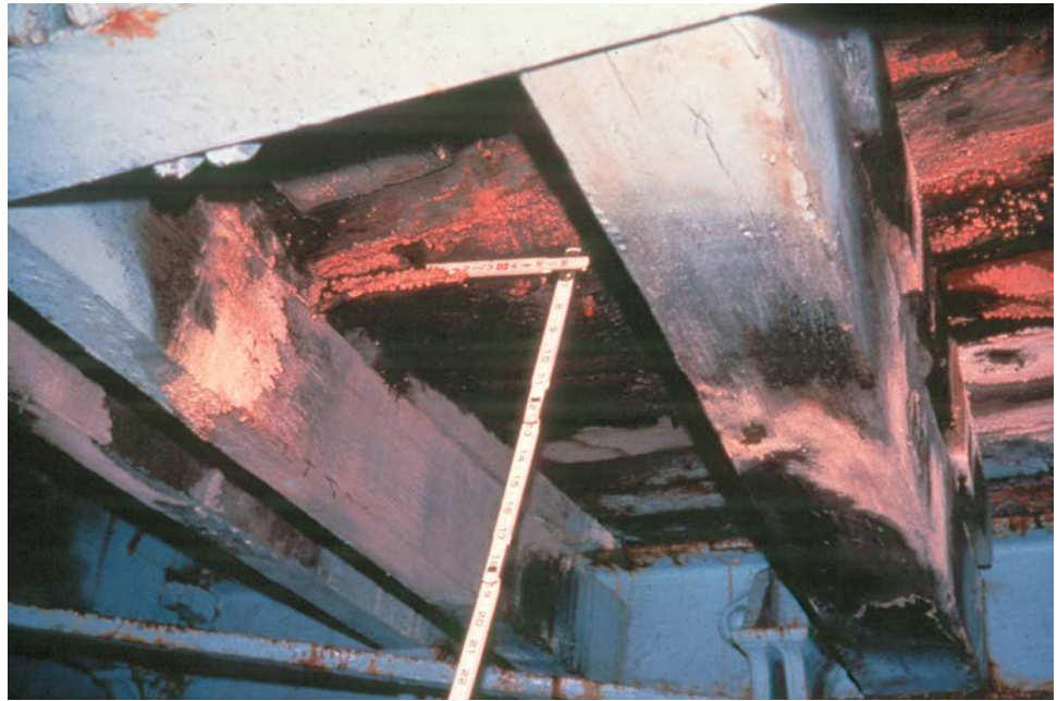
Figure 8.1.13 Decay in a Timber Beam
