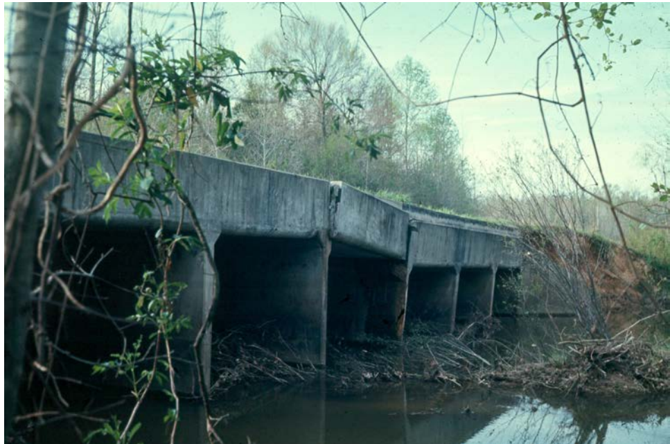
Figure 13.2.57 Rotational Movement and Failure Due to Undermining
