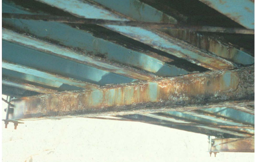
Figure 10.4.55 Corroded Floorbeams and Stringers
