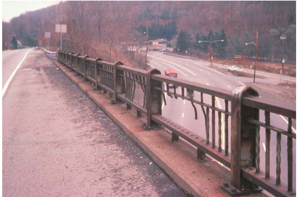
Figure 7.6.12 Deficiency Steel Post Bridge Railing
