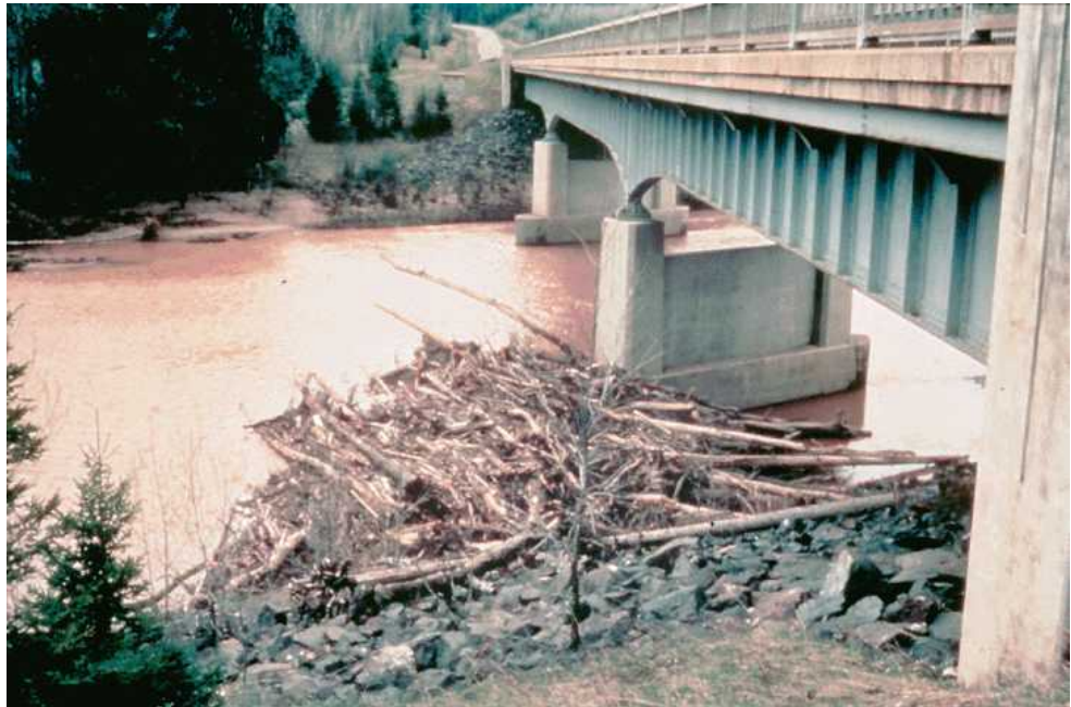
Figure 13.2.12 Debris Build-up in the Waterway
