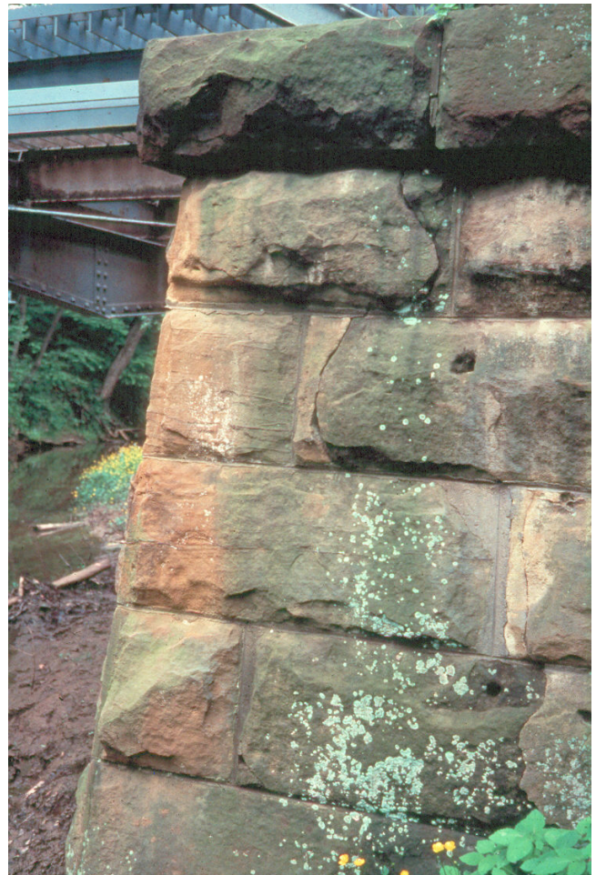
Figure 6.5.2 Splitting in Stone Masonry
