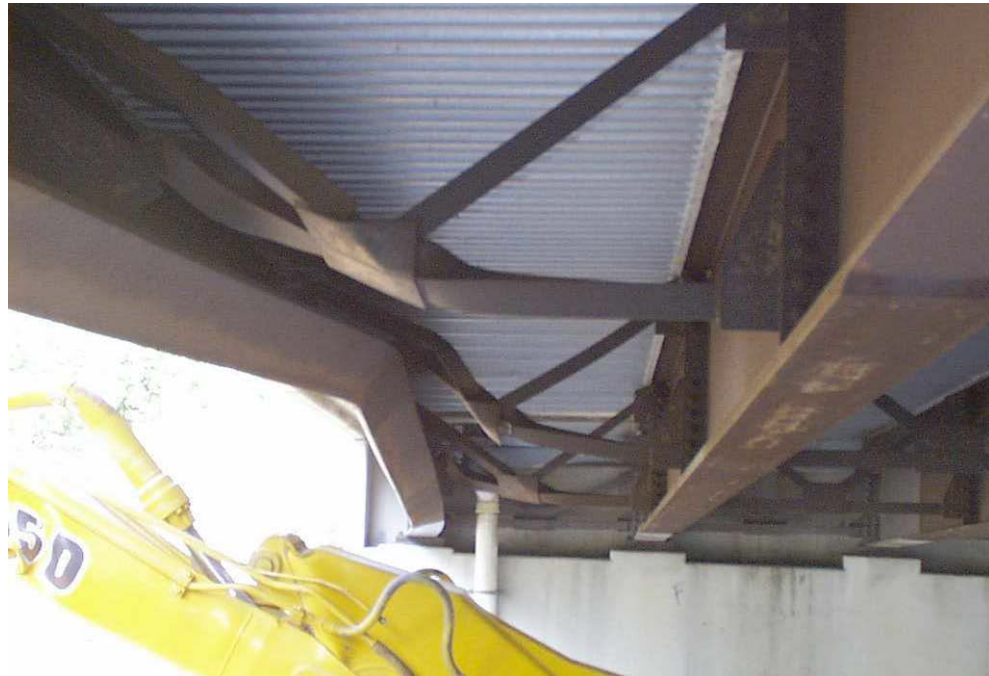
Figure 6.4.31 Severe Collision Damage on a Fascia Girder
