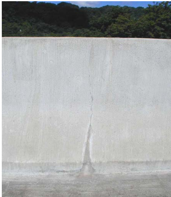
Photo No.16 Typical parapet crack
