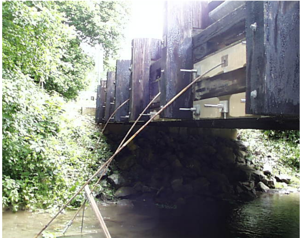
Figure 8.3.10 Broken Stressing Rods
