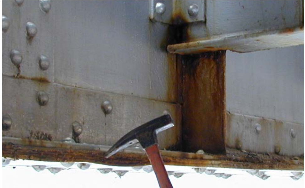
Figure 6.3.20 Corrosion of Steel
