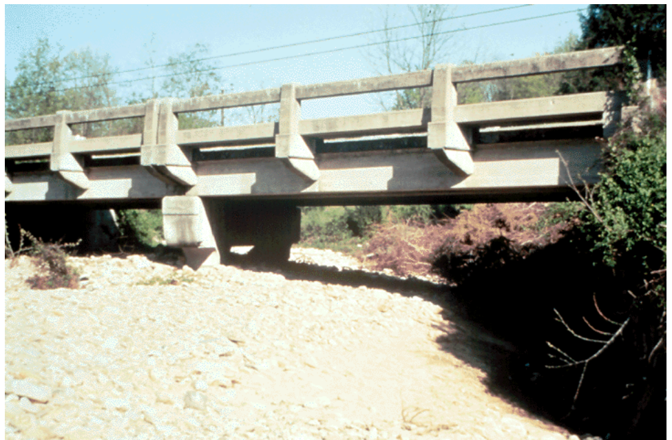
Figure 13.2.10 Sediment Deposits Within the Waterway Opening
