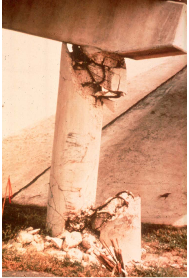
Figure 12.2.33 Collision Damage to Concrete Pier Column
