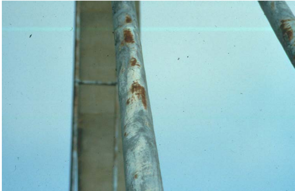
Figure 16.1.44 Corrosion of Steel Sheathing
