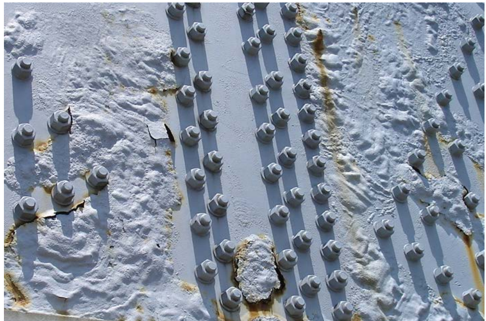
Figure 10.8.28 Gusset Plate with Paint Failure
