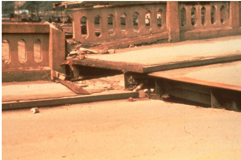
Figure 12.2.46 Superstructure Evidence of Pier Settlement
