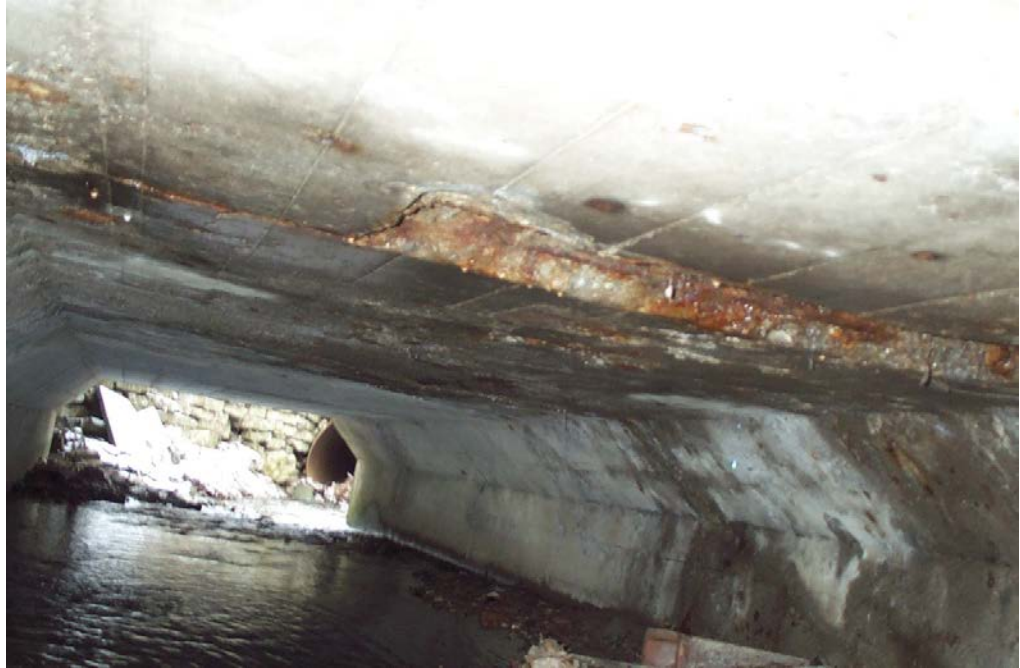
Figure 14.2.17 Spalls and Delaminations on Top Slab of Concrete Box Culvert
