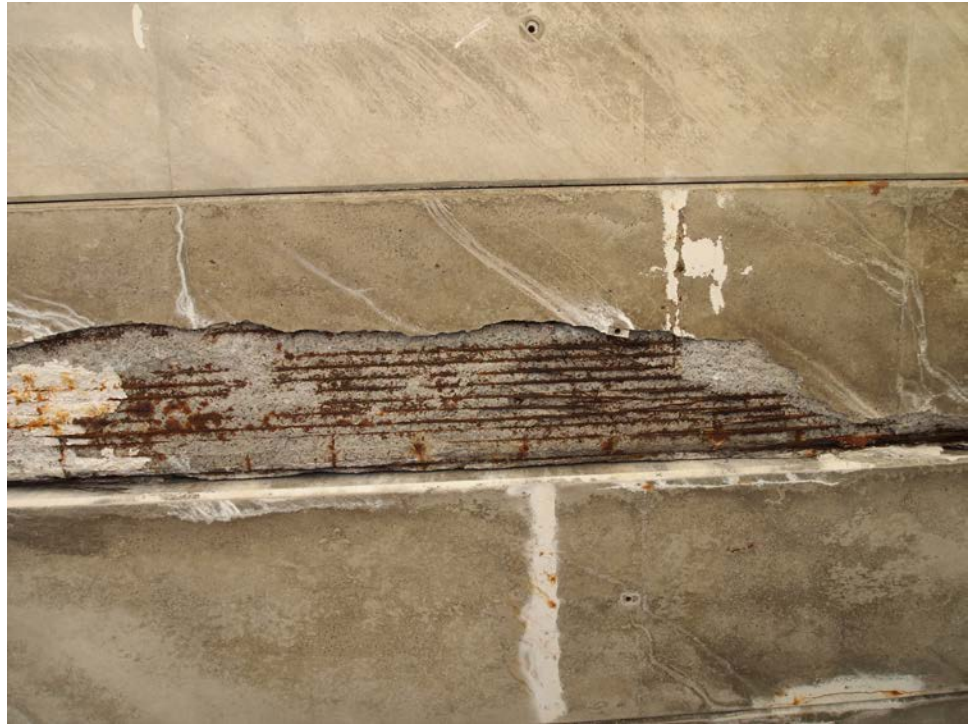
Figure 9.10.15 Spall and Exposed/Corroded Reinforcement
