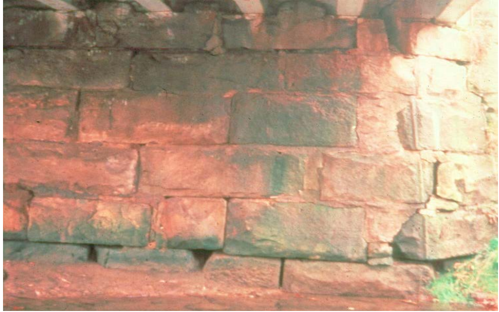
Figure 12.1.34 Stone Masonry Abutment with Deteriorated Joints
