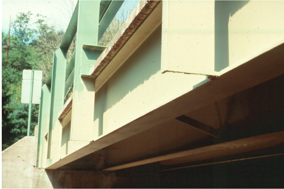
Figure 6.4.64 Welded Attachment in Tension Zone of a Beam
