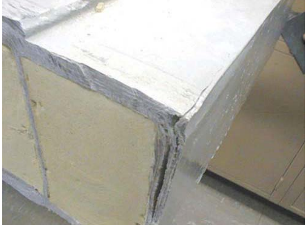
Figure 6.6.15 Voids Resulting in Surface Cracks
