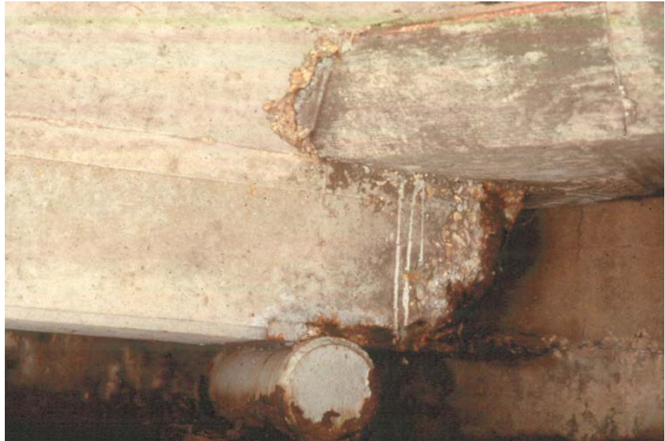
Figure 9.2.9 Spalled Tee Beam End
