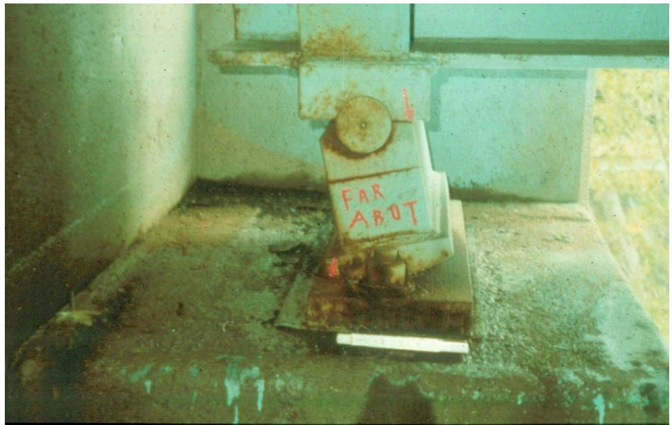
Figure 11.1.43 Broken Pintle on a Bearing
