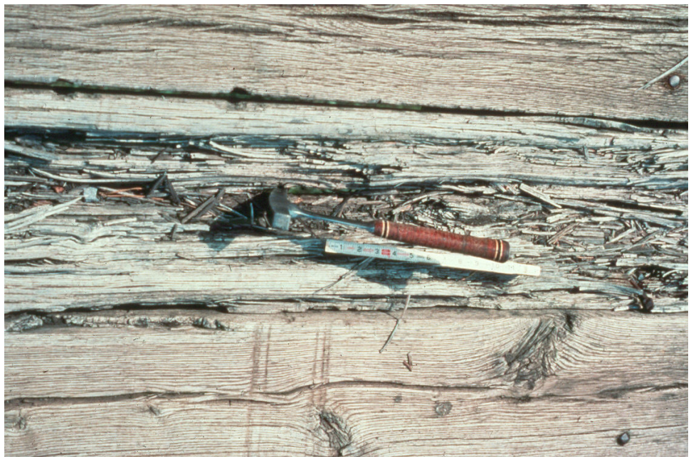
Figure 6.1.26 Weathering on Timber Deck
