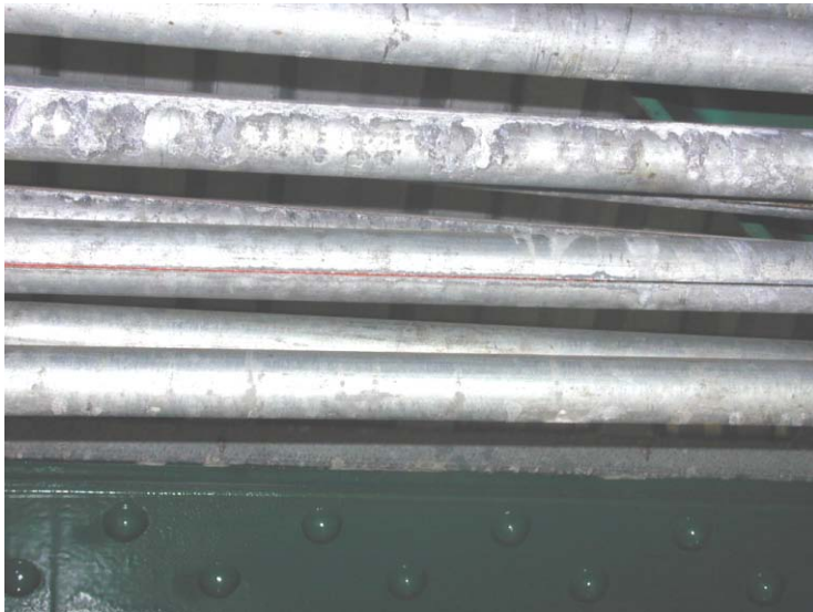
Photo No. 12 Conduit, Span 1 – note longitudinal crack/split
