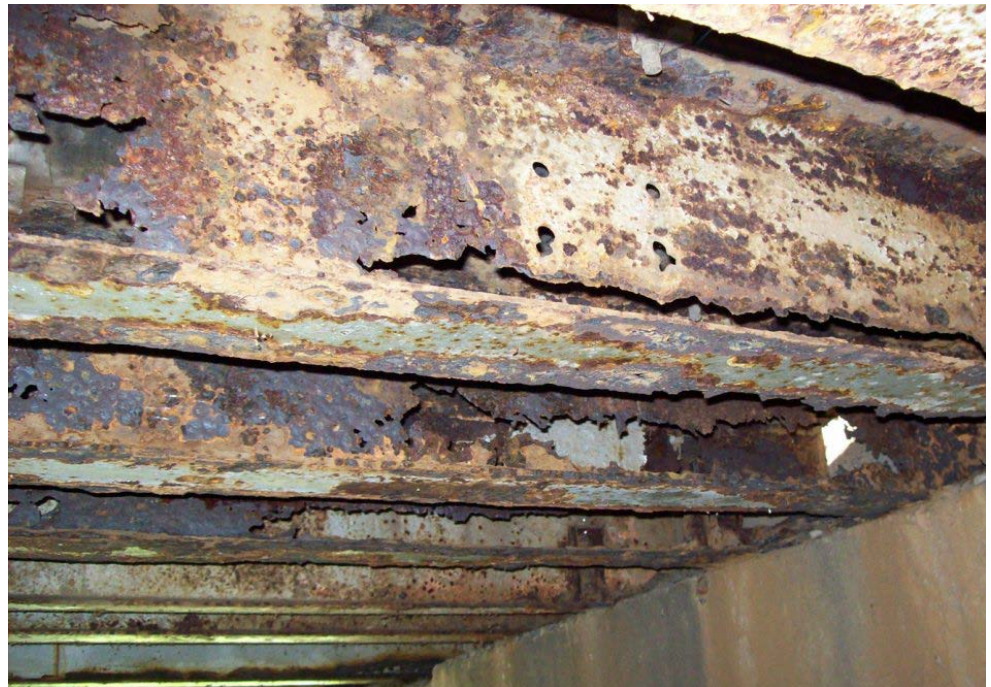
Figure 6.3.10 Steel Corrosion and Complete Section Loss on Girder Webs
