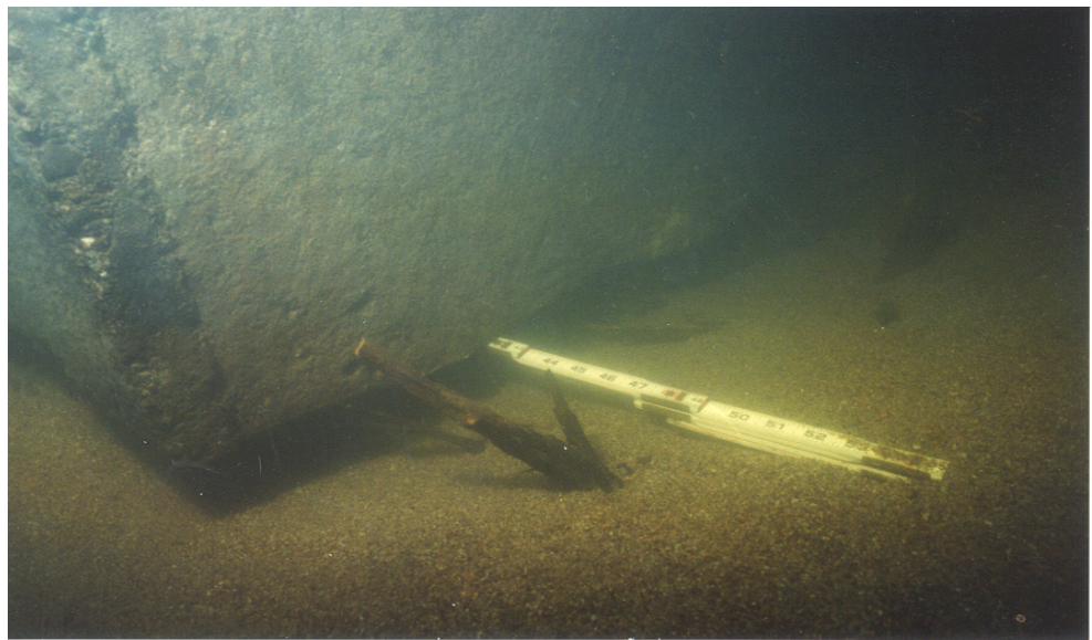
Figure 13.3.8 Local Scour; Causing Undermining of a Pier
