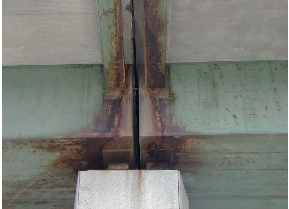
Figure 6.3.23 Water and Salt Runoff Near Expansion Joint
