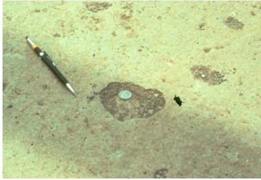
Figure 6.2.20 Light or Minor Scaling
