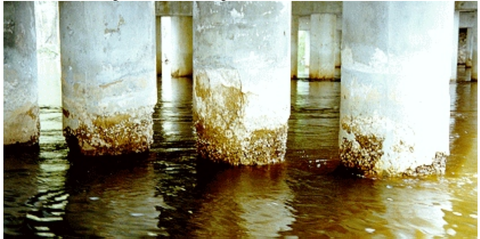
Figure 13.2.35 Pile Bent Deterioration Normally Hidden Underwater
