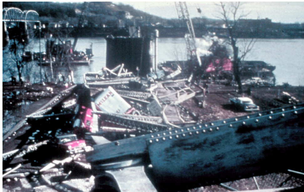
Figure 6.4.1 Silver Bridge Collapse
