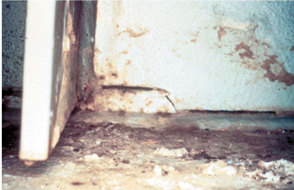
Figure 6.4.42 Through-Crack Ready to Propagate into the Flange
