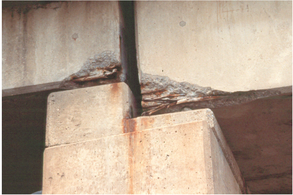
Figure 9.10.11 Spalled Beam Ends with Exposed Prestressing Reinforcement
