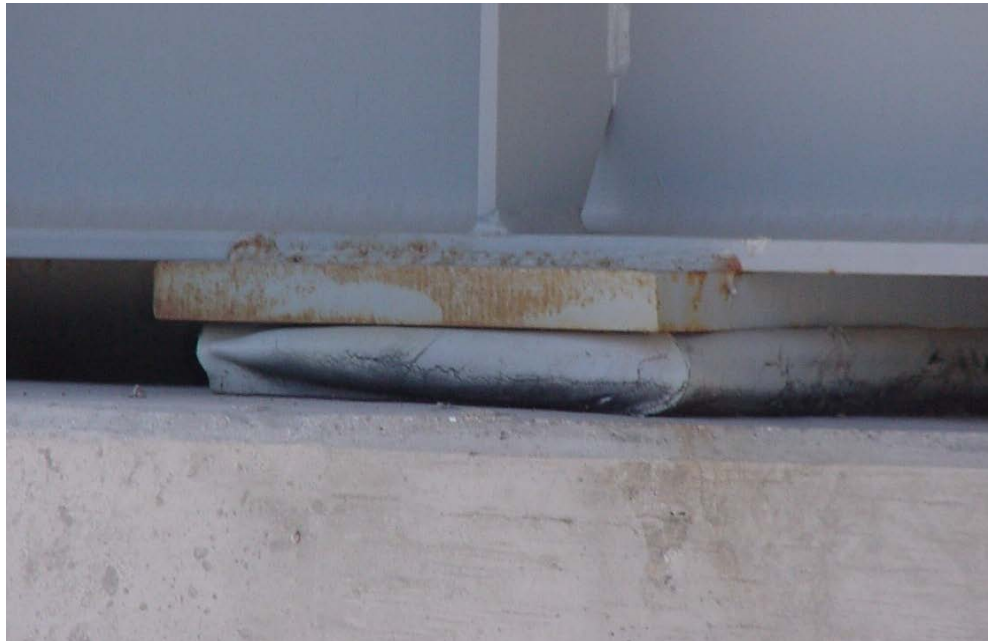
Figure 11.1.40 Neoprene Bearing Pad Excessive Bulging
