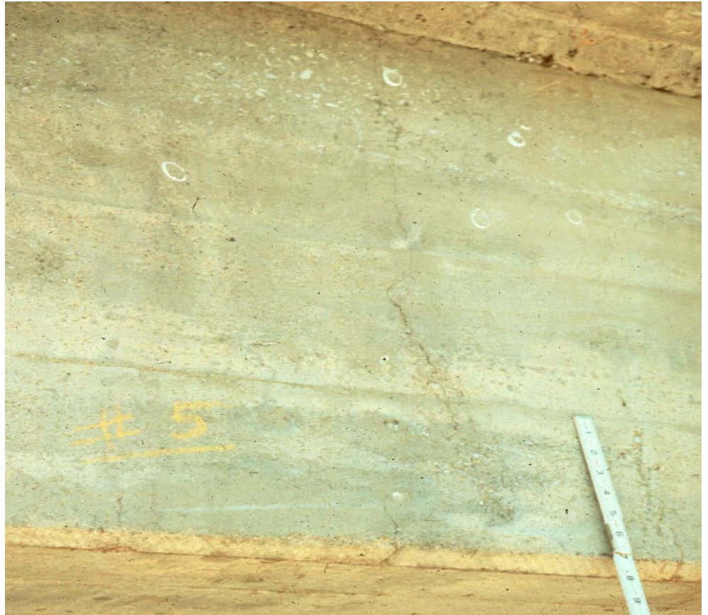
Figure 6.2.12 Flexural Crack on a Tee Beam
