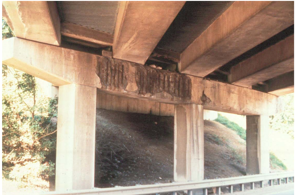
Figure 12.2.32 Concrete Spalling on Bent Cap
