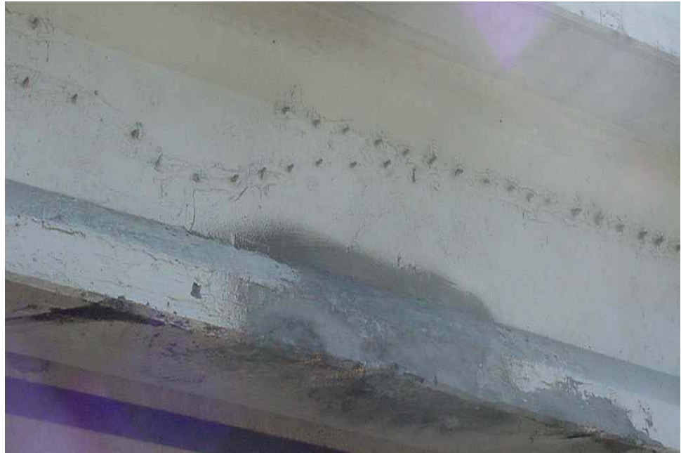
Figure 9.9.21 Collision Damage Repair on Prestressed Concrete I-Beam. Note Epoxy Injection Ports and Guniting Repair
