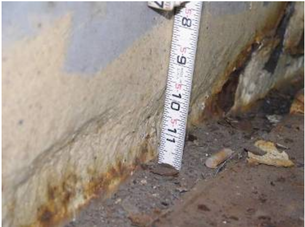
Figure 10.8.21 Inspector Using a Straightedge and Tape to Measure the Section Loss of the Gusset Plate
