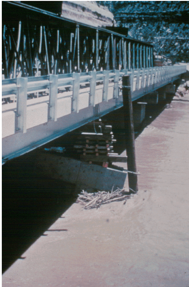
Figure 13.2.27 Pier Settlement due to Undermining
