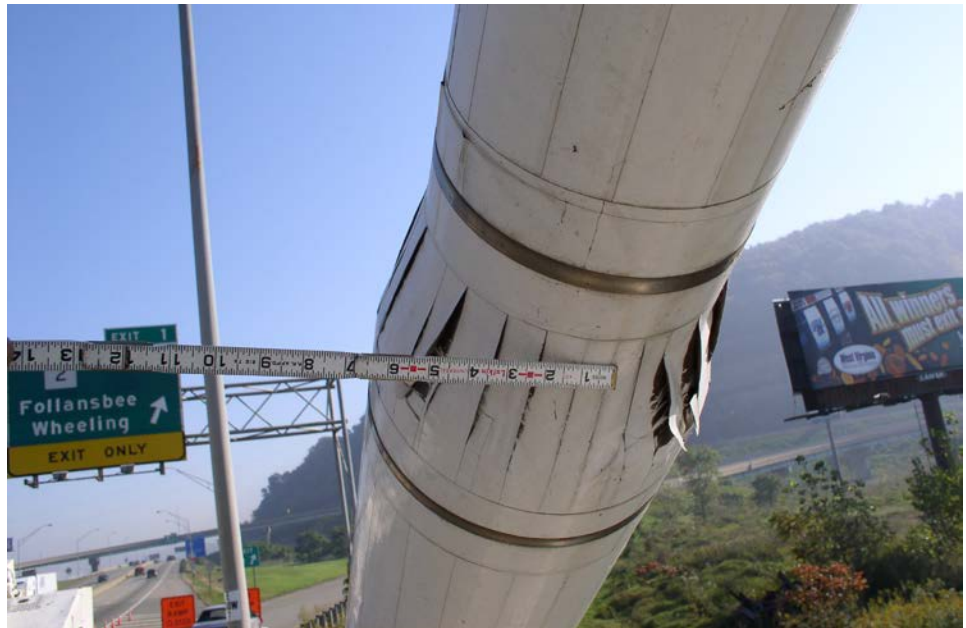
Figure 16.1.43 Deformed Cable Wrapping
