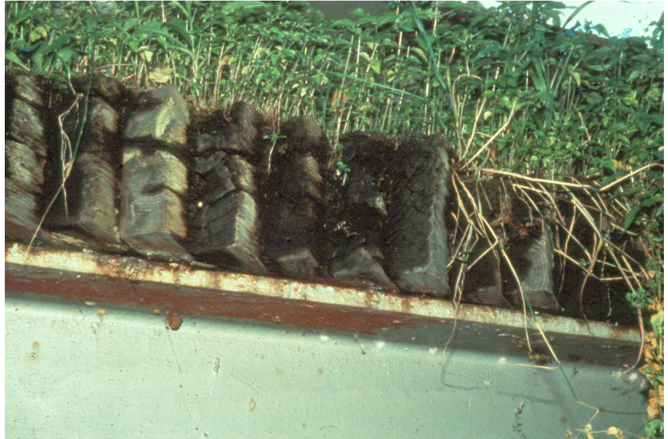
Figure 7.1.10 Edge of Deck Exposed to Drainage, Resulting in Plant Growth
