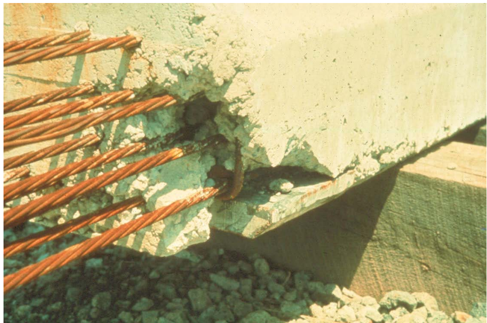
Figure 9.9.16 Spalling Due to Poor Concrete Placement
