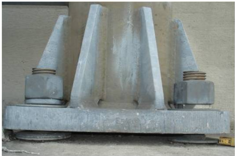
Figure 7.5.34 Sign Attachment Exhibiting Anchor Pullout
