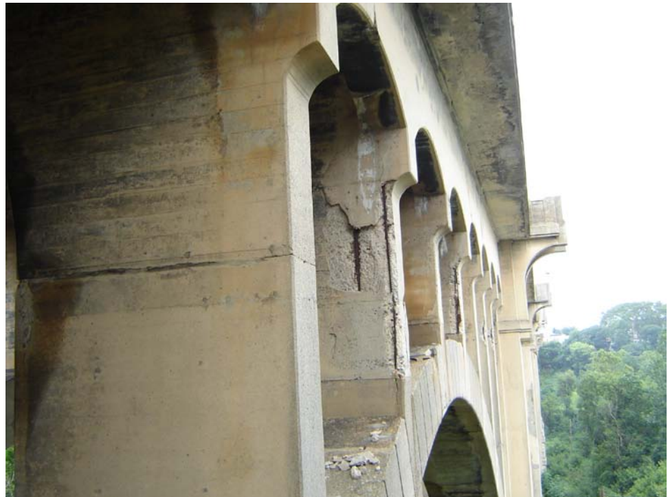
Figure 9.5.16 Severe Scaling and Spalling on a Spandrel Column
