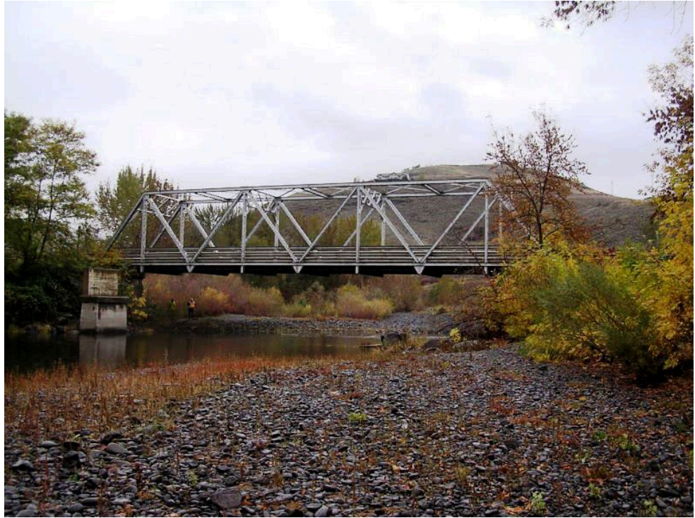
Figure 13.2.56 Stream Alignment Not Parallel with Abutments
