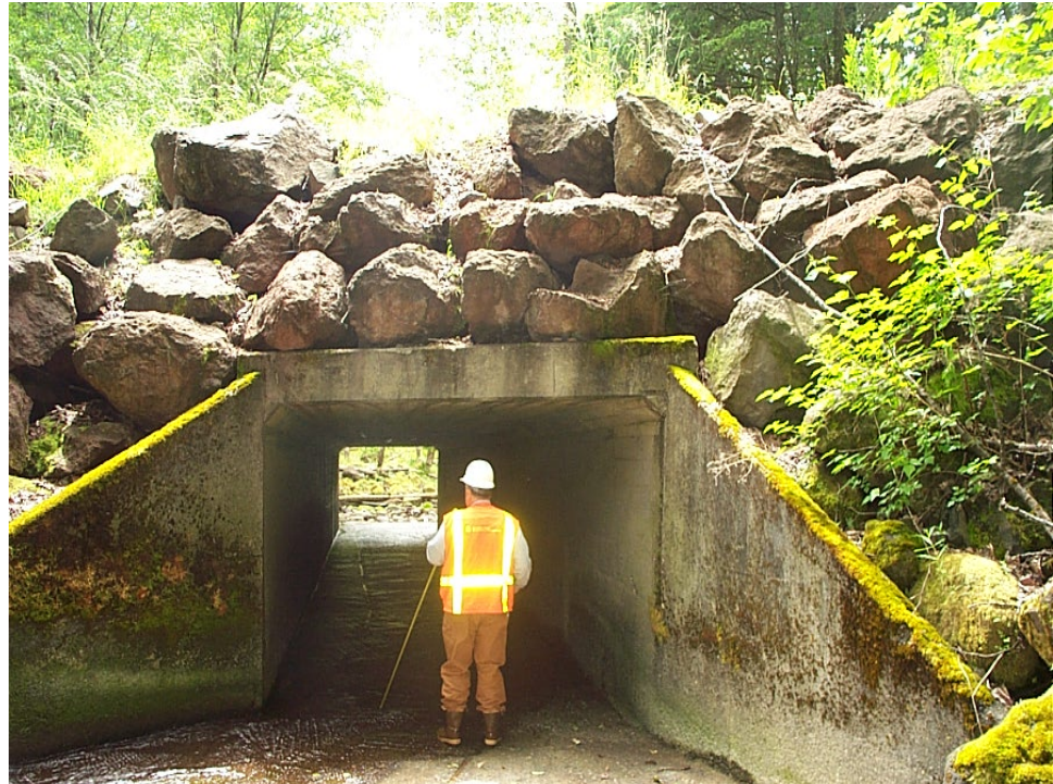
Figure 14.1.33 Potential for Tilted Wingwalls
