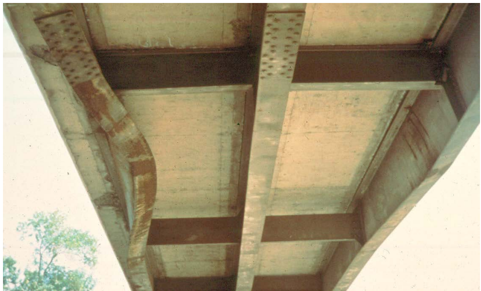
Figure 10.1.24 Collision Damage on a Fabricated Multi-Girder Bridge
