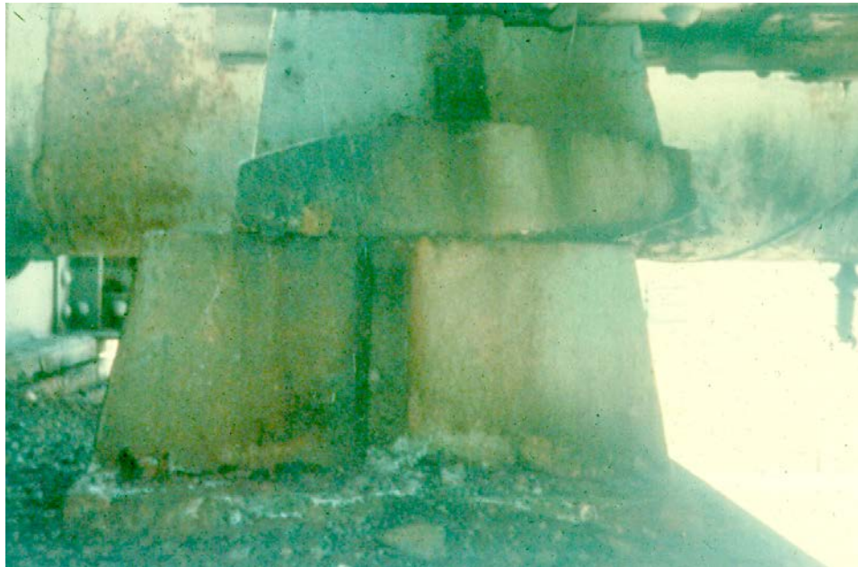
Figure 11.1.29 Rocker Bearing with Excessive Horizontal Movement
