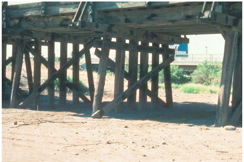
Figure 12.2.16 Timber Pile Bent
