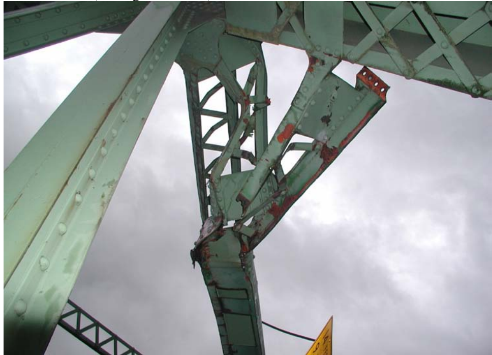
Figure 10.4.56 Collision Damage to Portal
