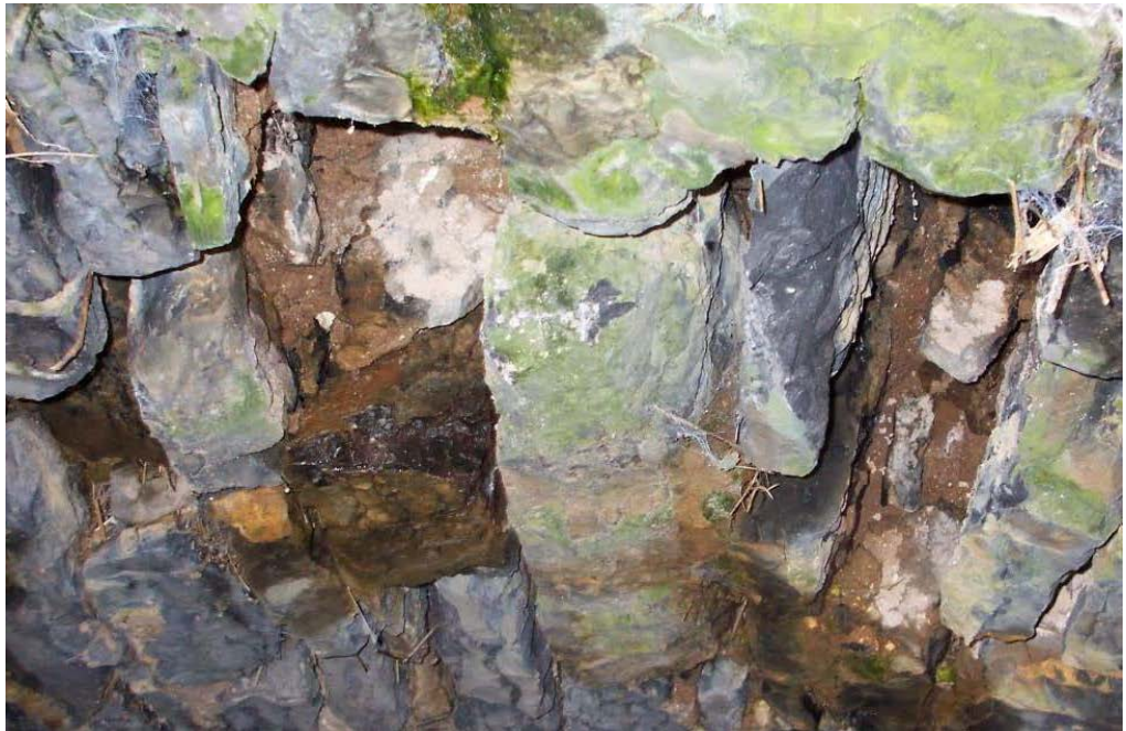
Figure 14.2.18 Missing Stones in Masonry Culvert
