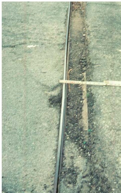
Figure 7.5.24 Debris Lodged in a Sliding Plate Joint
