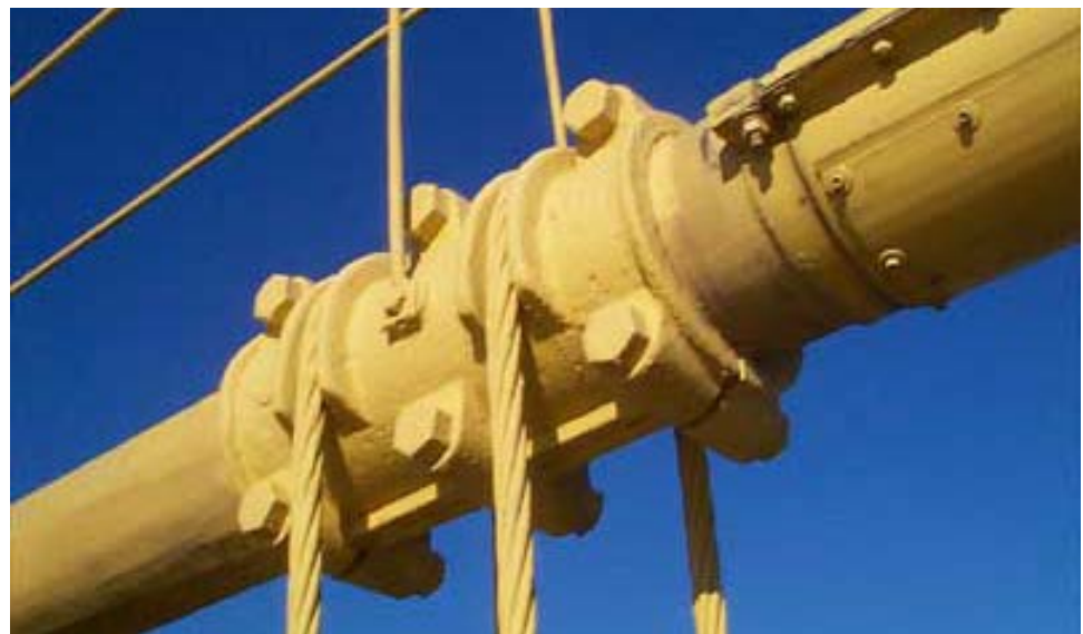
Figure 16.1.19 Grooved Cable Bands
