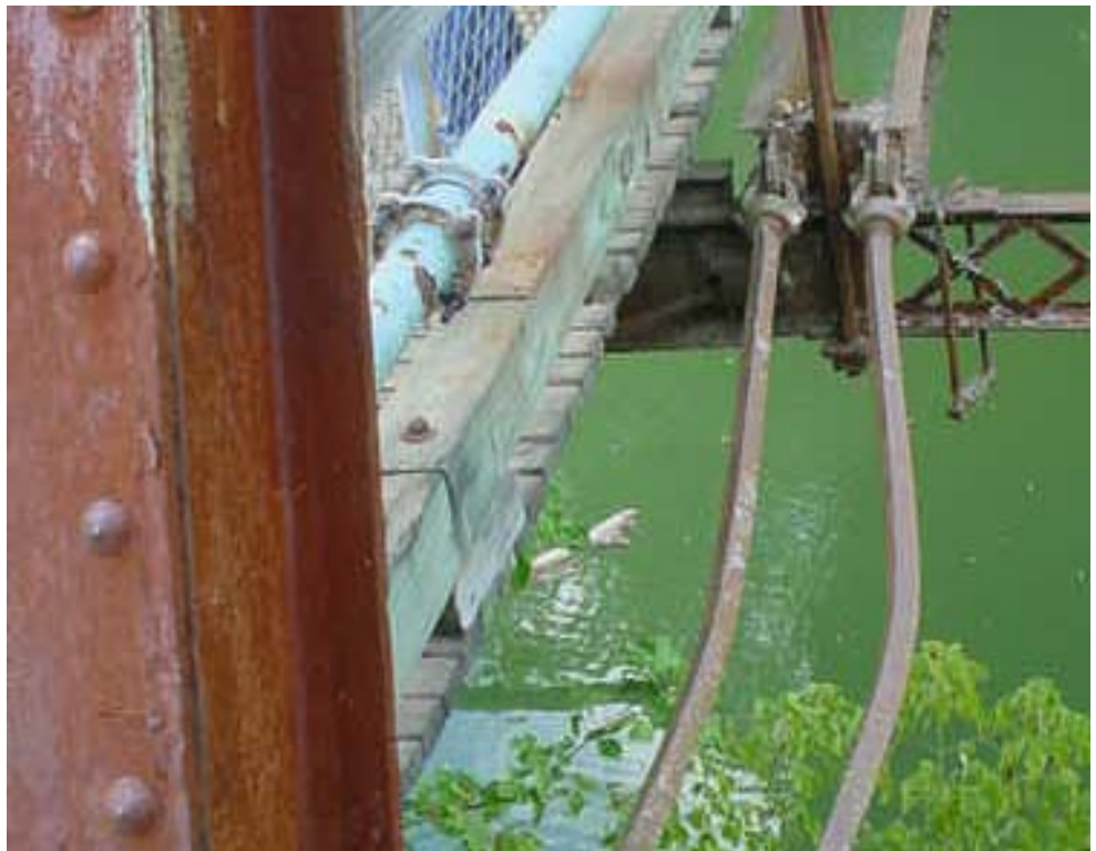
Figure 10.4.47 Bowed Bottom Chord Eyebar Member
