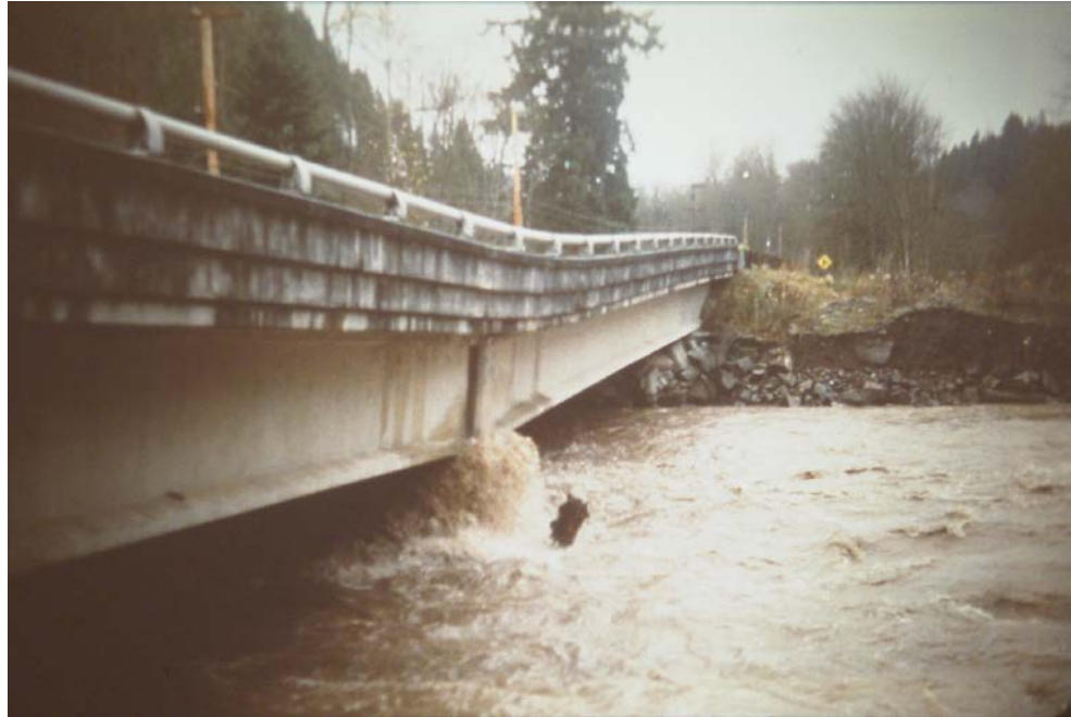
Figure 13.3.12 Movement of a Substructure Unit
