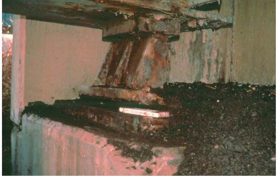
Figure 11.1.28 Heavy Corrosion on a Steel Rocker Bearing
