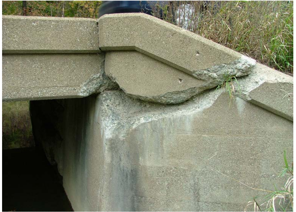
Figure 12.1.32 Spalled Concrete Wingwall
