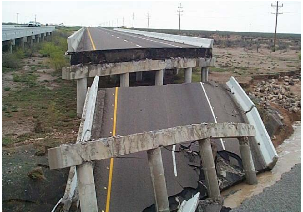
Figure 12.2.48 Pier Movement and Superstructure Damage due to Scour/Undermining
