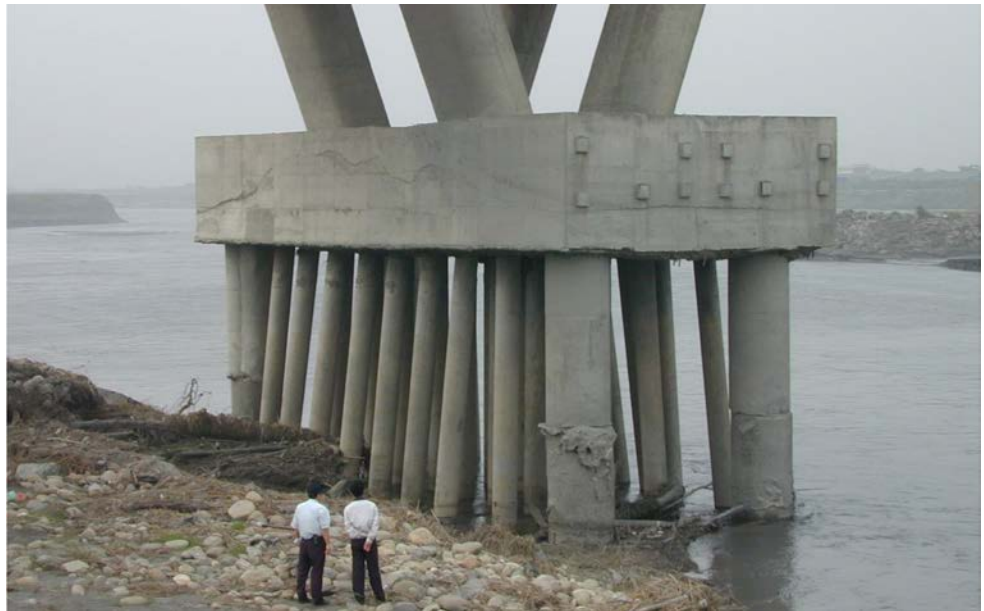
Figure 13.2.5 Close-up of General Scour of a Pier
