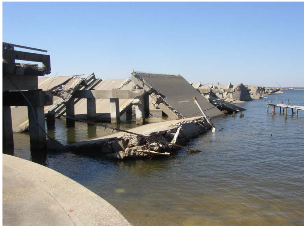
Figure 13.1.2 Failure Due to High Water Levels During Hurricane: Close-Up View
