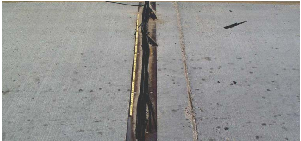
Figure 7.5.27 Failed Compression Seal
