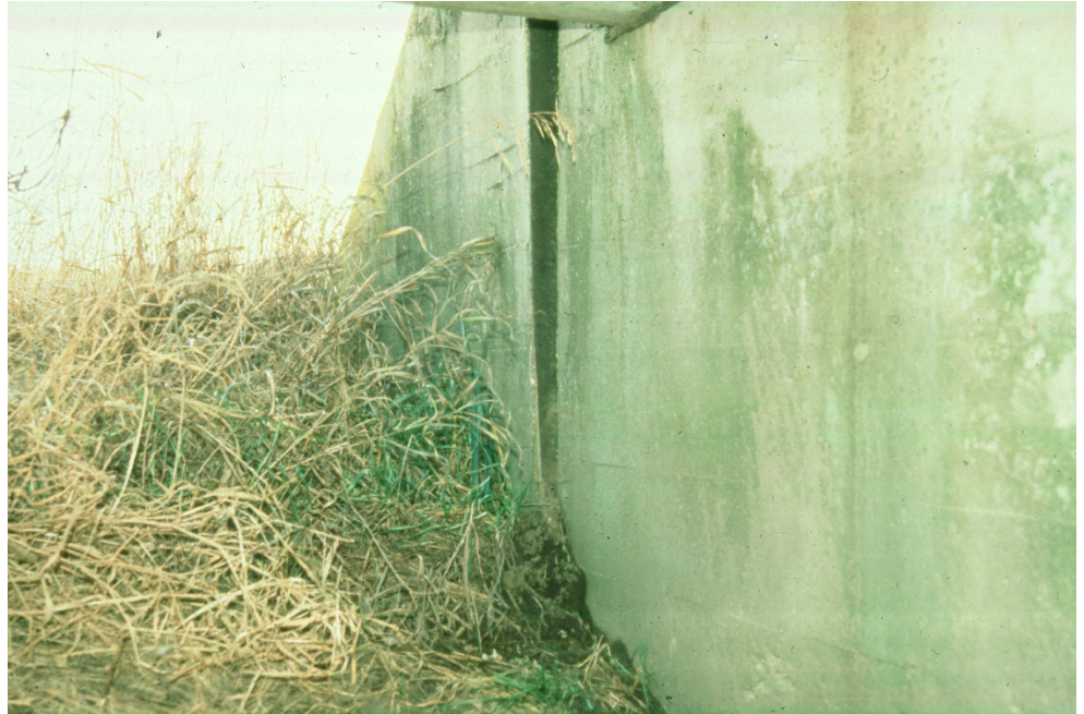
Figure 12.1.49 Rotational Movement at Concrete Wingwall
