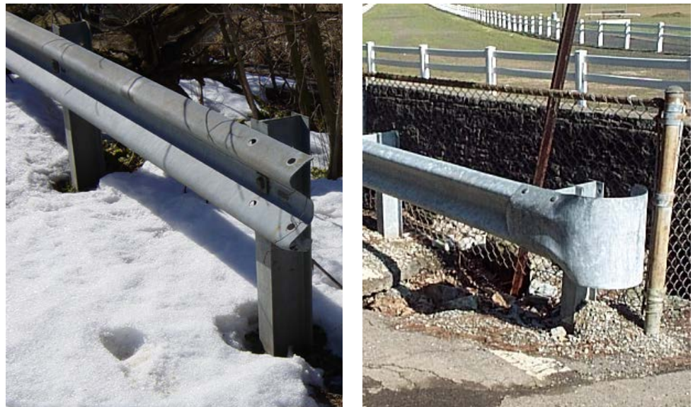
Figure 7.6.11 Unacceptable Blunt Ends
