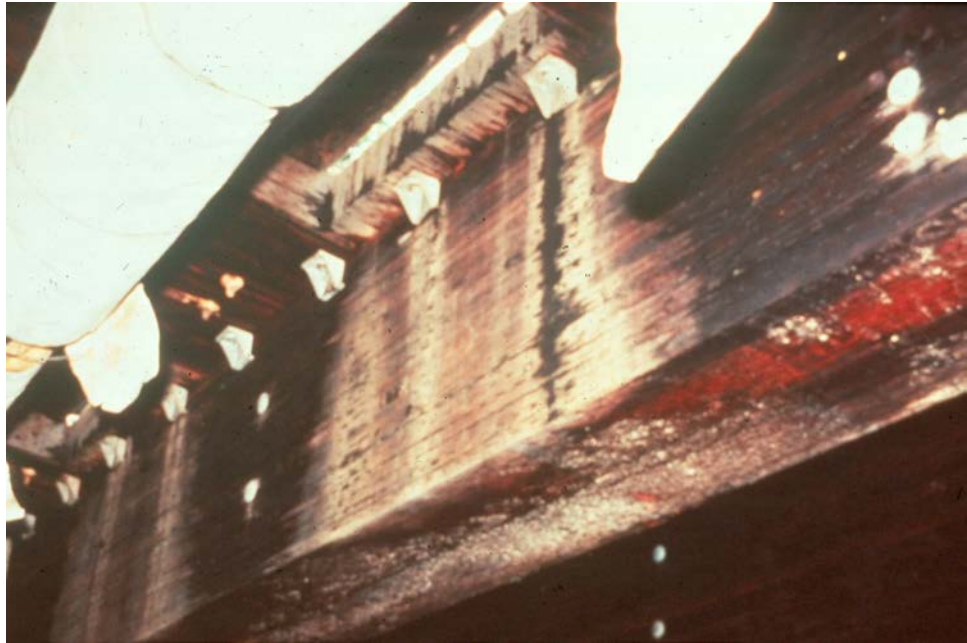
Figure 8.2.12 Decay on Glulam Beam
