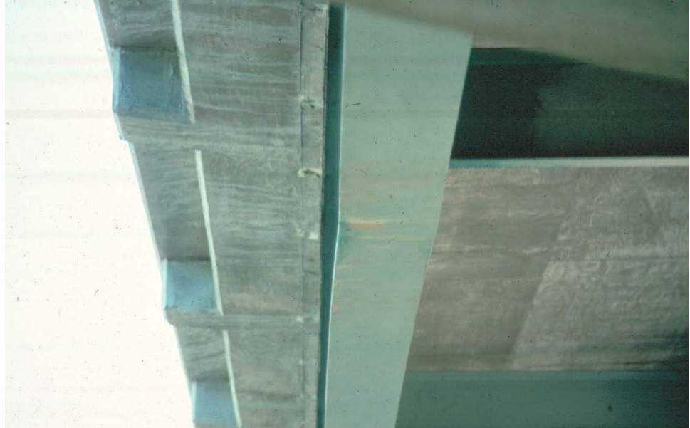
Figure 10.2.18 Collision Damage to a Deck Girder Bridge
