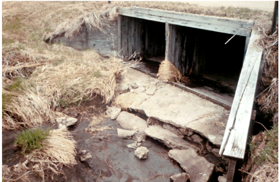
Figure 14.1.27 Scour and Undermining at Culvert Inlet
