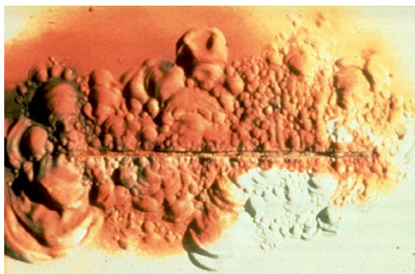
Figure 6.3.16 Rust Undercutting at Scratched Area
