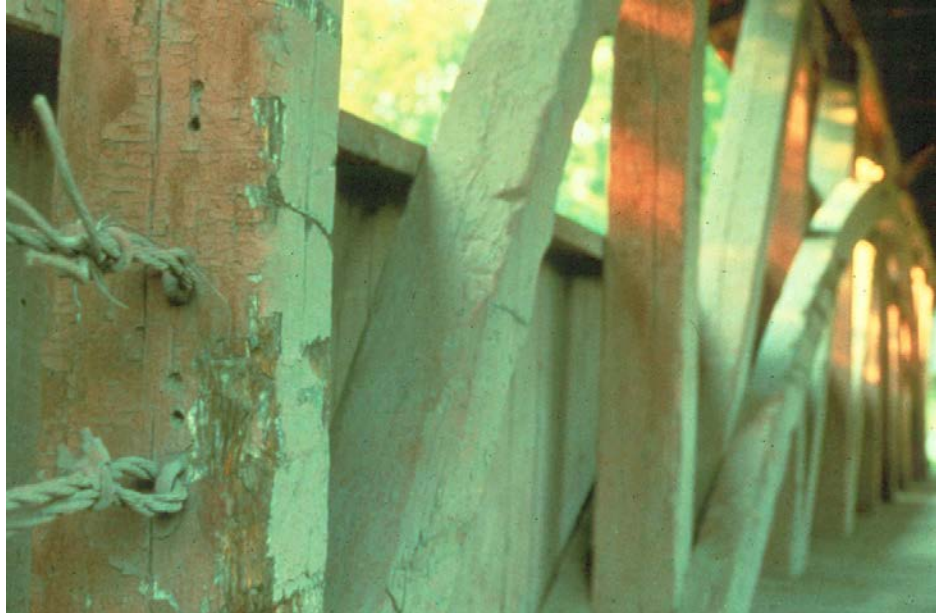
Figure 6.1.21 Impact/Collision Damage to a Timber Member
