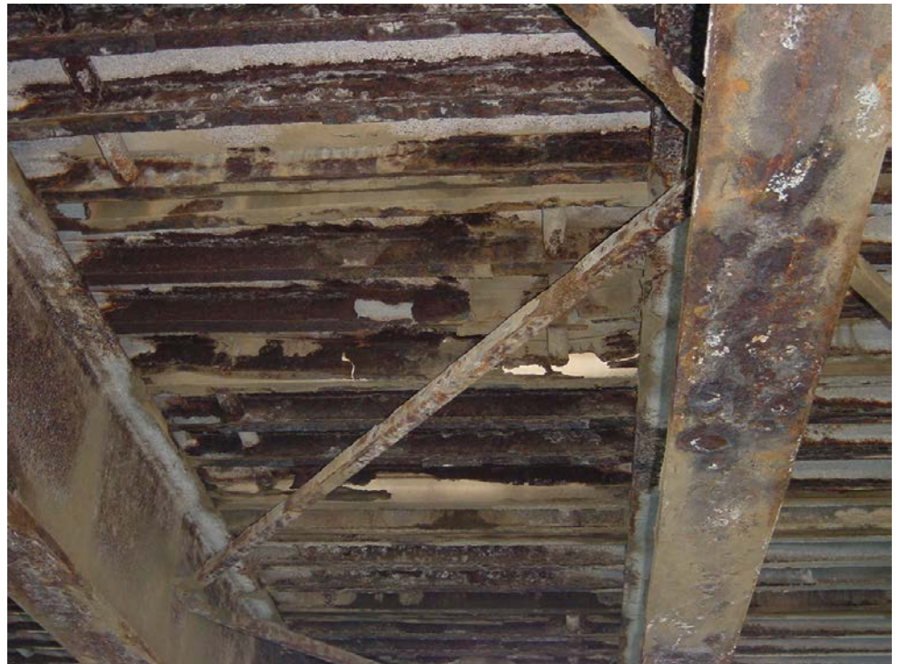
Figure 7.2.9 Deteriorated Stay-in-Place Form
