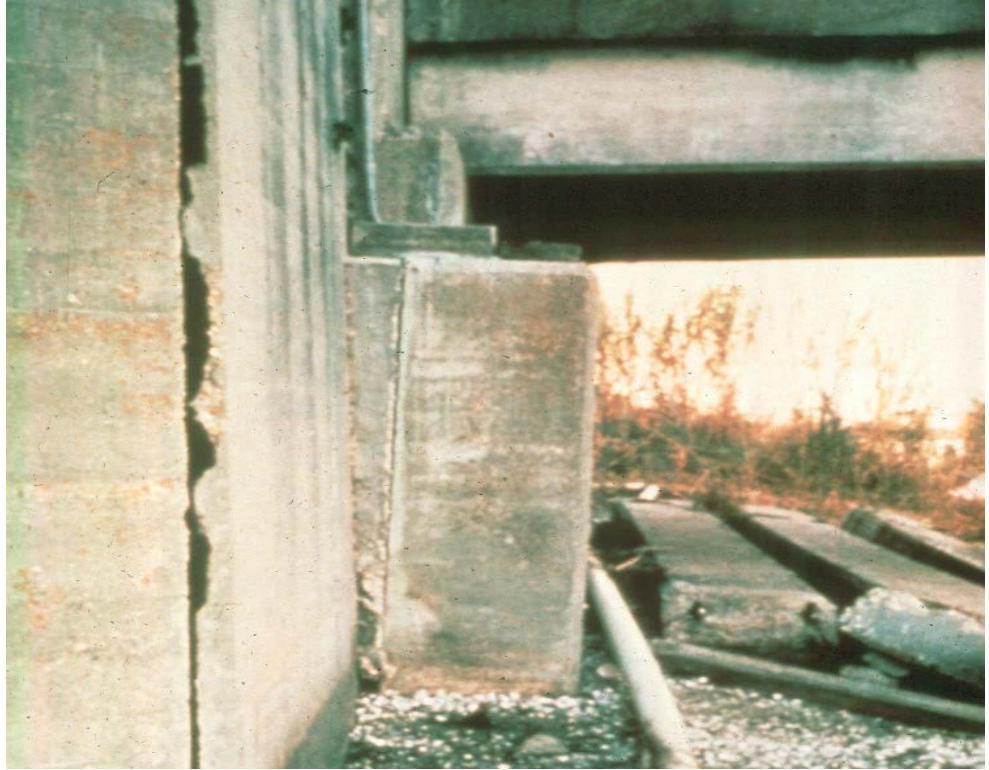
Figure 12.1.47 Rotational Movement at Abutment
