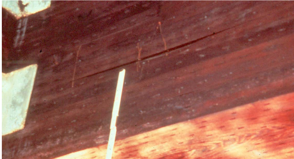
Figure 6.1.18 Delamination in a Glue Laminated Timber Member
