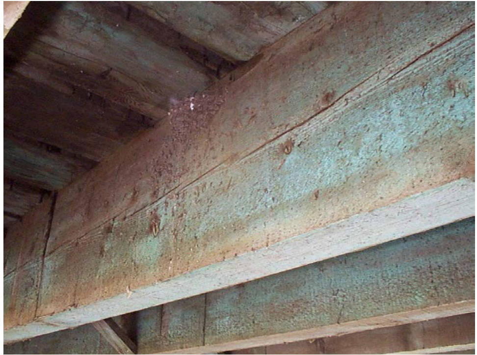
Figure 6.1.23 Horizontal Shear Failure in Timber Member
