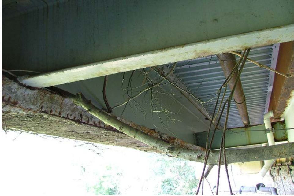
Figure 13.2.38 Drift Lodged in a Superstructure
