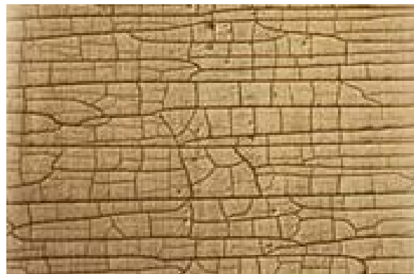
Figure 6.3.18 Paint Peeling from Steel Bridge Members
