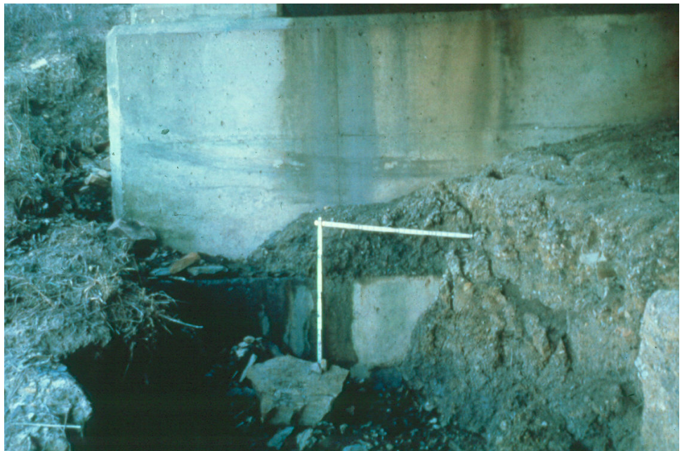
Figure 12.1.45 Erosion at Abutment Exposing Footing
