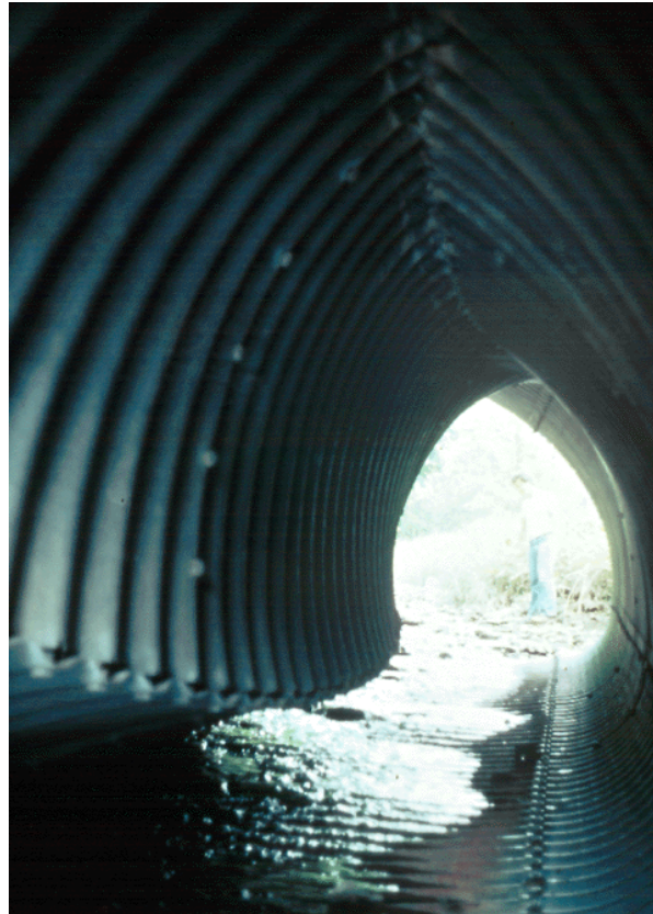
Figure 14.1.25 Bending or Shear Failure
