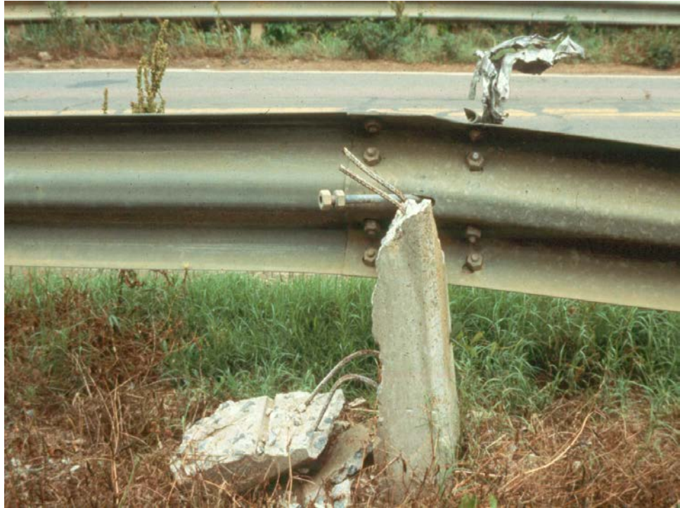
Figure 7.6.13 Approach Guardrail Collision Damage
