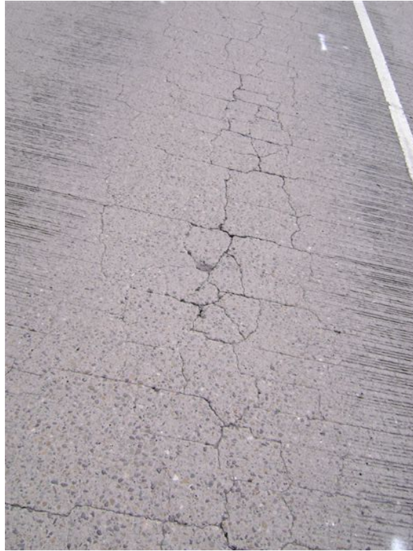
Figure 6.2.19 Pattern or Map Cracks
