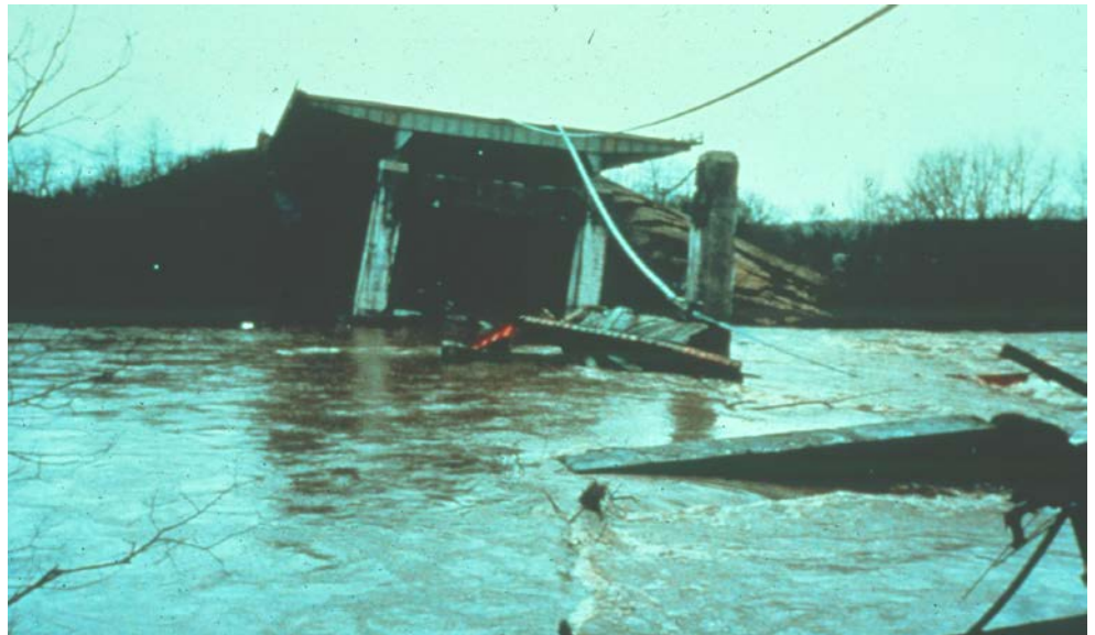
Figure 13.3.1 Schoharie Creek Bridge Failure
