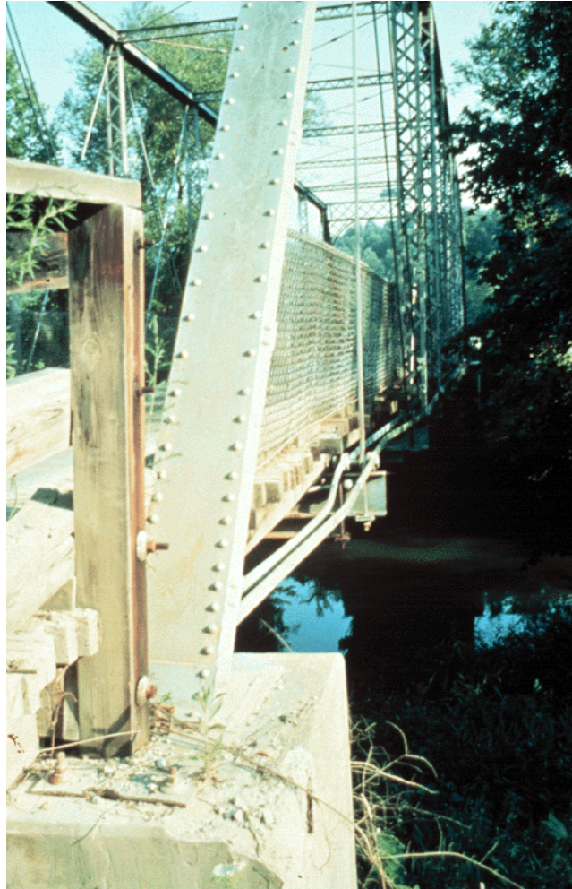
Figure 10.9.22 Buckled Eyebar due to Abutment Movement
