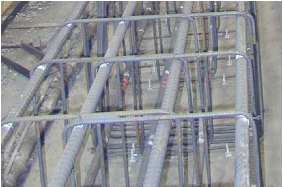
Figure 6.3.5 Steel Reinforcement Bars
