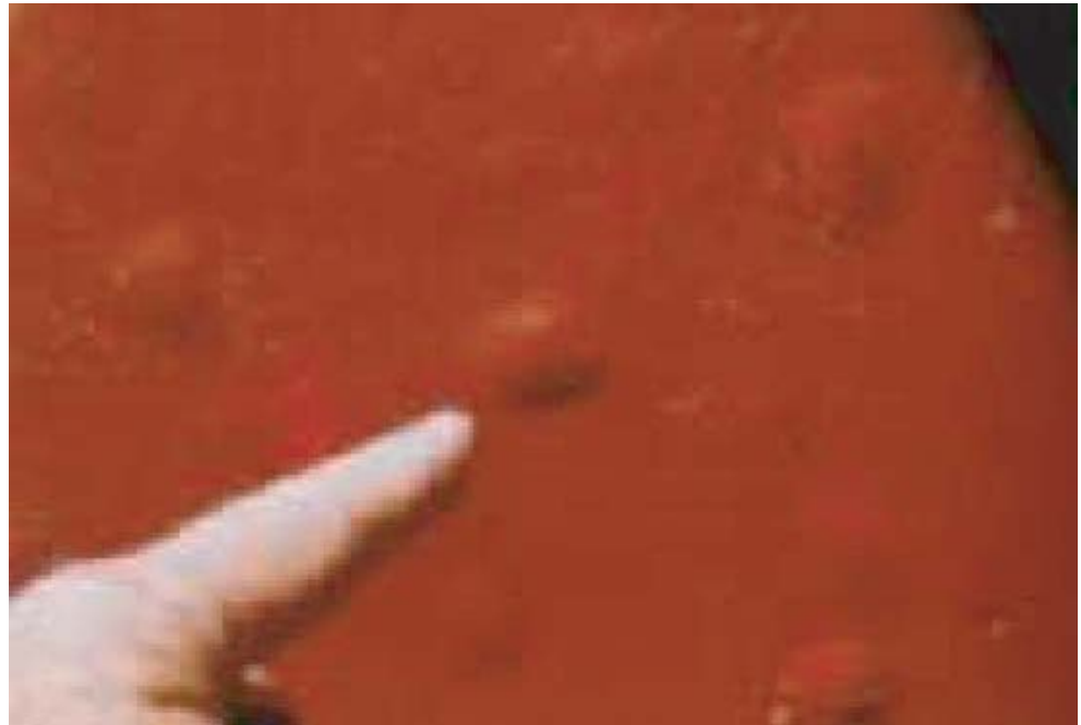
Figure 6.6.14 Blistering on a Laminated Surface
