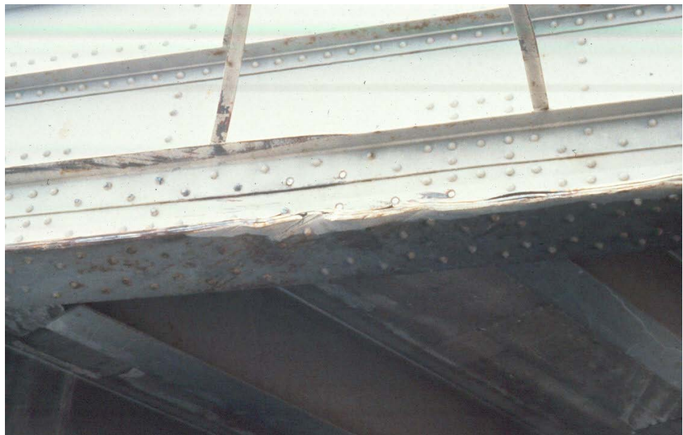
Figure 10.2.19 Collision Damage to a Through Girder Bridge
