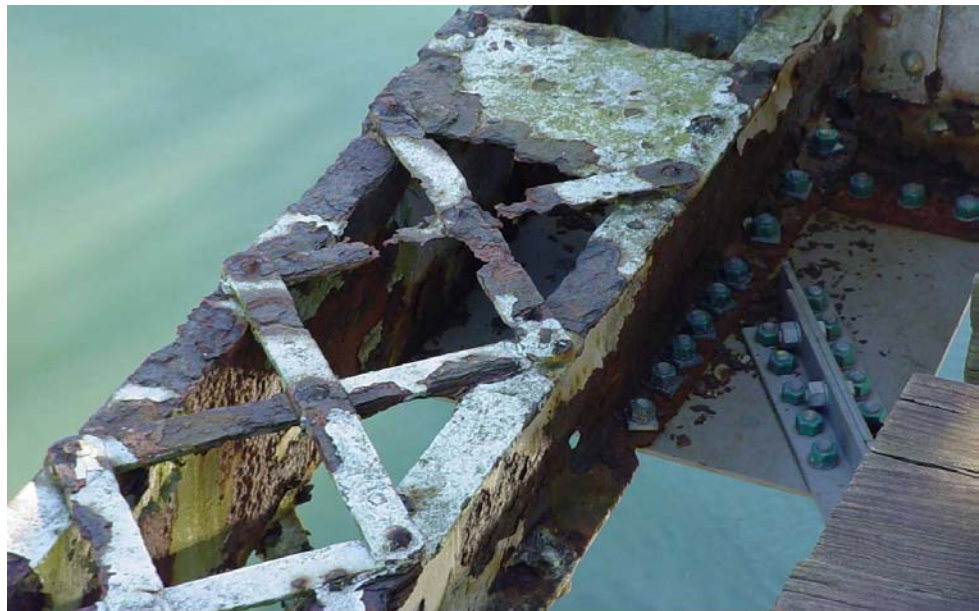
Figure 10.4.41 Corrosion and Section Loss on Truss Bottom Chord
