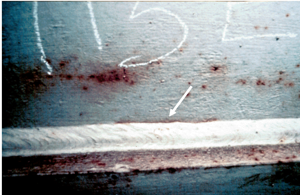
Figure 6.4.33 Part-Through Crack at a Cover Plated Flange Stage 1
