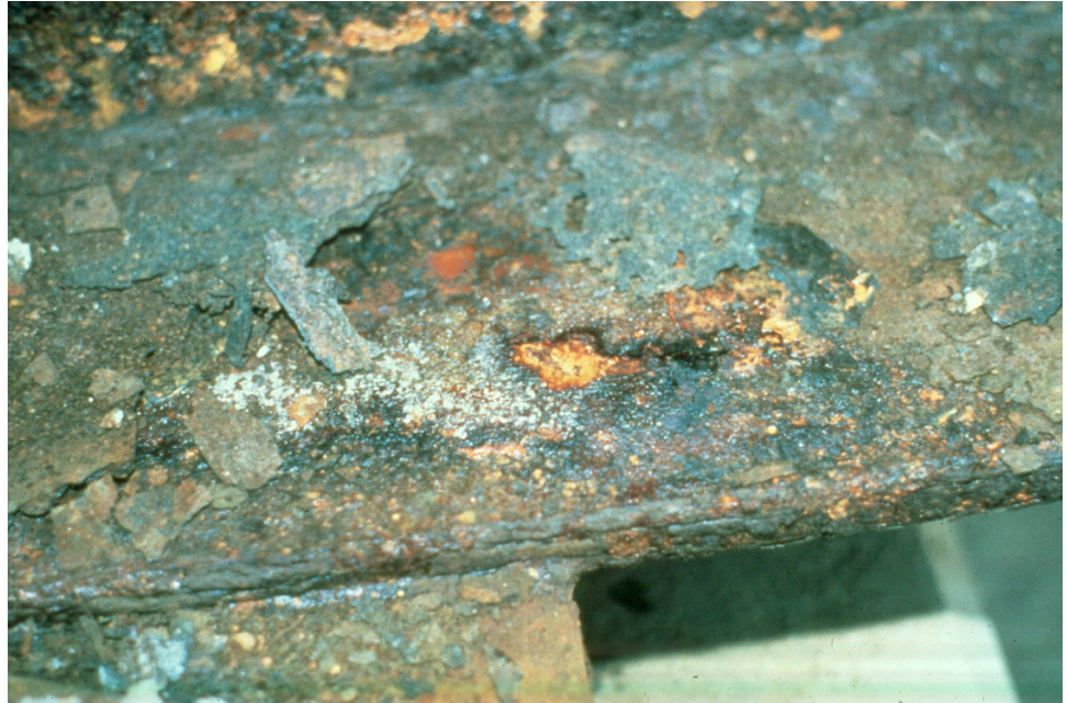
Figure 6.3.26 Color of Oxide Film is Critical in the Inspection of Weathering Steel; Dark Black Color in an Indication of Non-protective Oxide
