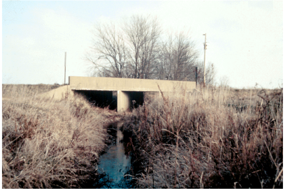
Figure 13.2.9 Vegetation Constricting the Waterway
