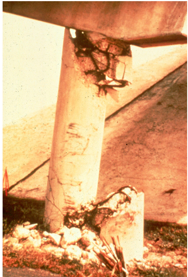
Figure 6.2.28 Concrete Column Collision Damage
