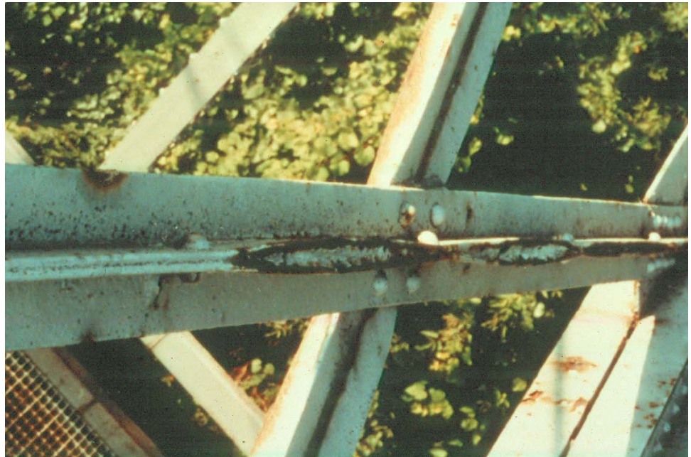
Figure 10.4.58 Sway Bracing with Pack Rust
