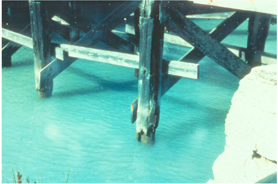
Figure 6.1.15 Marine Borer Damage to Wood Piling
