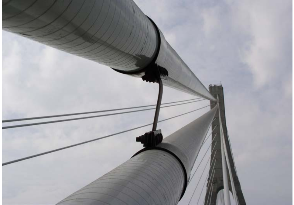
Figure 16.1.50 Cable Tie Type Damper System
