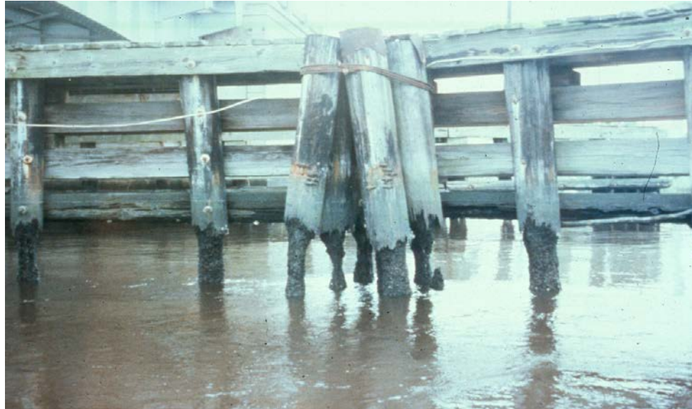
Figure 13.3.21 Damaged Protective System
