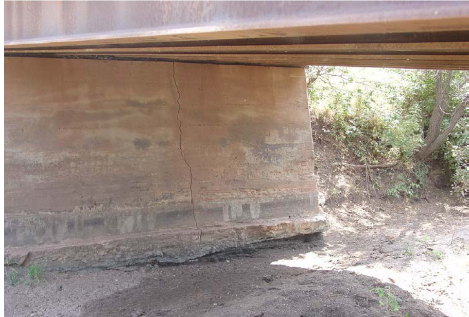
Figure 12.1.41 Crack in Abutment due to Settlement
