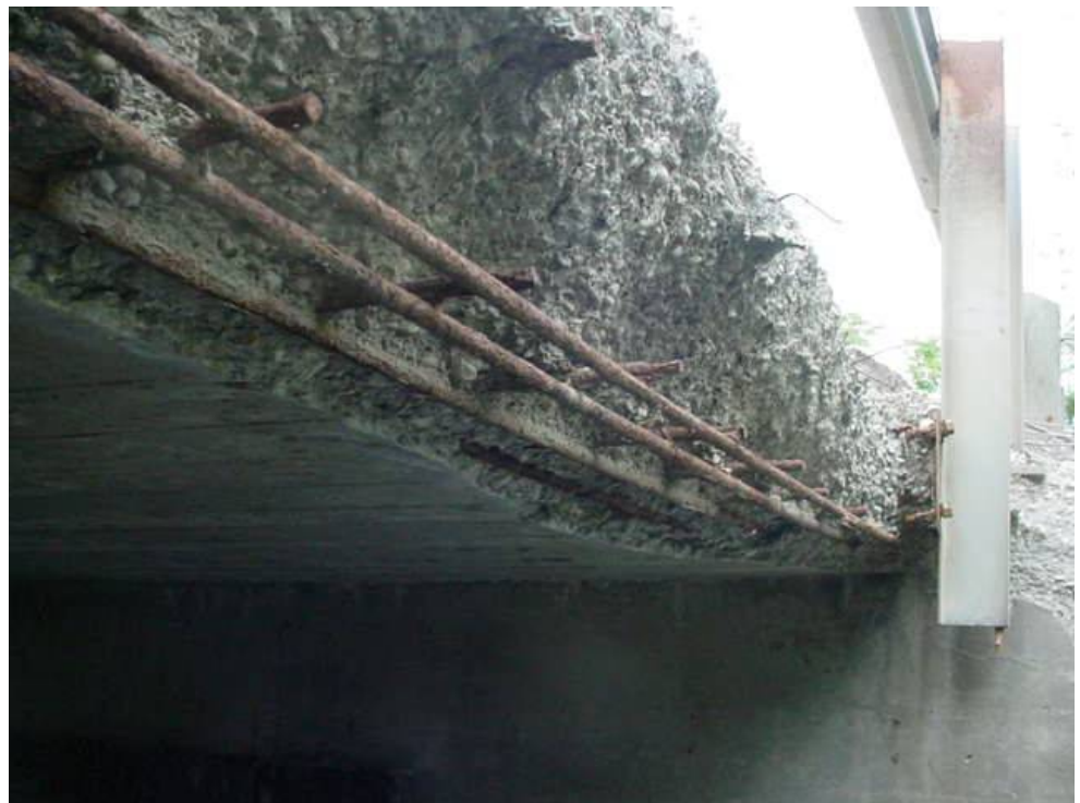
Figure 6.2.31 Loss of Bond: Concrete / Corroded Reinforcing Bar
