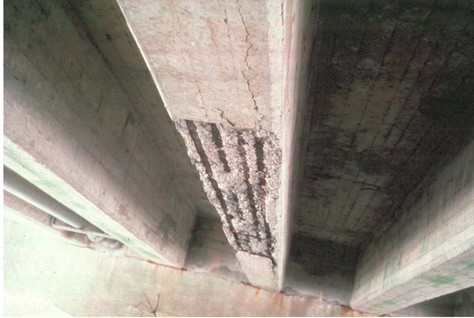
Figure 9.2.16 Spall on the Bottom of the Stem of a Tee Beam with Corroded Main Steel Exposed
