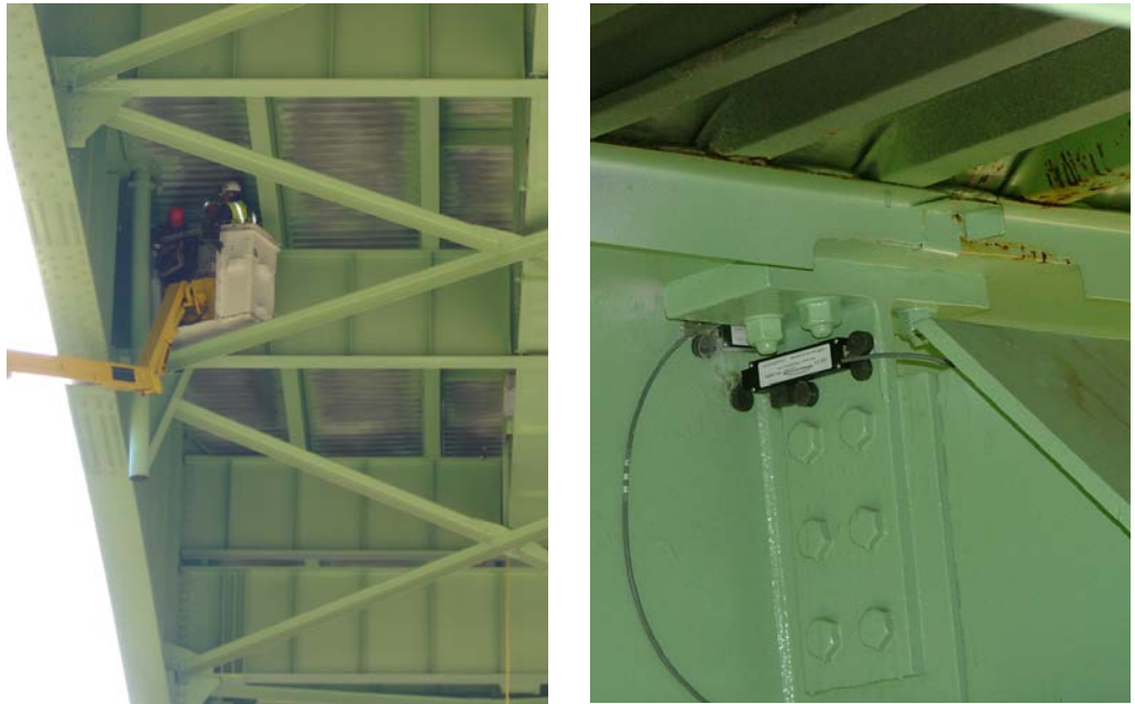
Figure 15.4.1 Installation of Sensors
