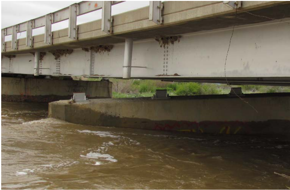
Figure 13.3.10 Flood Conditions: Pier Settlement.
