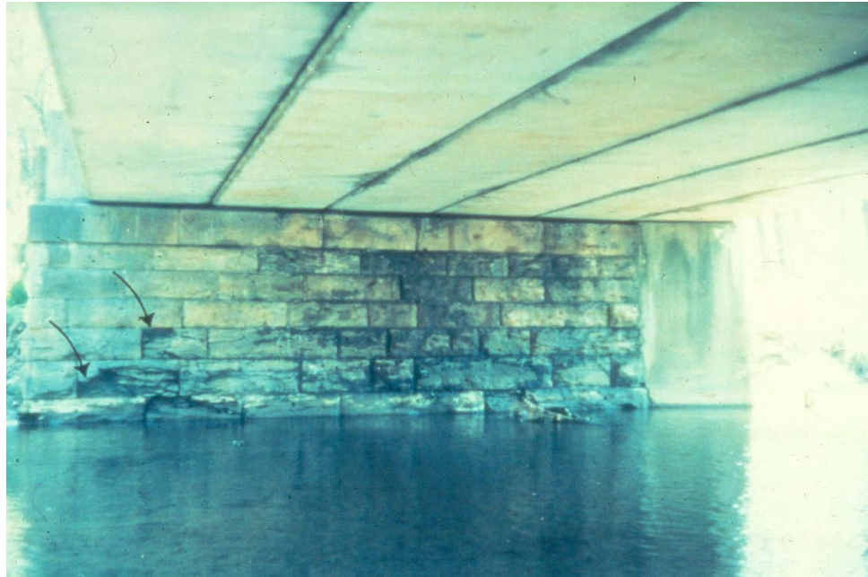
Figure 12.2.34 Deteriorated and Missing Stone at Masonry Pier
