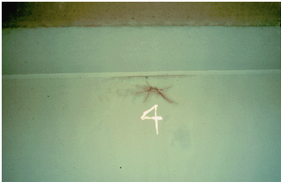
Figure 6.4.41 Through Crack in the Web
