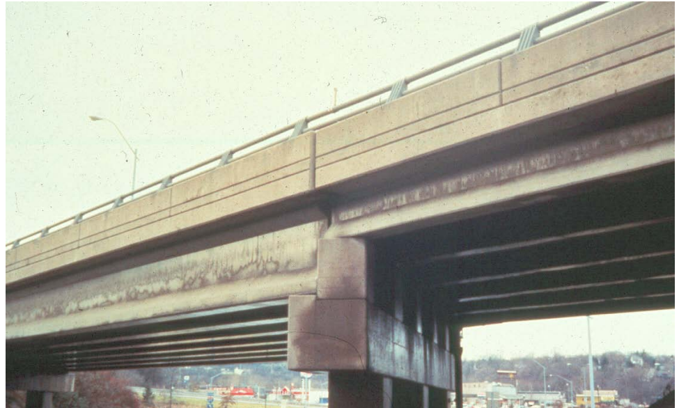
Figure 9.9.19 Leakage of Water at Joint between Spans
