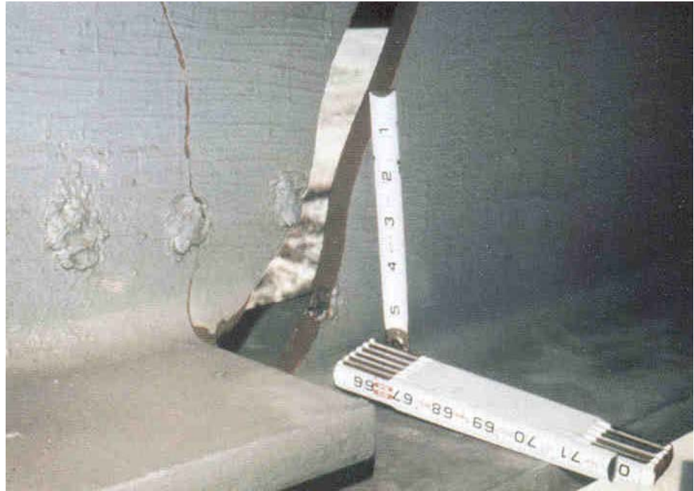
Figure 6.4.24 Crack Resulting from Plug Welded Holes
