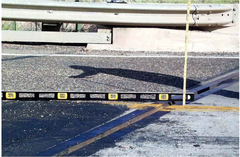
Figure 12.1.44 Vertical Misalignment Between Approach Slab (left) and Bridge Deck (right)
