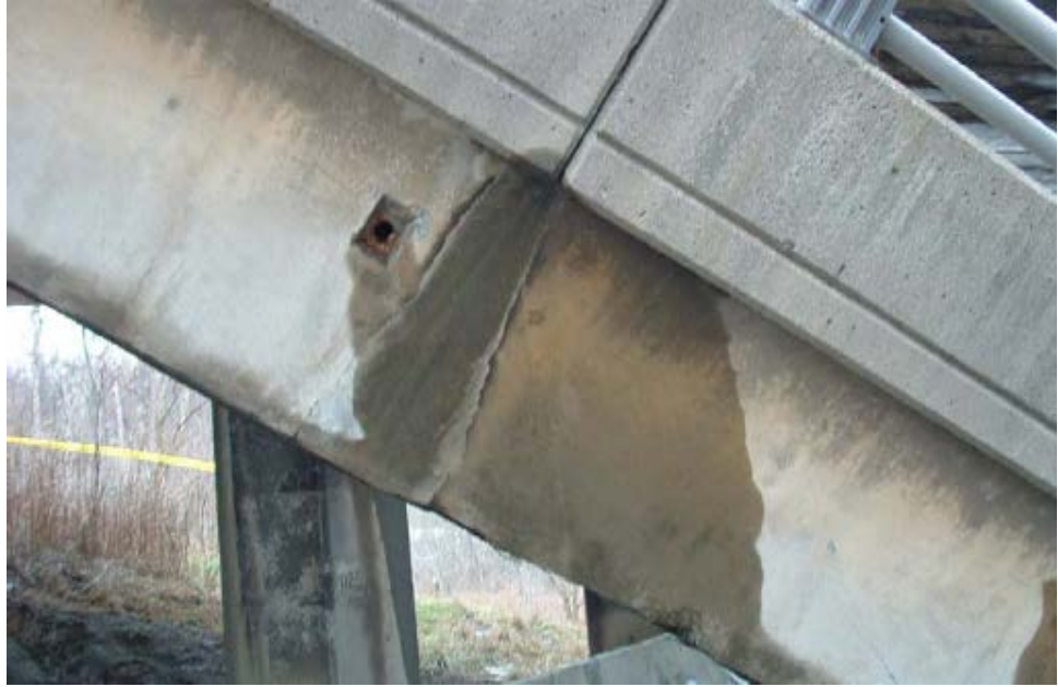
Figure 9.10. 29 Water Leakage Through Parapet Deflection Joints
