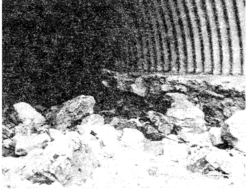
Figure 14.3.20(Exhibit 78) Erosion of Invert Undermining footing of Arch
