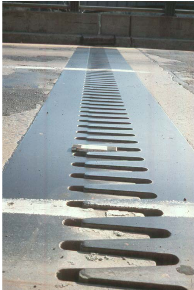
Figure 7.5.26 Improper Vertical Alignment at a Finger Plate Joint
