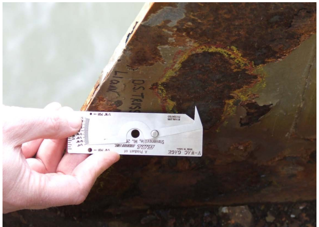
Figure 10.8.22 V-WAC Gage and Inspector Using the V-WAC in the Field to Measure the Section Loss of the Gusset Plate
