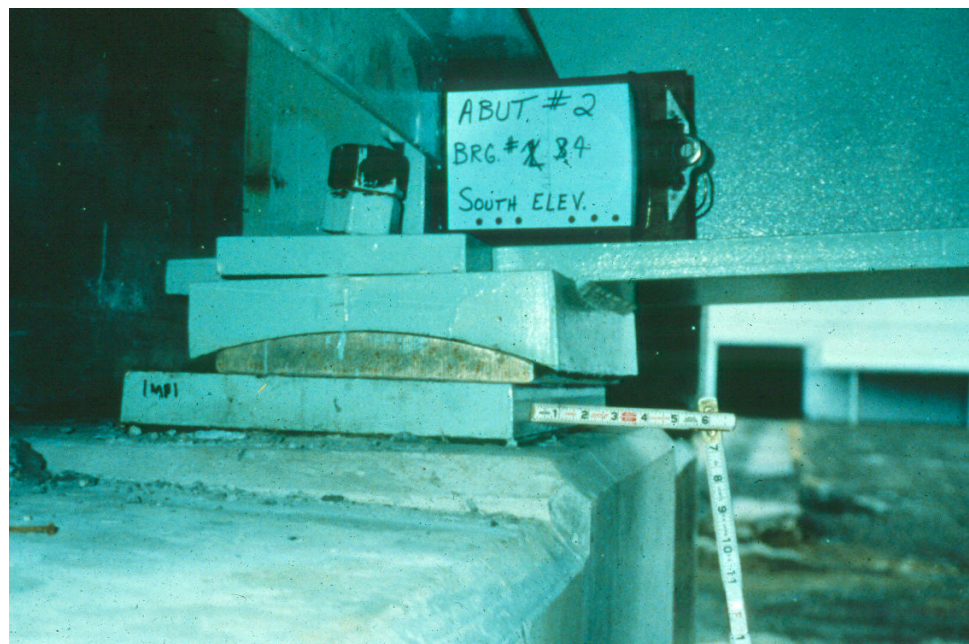
Figure 11.1.32 Longitudinal Misalignment in Bronze Sliding Plate Bearing
