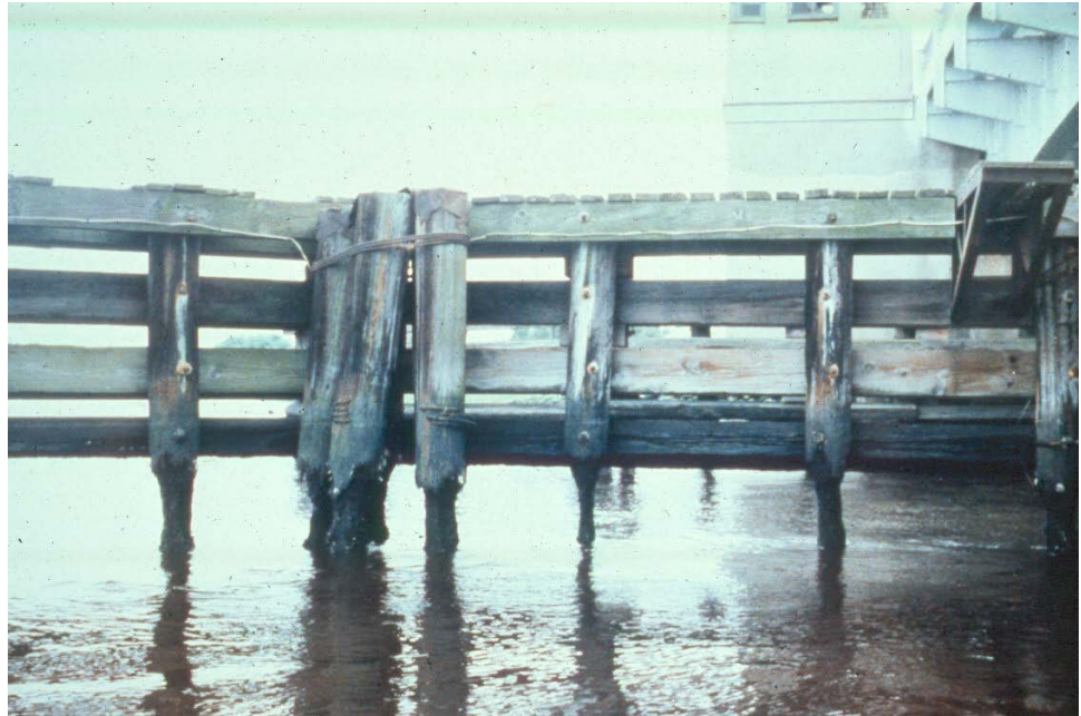
Figure 12.2.54 Timber Fender System with Deteriorated Piles
