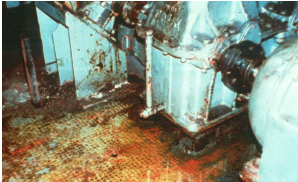
Figure 16.2.61 Cracked Speed Reducer Housing
