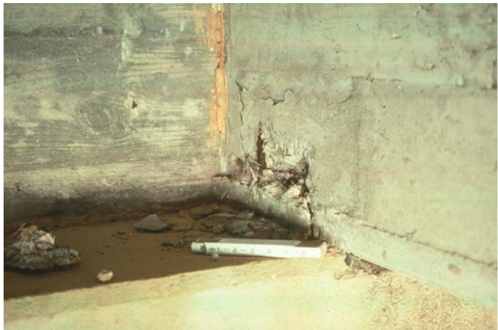
Figure 9.2.10 Deteriorated Tee Beam Bearing Area
