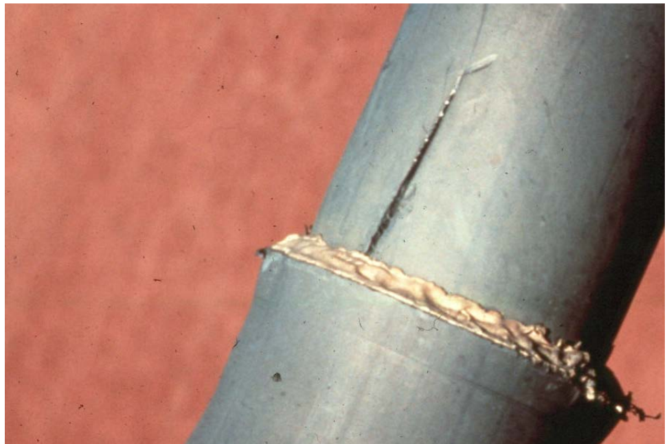
Figure 16.1.47 Splitting of Cable Sheathing
