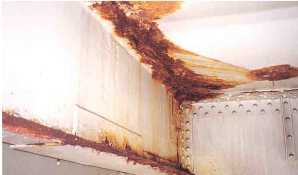
Figure 6.4.53 Field Welds Perpendicular to Bending Stresses are Susceptible to Cracking
