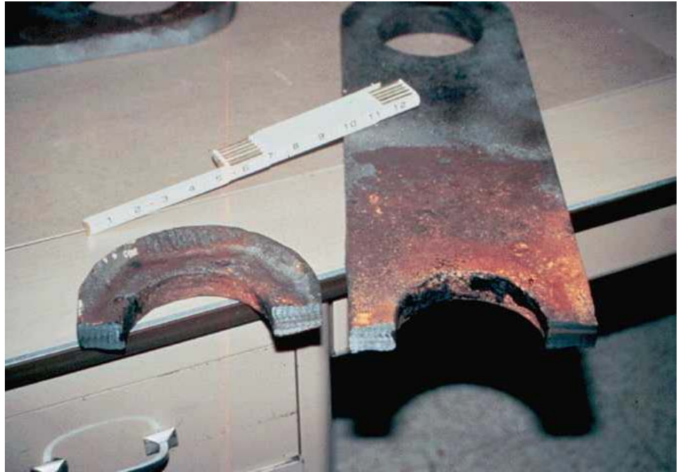
Figure 10.7.21 Corroded Hanger Plate
