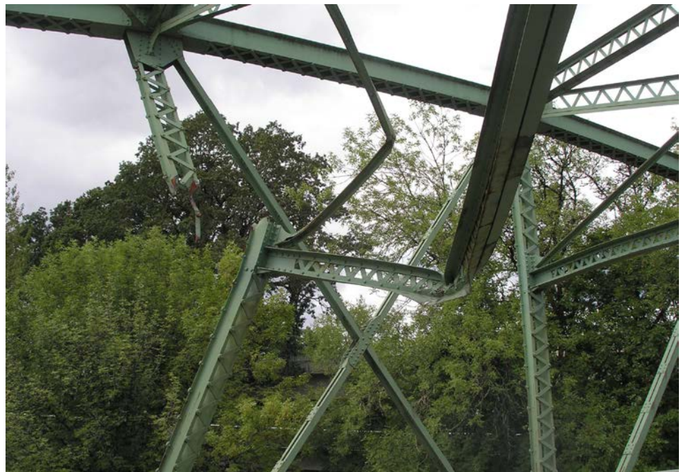
Figure 6.3.13 Collision Damage on a Steel Bridge
