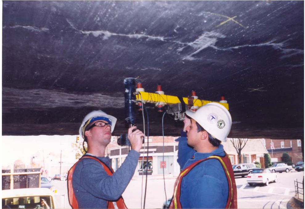
Figure 15.2.1 Portable Hand Held Sonic/Ultrasonic Testing Sensor Array System
