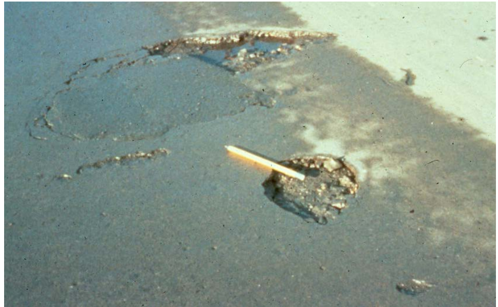
Figure 6.2.24 Spalling on a Concrete Deck
