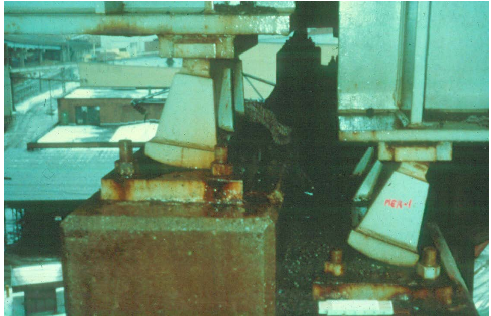
Figure 11.1.42 Serious Bearing Condition
