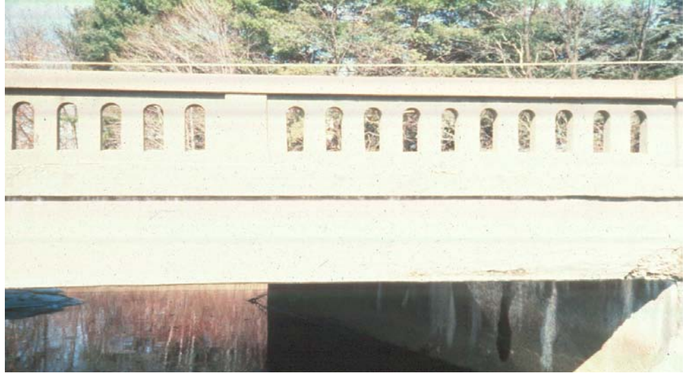
Figure 9.2.19 Deteriorated Tee Beam End Due to Drainage
