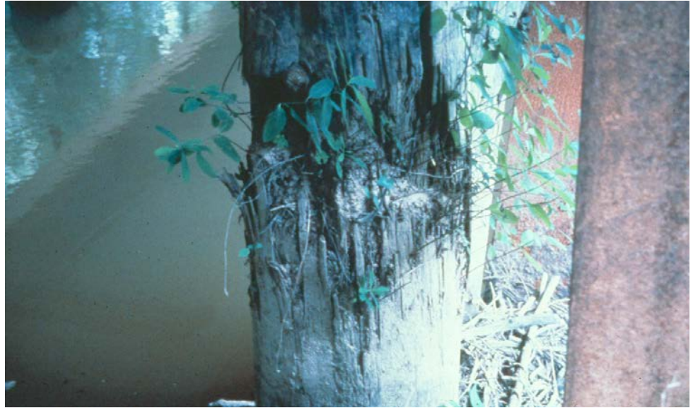
Figure 13.3.24 Deteriorated Timber Piling
