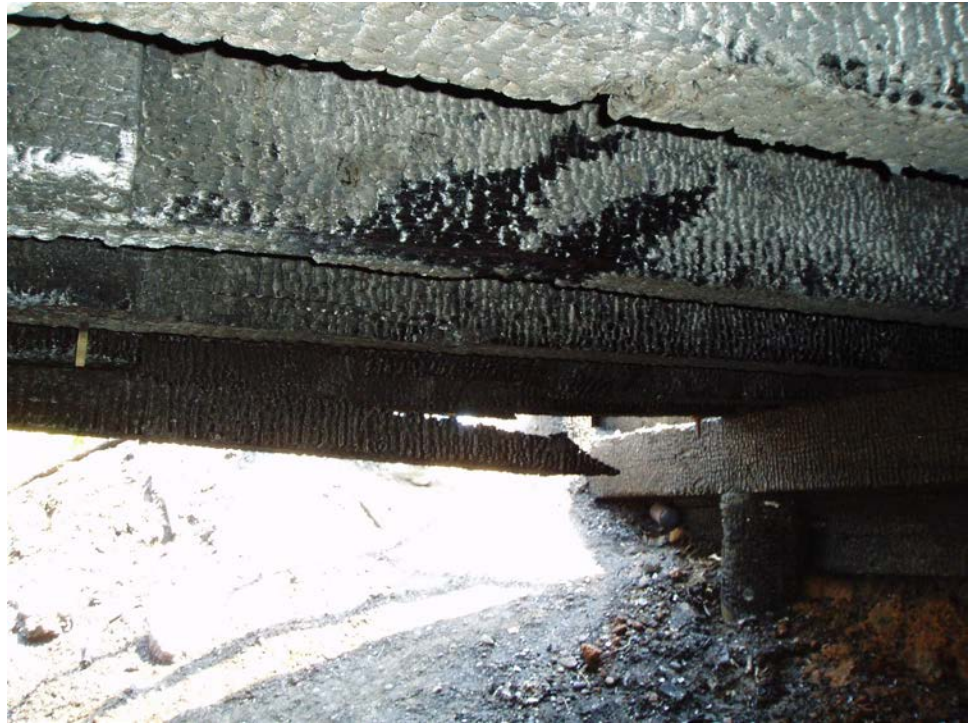
Figure 6.1.20 Fire Damaged Timber Members
