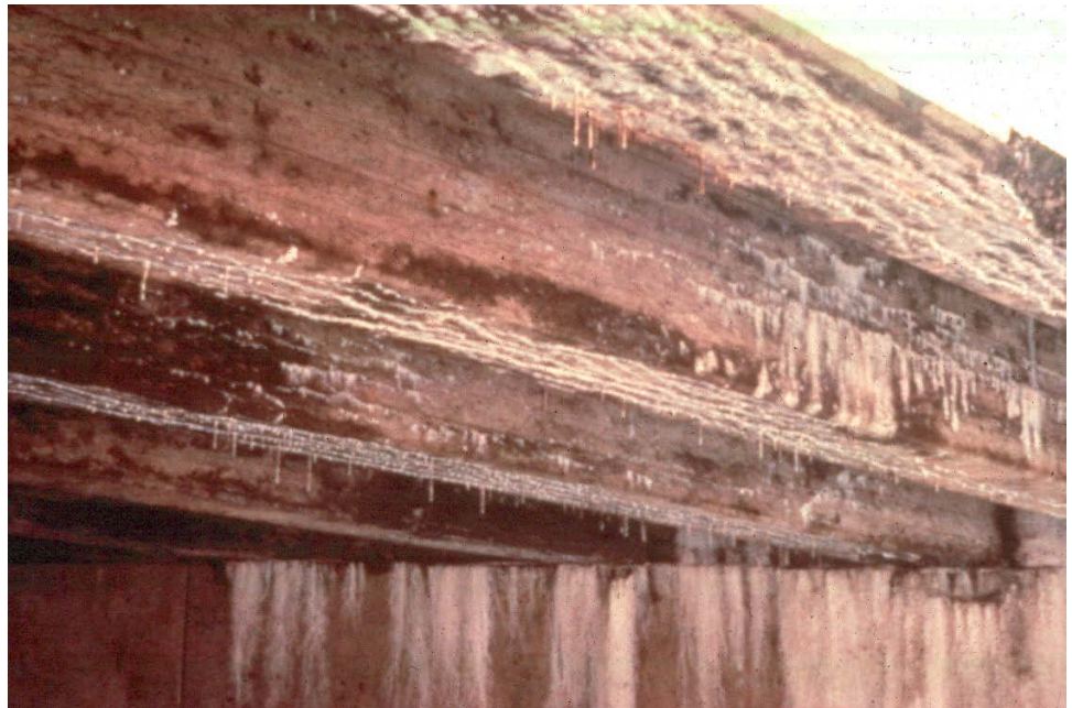
Figure 9.2.15 Stem of a Cast-in-Place Concrete Tee Beam with Cracking and Efflorescence
