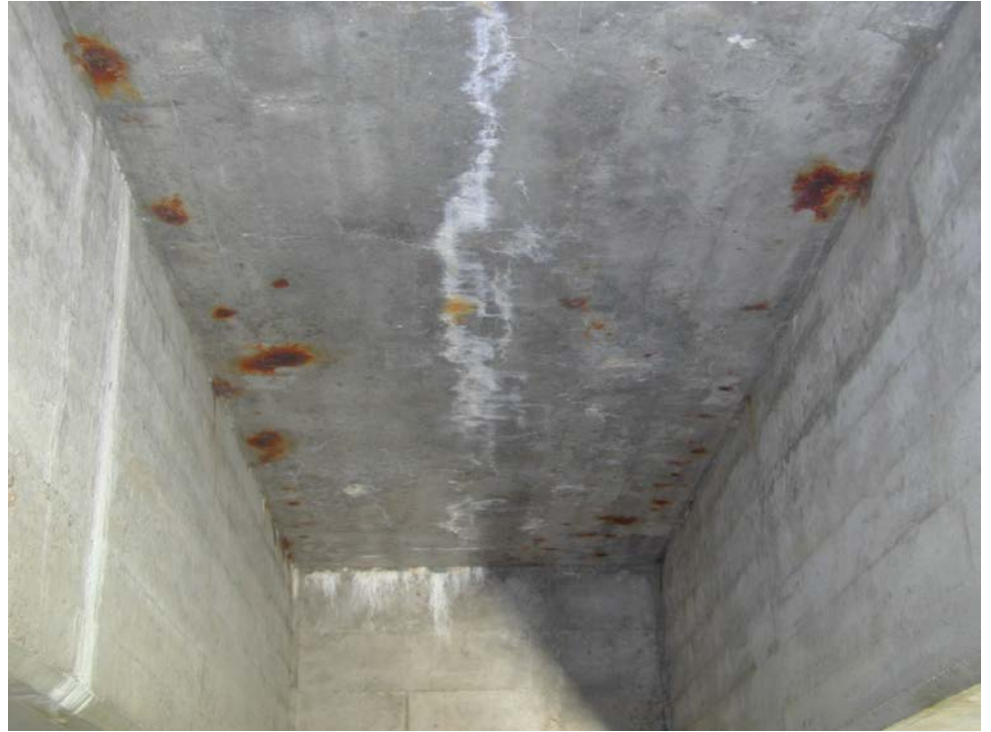
Figure 7.2.8 Underside View of Longitudinal Deck Crack
