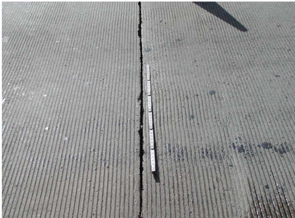
Figure 7.5.12 Open Expansion Joint
