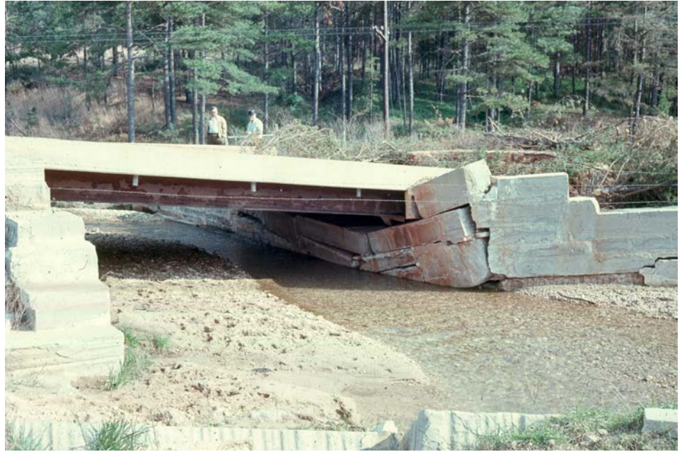
Figure 12.1.50 Abutment with Undermining due to Scour
