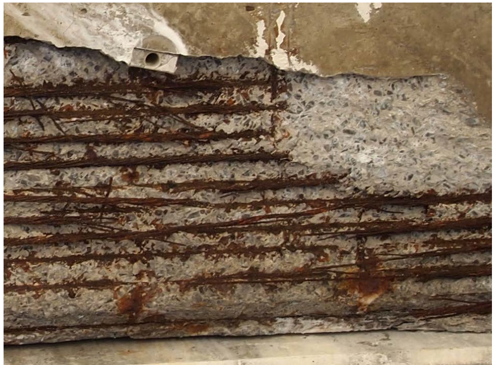
Figure 9.10.16 Close-up of Failed Strands due to Corrosion
