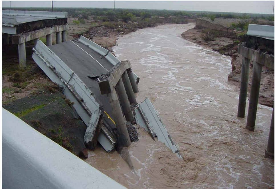
Figure 13.1.3 Pier Foundation Failure
