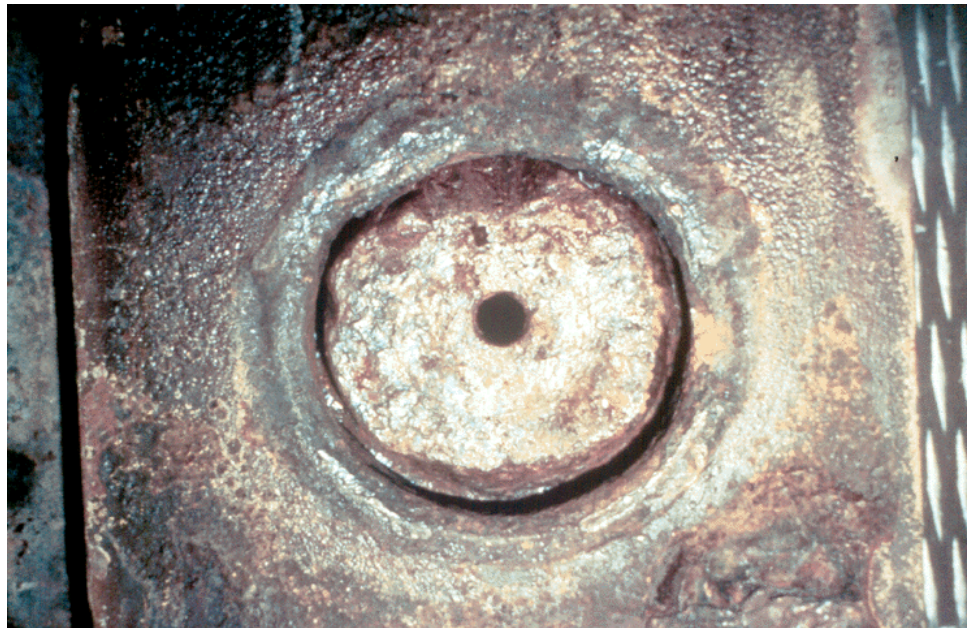
Figure 10.7.24 Corroded Pin-and-Hanger Assembly
