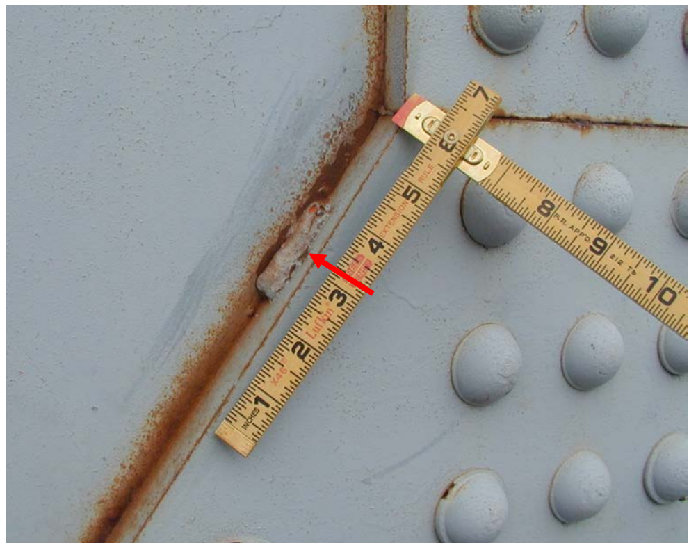
Figure 10.8.26 Partial Length Cracked Tack Weld
