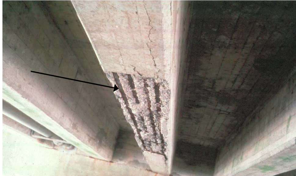
Figure 6.2.5 Concrete Member with Tensile Steel Reinforcement Showing
