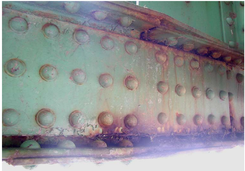
Figure 6.3.24 Corroding Rivet Head
