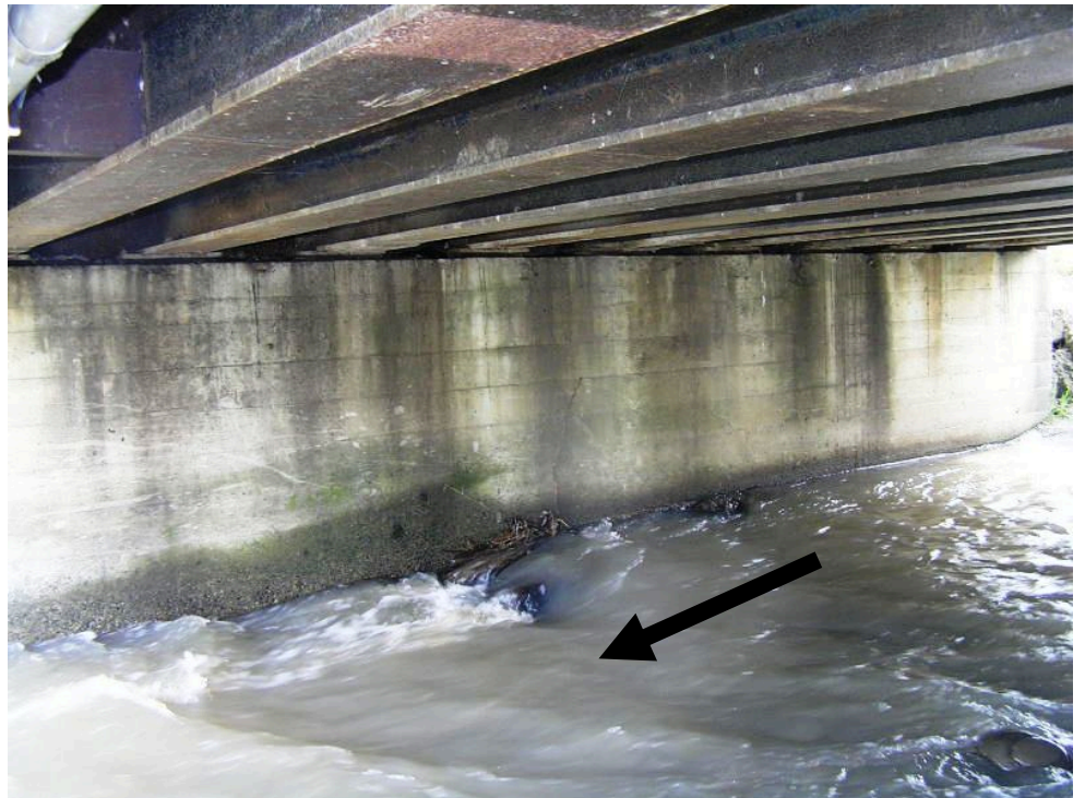
Figure 13.2.59 Accelerated Flow Due to Constricted Waterway
