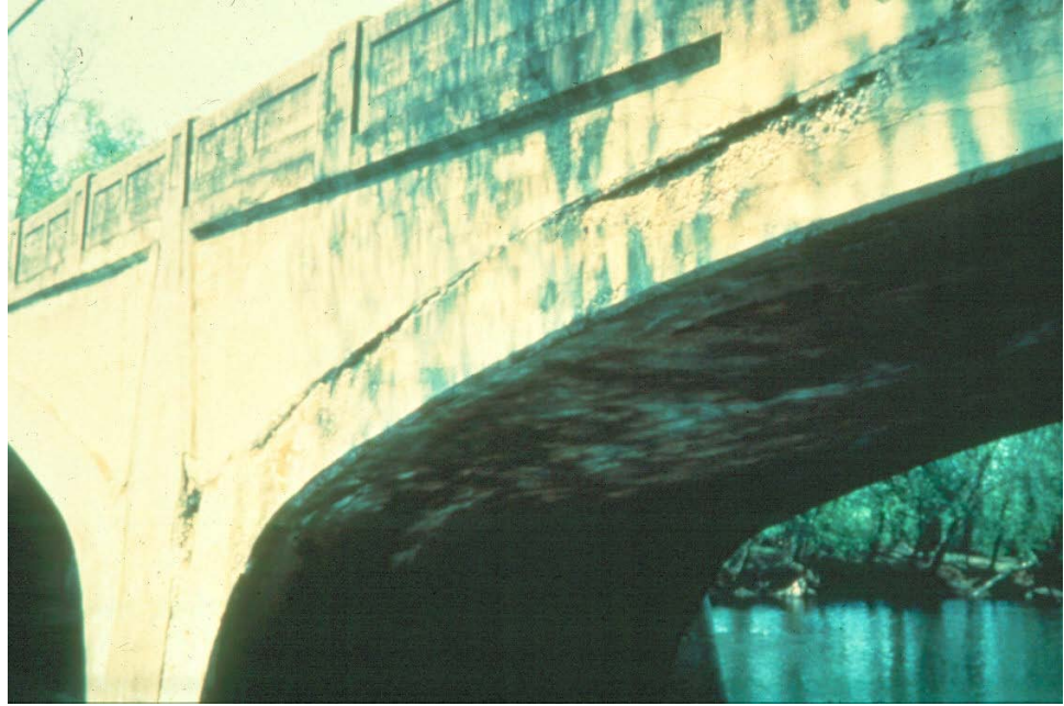
Figure 9.5.15 Deteriorated Arch/Spandrel Wall Interface
