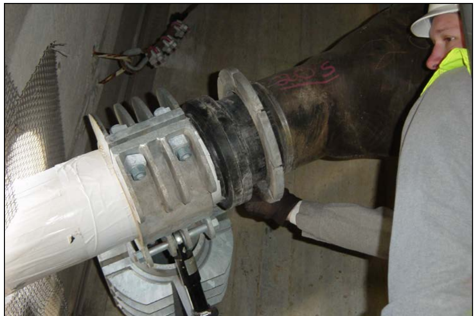
Figure 16.1.35 Damper on Cable-Stayed Bridge
