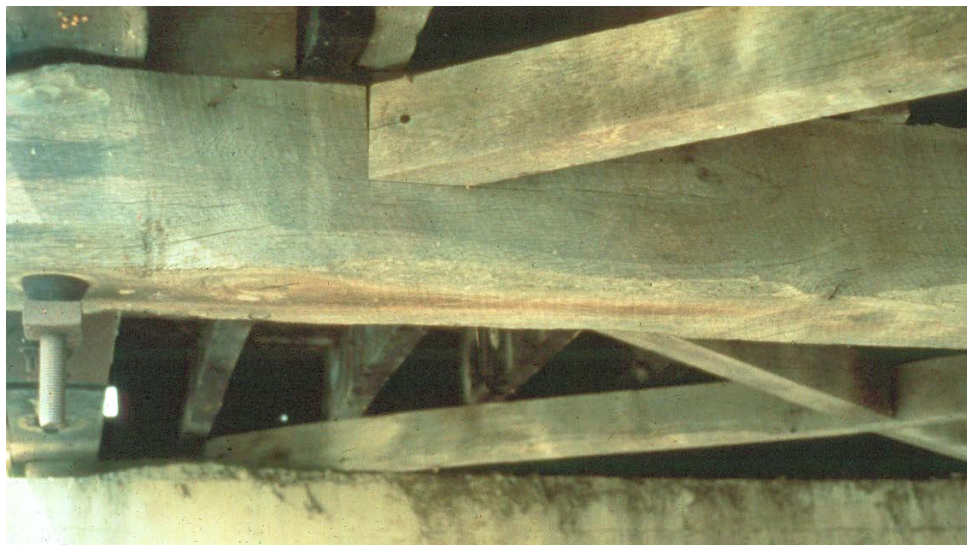
Figure 6.1.19 Loose Hanger Connection Between the Timber Truss and Floorbeam
