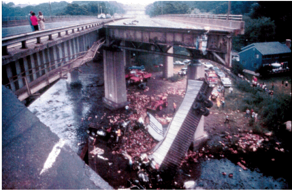
Figure 6.4.2 Mianus River Bridge Collapse
