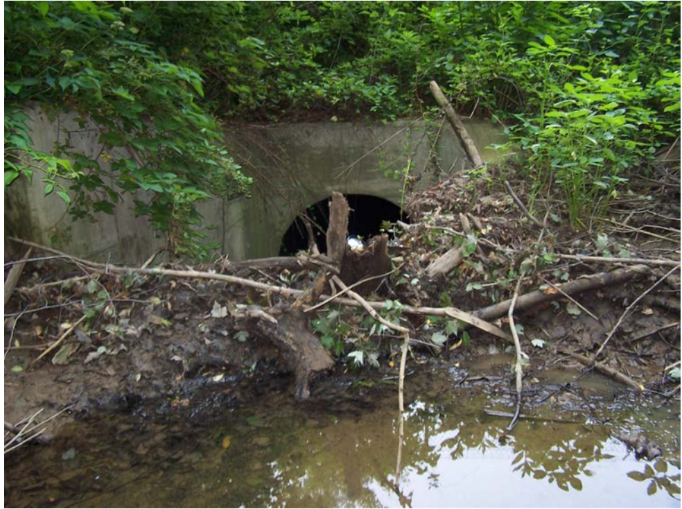
Figure 14.1.28 Debris and Sediment Buildup
