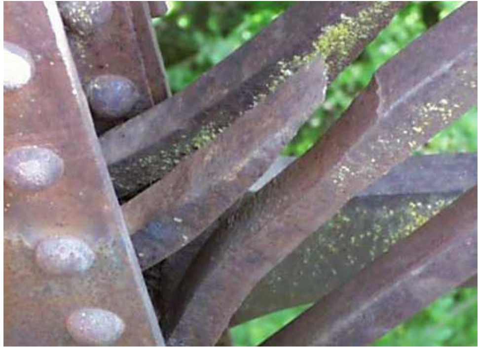
Figure 10.4.44 Cracked Forge Zone on a Loop Rod
