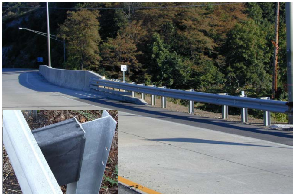
Figure 7.6.9 Approach Guardrail System and Approved Plastic Offset Block
