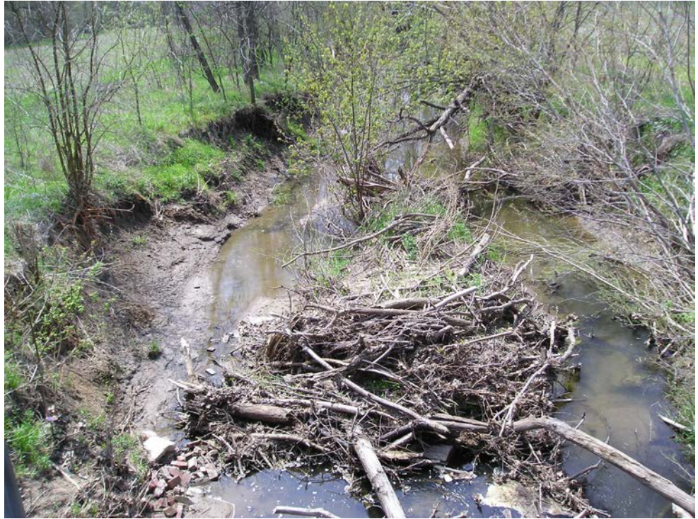
Figure 13.2.48 Debris and Sediment in the Channel
