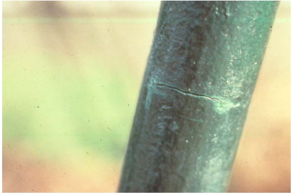
Figure 16.1.46 Cracking of Cable Sheathing
