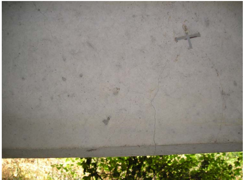
Figure 9.2.13 Flexure Cracks on a Tee Beam Stem
