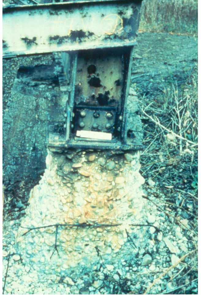
Figure 12.2.35 Deterioration of Steel Bent Leg
