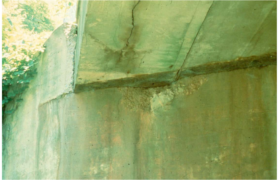
Figure 9.10.13 Longitudinal Cracks in Bottom Flange of Beam
