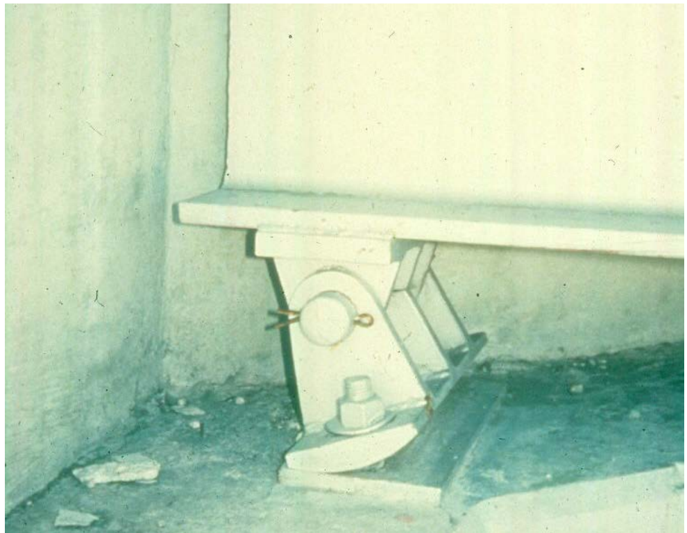
Figure 12.1.43 Excessive Rocker Bearing Displacement Indicating Possible Lateral Displacement of Abutment
