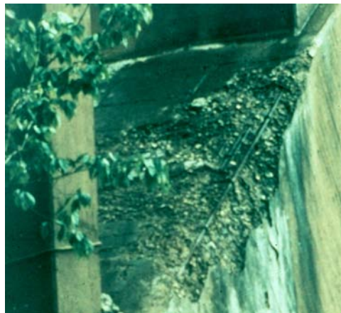
Figure 9.5.18 Scaling and Contamination on an Arch Rib Due to a Failed Drainage System
