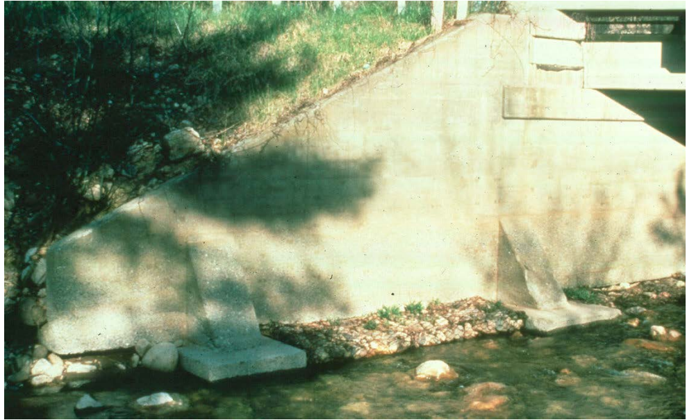
Figure 12.1.52 Scour and Possible Undermining of Concrete Wingwall
