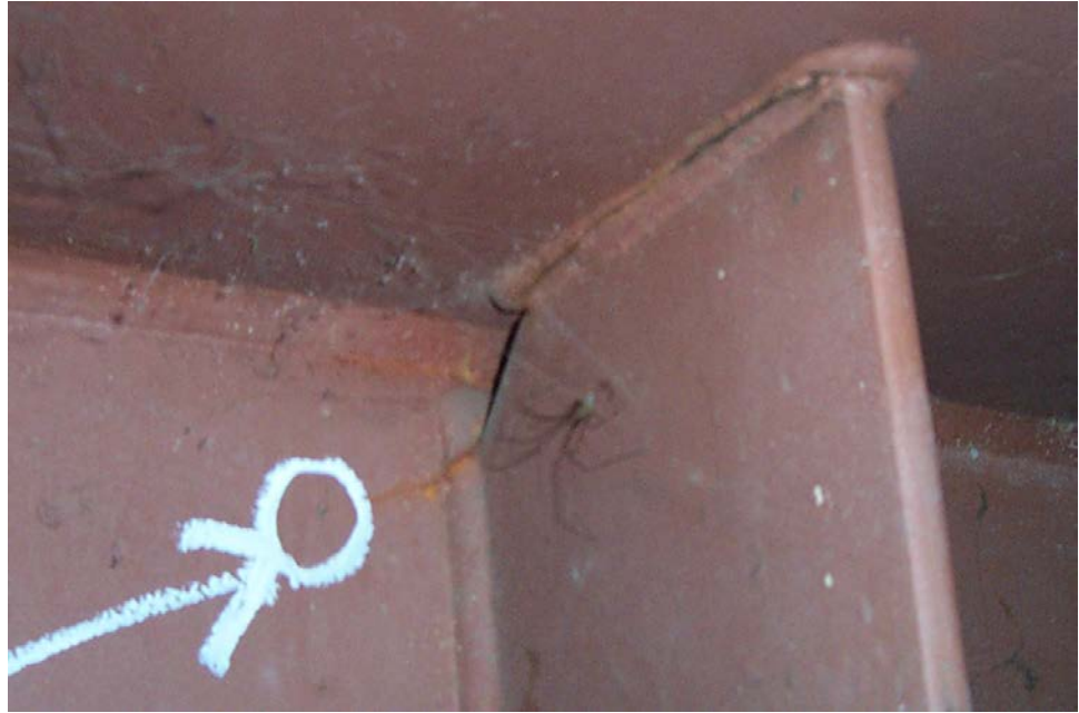
Figure 6.4.56 Web Crack due to Out-of-Plane Distortion at Top Flange
