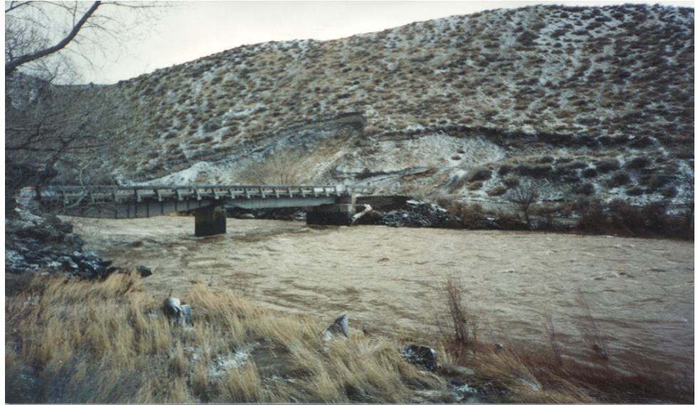
Figure 13.3.20 Severe Flood-Induced Abutment Scour
