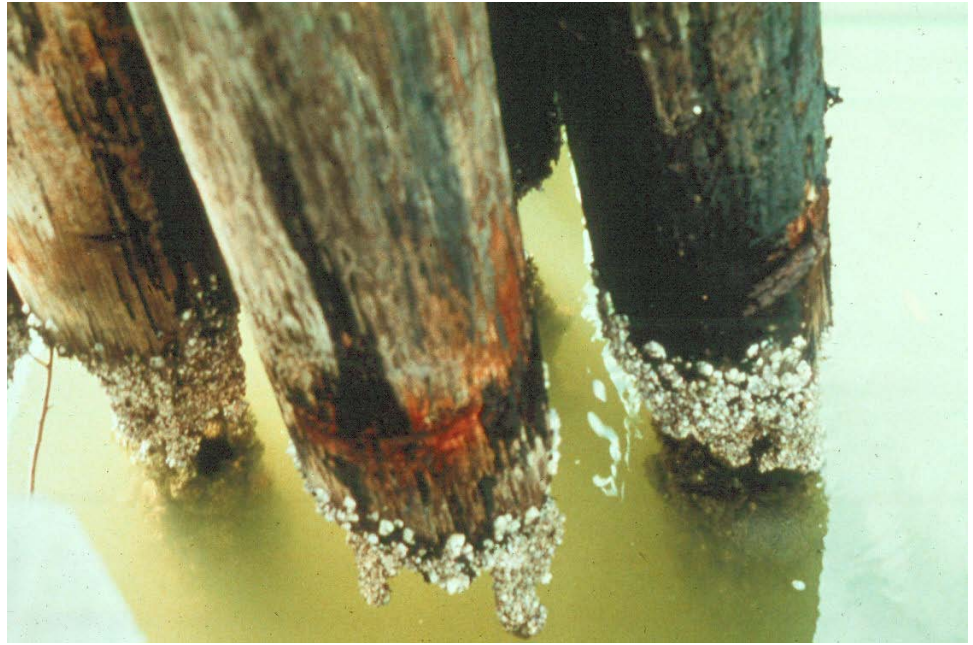
Figure 12.2.42 Timber Pile Damage due to Limnoria Marine Borers
