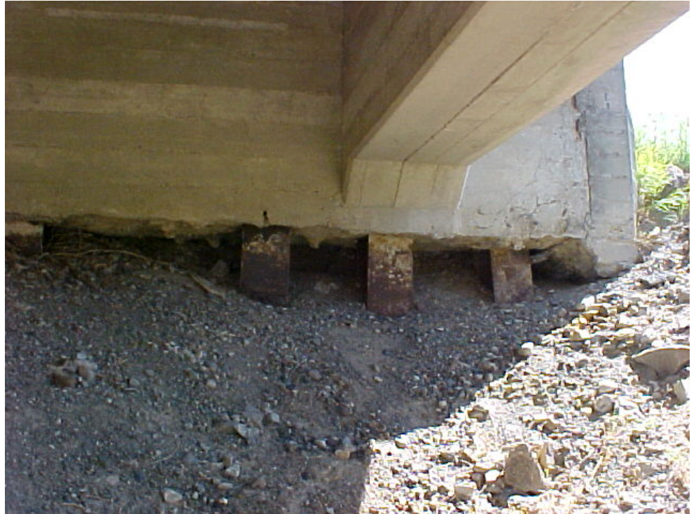
Figure 13.2.58 Exposed Piling Due to Scour
