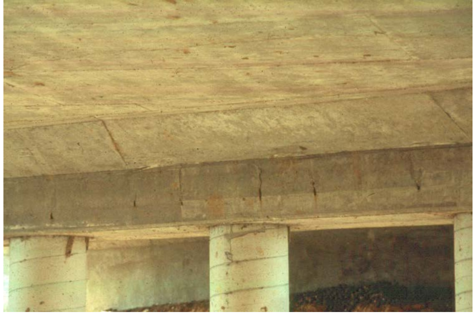
Figure 9.1.6 Shear Zone on the Underside of a Continuous Slab Bridge Near a Pier
