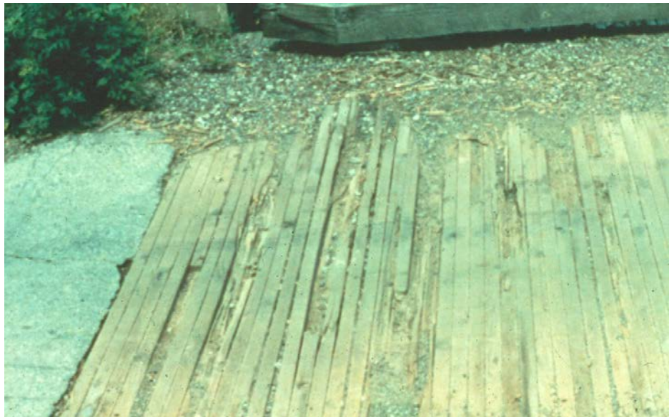
Figure 6.1.22 Wear of a Timber Deck
