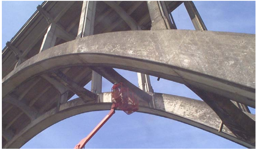
Figure 9.5.17 Inspection and Documentation of Arch Strut Deficiencies
