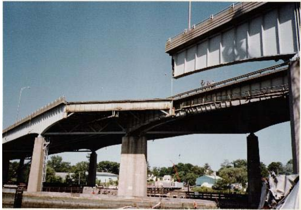
Figure 10.7.15 Mianus River Bridge Failure
