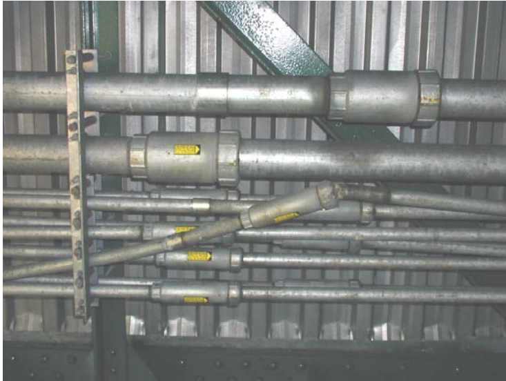
Photo No. 13 Conduit and Couplers, Span 1 – note bend in conduit, and coupler separation
