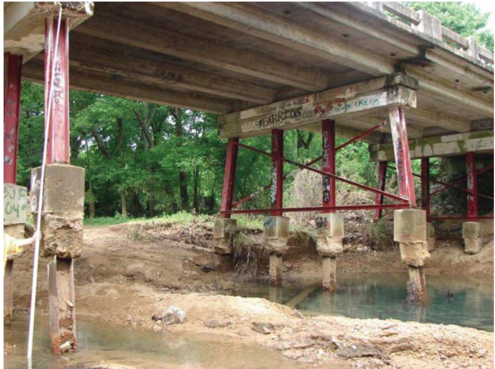
Figure 13.2.41 Severe Streambed Degradation Evident at Low Water
