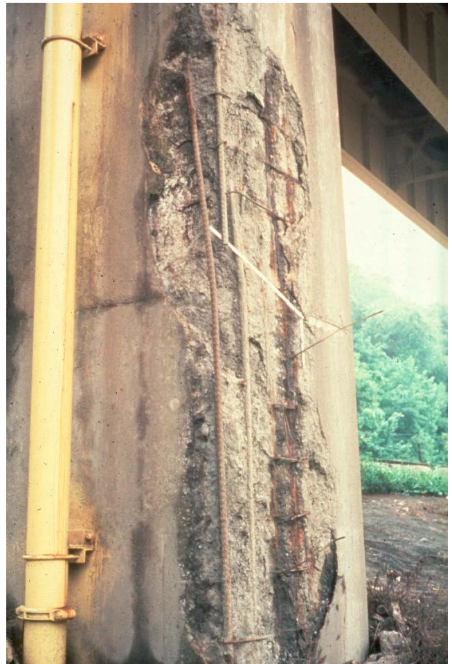
Figure 12.2.30 Concrete Spalling due to Contaminated Drainage
