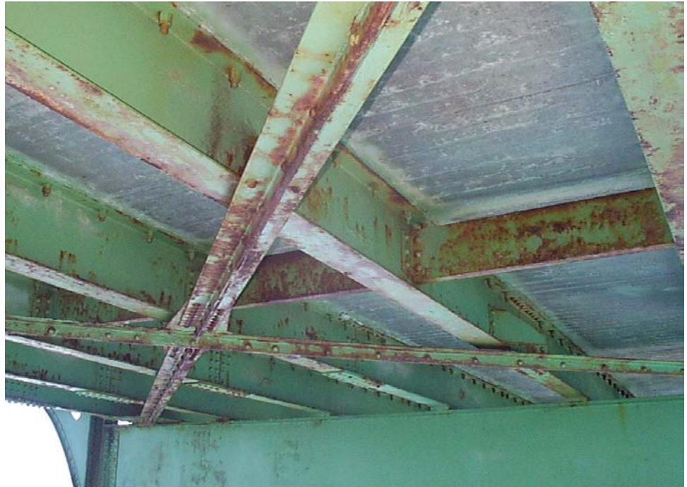
Figure 10.4.57 Lateral Bracing with Corrosion
