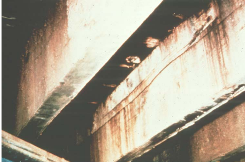
Figure 8.1.12 Horizontal Shear Crack in a Timber Beam
