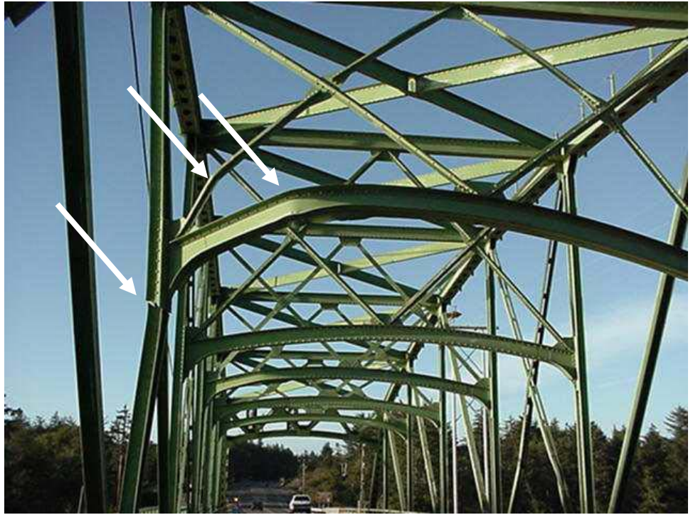
Figure 10.4.49 Collision Damage to Truss Members Due to Overheight Vehicle
