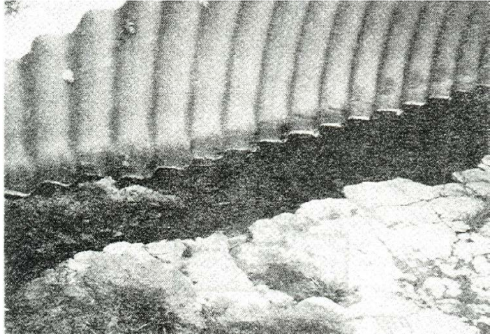
Figure 14.3.21 (Exhibit 79) Erosion Damage to Concrete Invert
