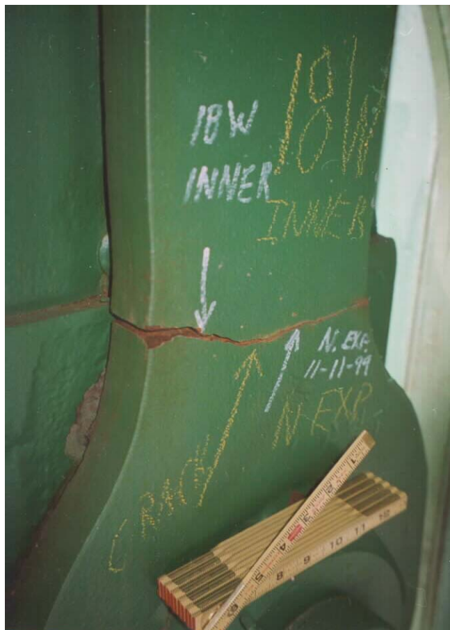
Figure 10.4.43 Cracked Forge Zone on an Eyebar
