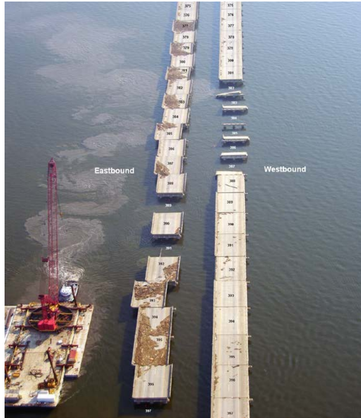
Figure 13.1.1 Failure Due to High Water Levels During Hurricane: Aerial View
