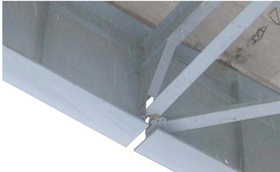
Figure 6.4.47 Local Triaxial Constraint Condition Resulting in Fracture on the Hoan Bridge, Milwaukee, Wisconsin
