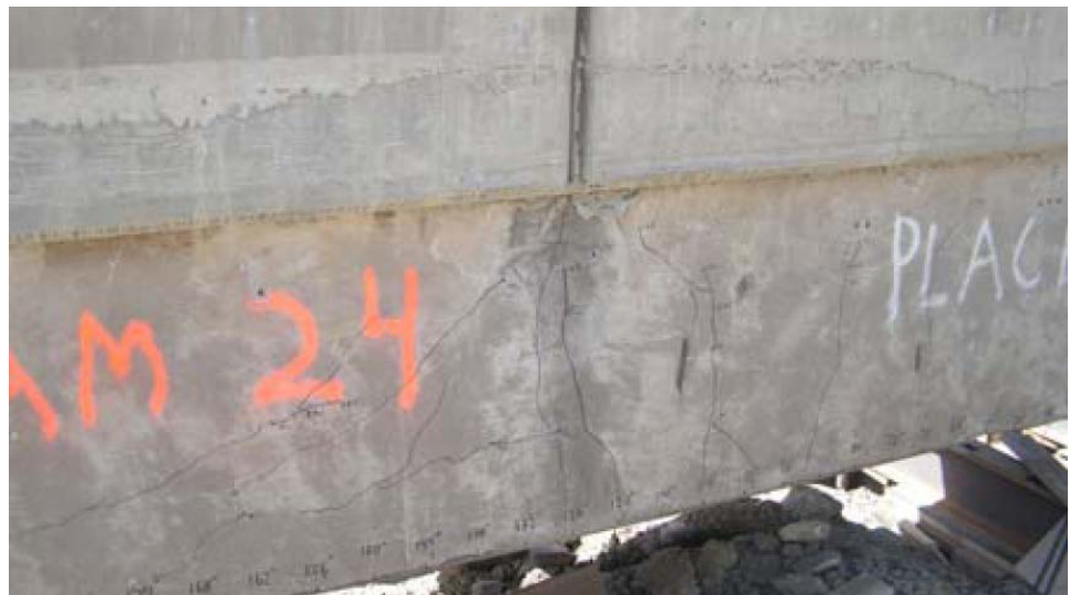
Figure 9.10.28 Cracking Near Barrier Joints
