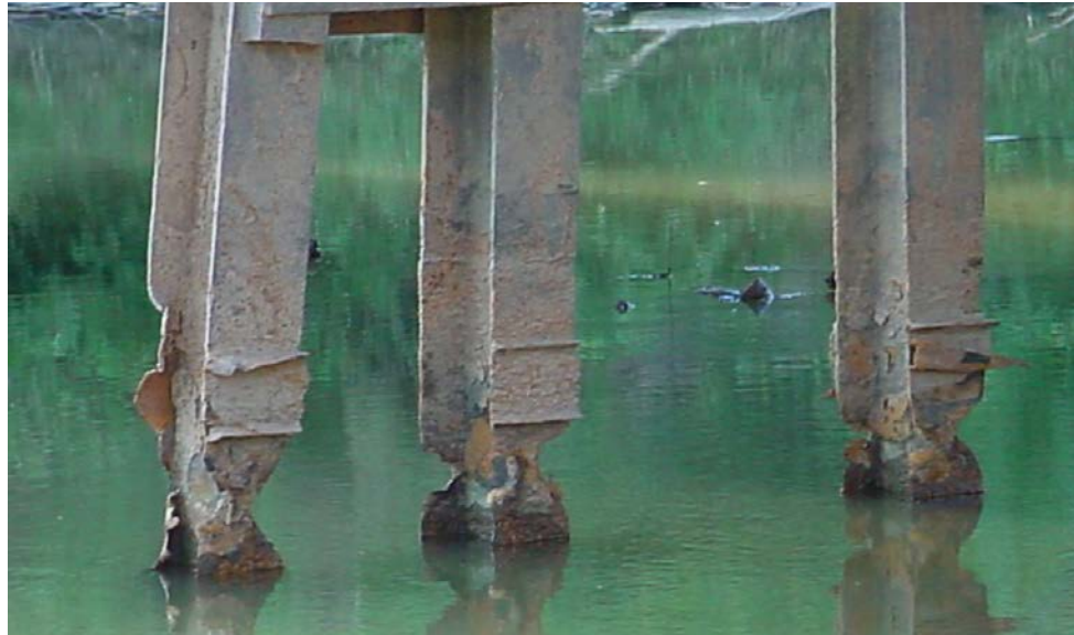
Figure 13.3.25 Deteriorated Steel Piles at Splash Zone
