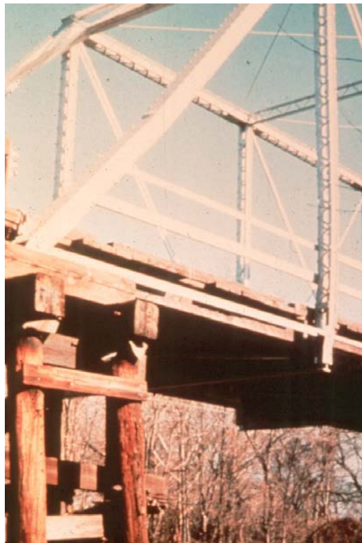
Figure 10.4.50 Buckled End Post
