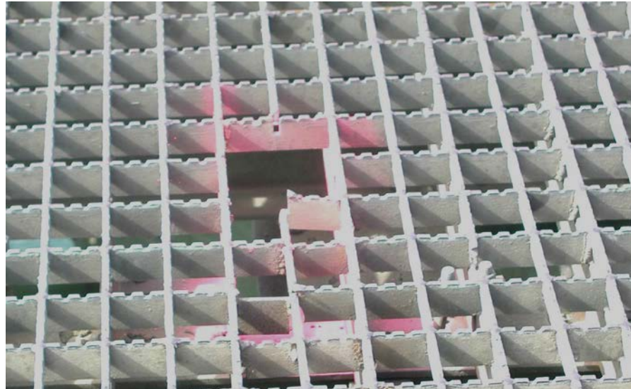
Figure 7.4.10 Broken Members of an Open Steel Grid Deck
