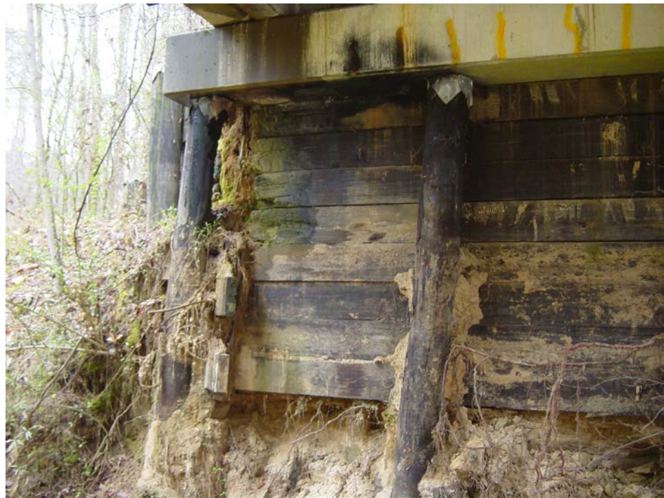
Figure 13.2.50 Scour at a Pile Abutment
