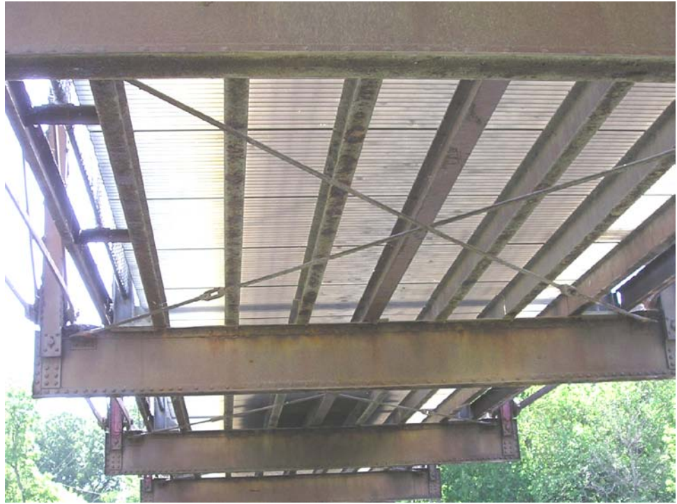
Figure 10.4.53 Corroded Stringers under an Open Grid Deck
