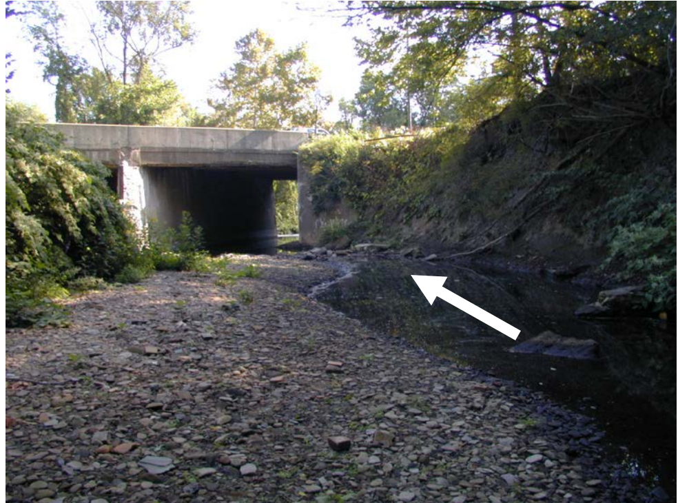
Figure 13.2.53 Typical Misaligned Waterway
