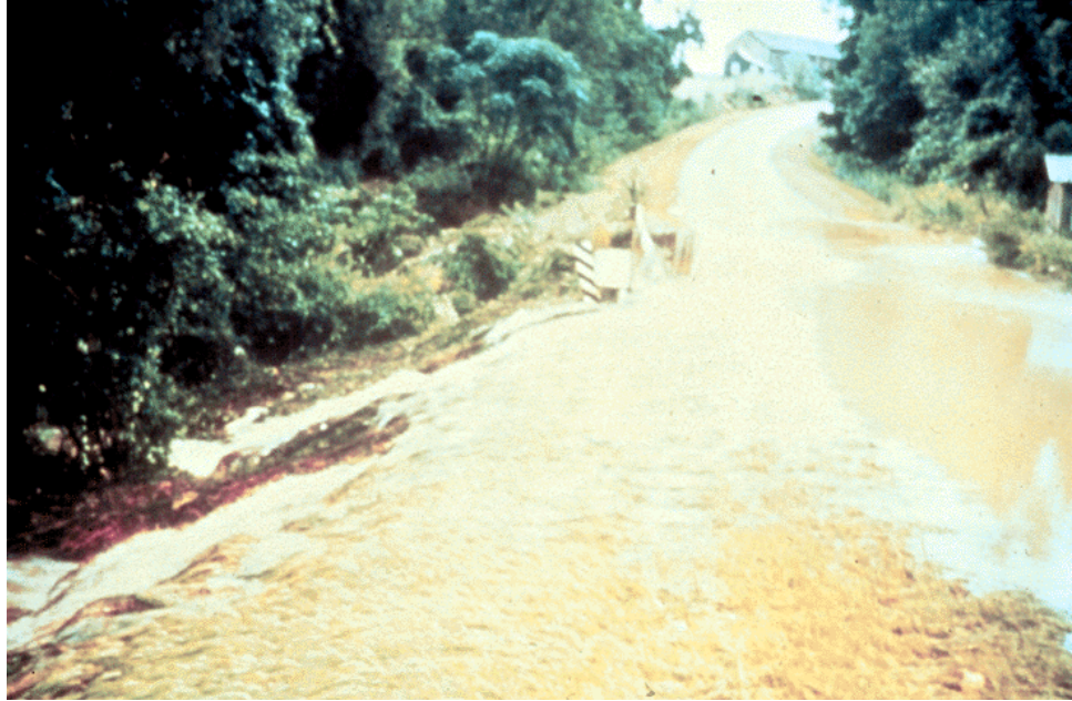
Figure 13.2.63 (Exhibit 63) Culvert Failure Due to Overtopping
