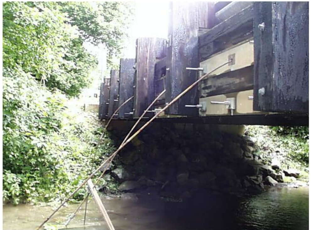
Figure 7.1.11 Broken Prestressing Anchors
