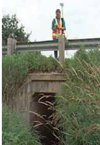
A field inspector uses a global positioning system receiver to collect data that will be recorded in HYDINFRA.
