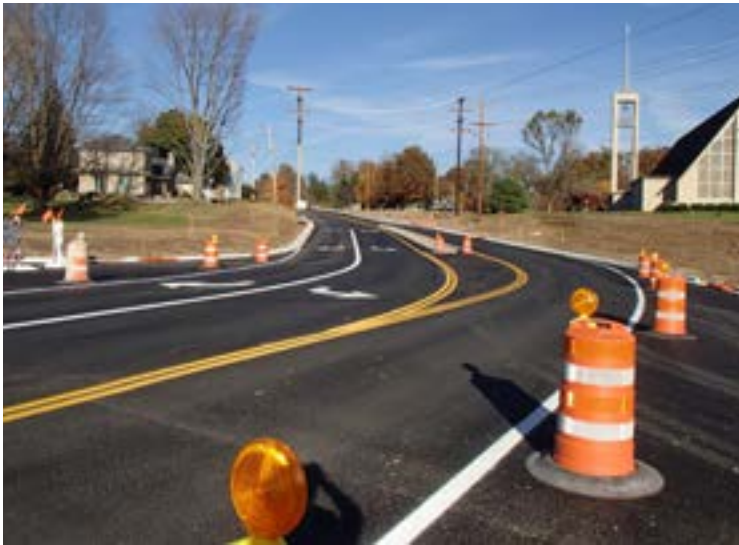
The Hamilton Road improvement project in Franklin County, Ohio, is one of the more than 250 projects administered annually through ODOT's Local Let program. (Photo courtesy Franklin County, Ohio)
