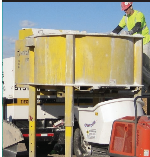
Figure 13. Portable concrete pan mixer preparing UHPC for placement during the construction of the field-cast connections.
