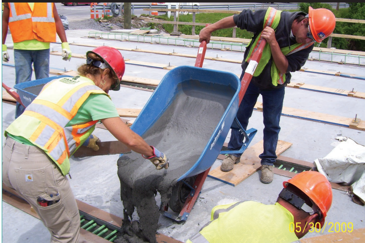
Figure 14. Longitudinal connections cast between deck-bulb-tee girders on the Route 31 bridge in Lyons, NY.
