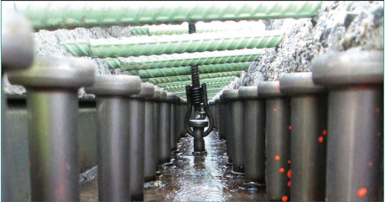
Figure 21. Longitudinal connection detail above first interior girder line with shear studs stopping below the bottom mat of rebar.
