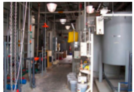
Industrial Wastewater Treatment Plant
