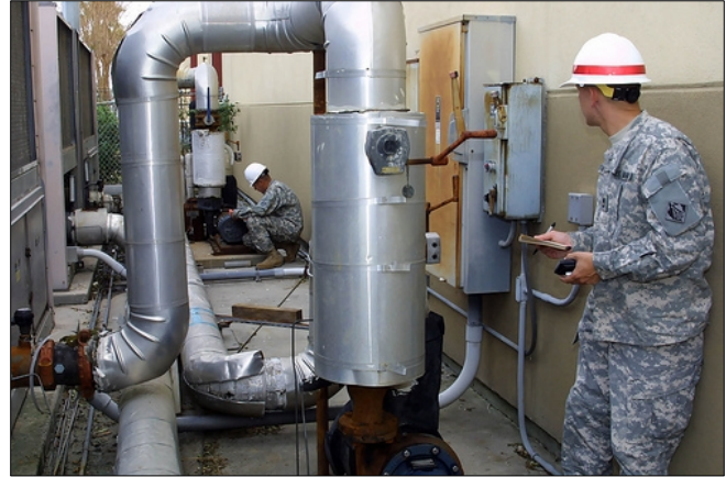
Soldiers from the 249th Engineer Battalion (Prime Power) check the electrical requirements for an air conditioning unit at a community center in 2008 in Galveston, Texas after Hurricane Ike struck. Teams of power experts from the unit deployed to provide temporary power to critical facilities where needed. (Photo by Brooks O. Hubbard IV, Los Angeles District)
