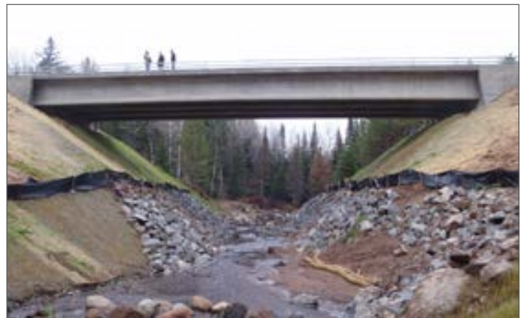
The CM/GC process helped expedite delivery of a new bridge for the Reservation while saving approximately $150,000 in engineering costs. (Photo courtesy: Central Federal Lands Highway Division)
