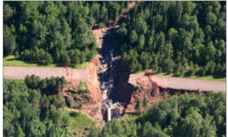
Floodwaters damaged the culvert and washed out more than 100 feet of road at a creek crossing on the Fond du Lac Reservation in Minnesota during June 2012. (Photo courtesy: Central Federal Lands Highway Division)
