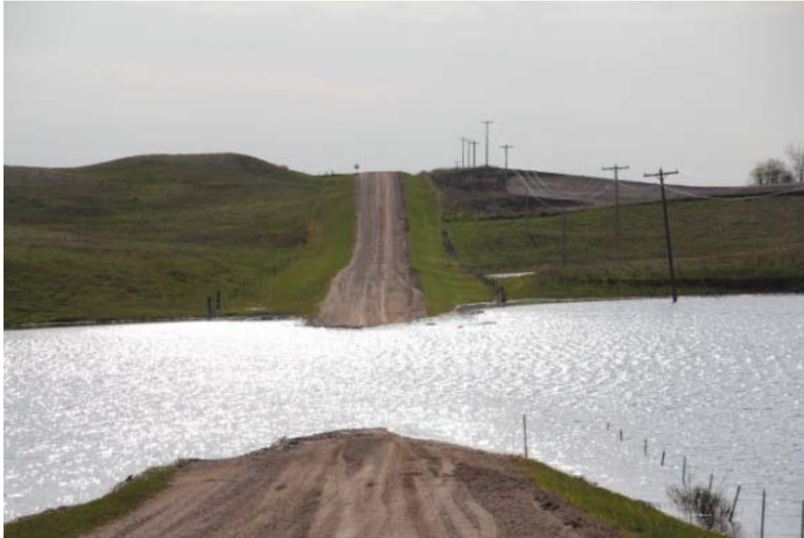
Photo: Ward County Road, 20 miles south of Minot, ND. Source: FHWA North Dakota Division Office
