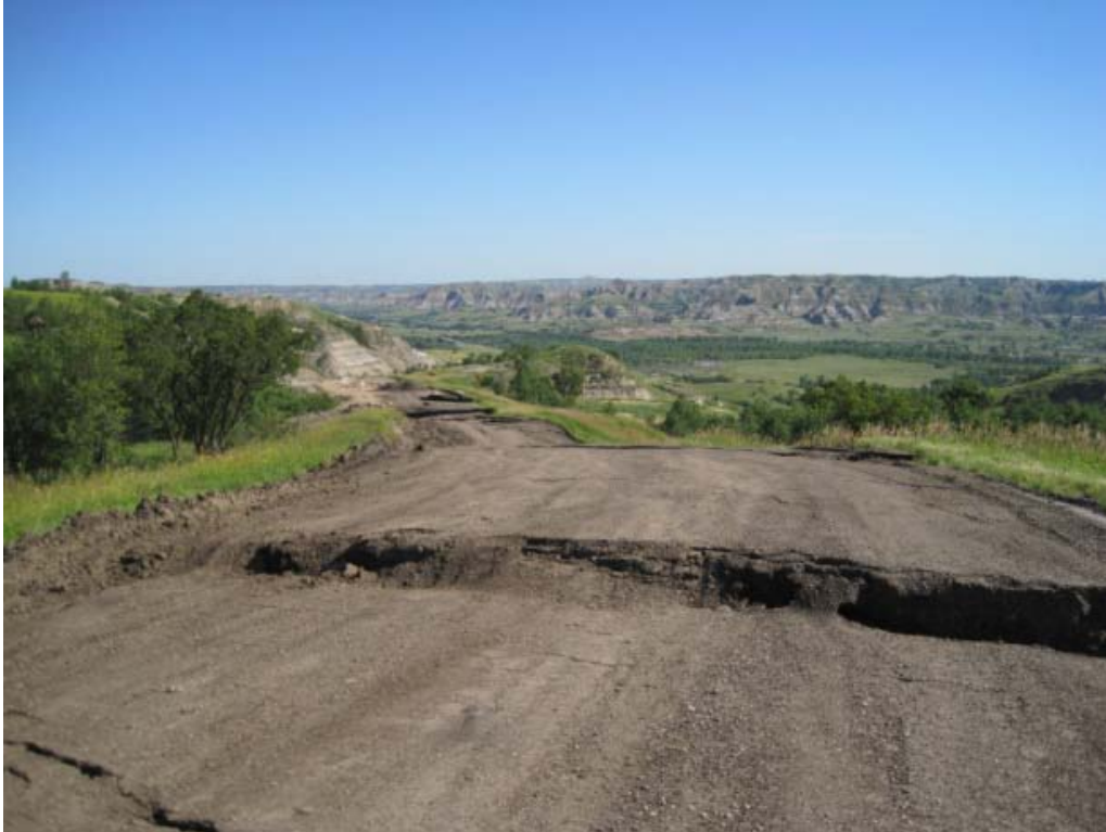
Photo: ND 22 about 14 miles north of Killdeer. Source: FHWA North Dakota Division Office.
