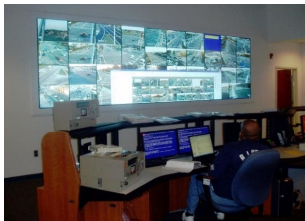
Figure 3. City of Virginia Beach Traffic Management Center (TMC)
