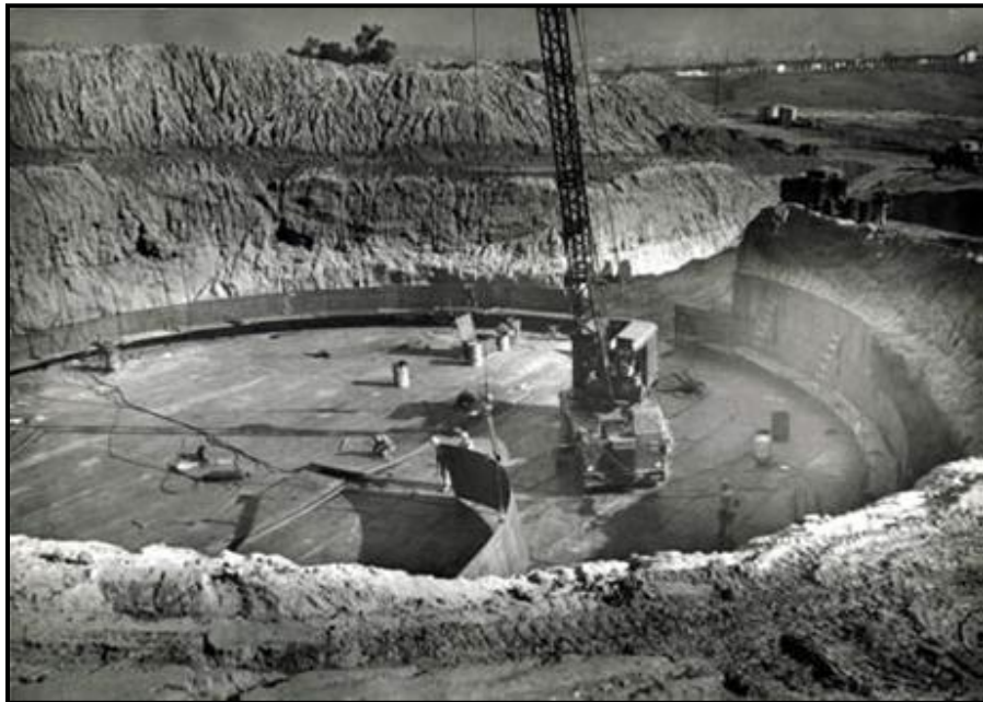
Photo 3.2-1. Construction of an UST at the Main Terminal from 1952 – 1954 during the Korean Conflict (DLA 2008)
