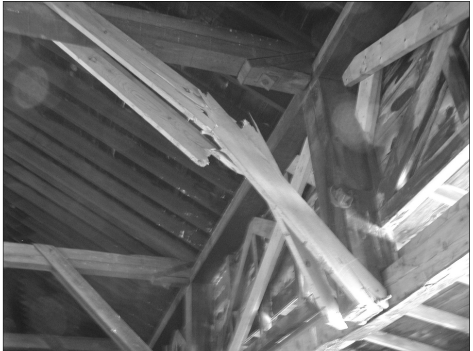
Figure 5: Structurally Unsound Warehouse at Fort Leavenworth, Kansas
