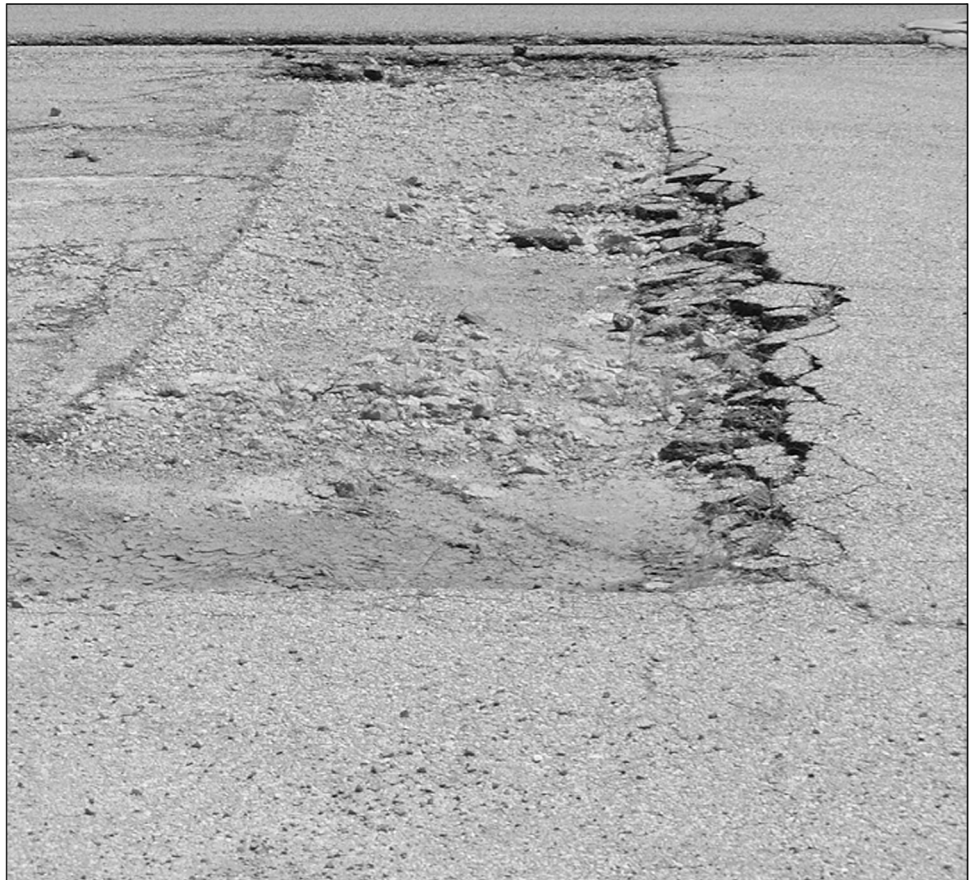
Figure 7: Crumbling Concrete Outside Cargo Center at Whiteman Air Force Base, Missouri
