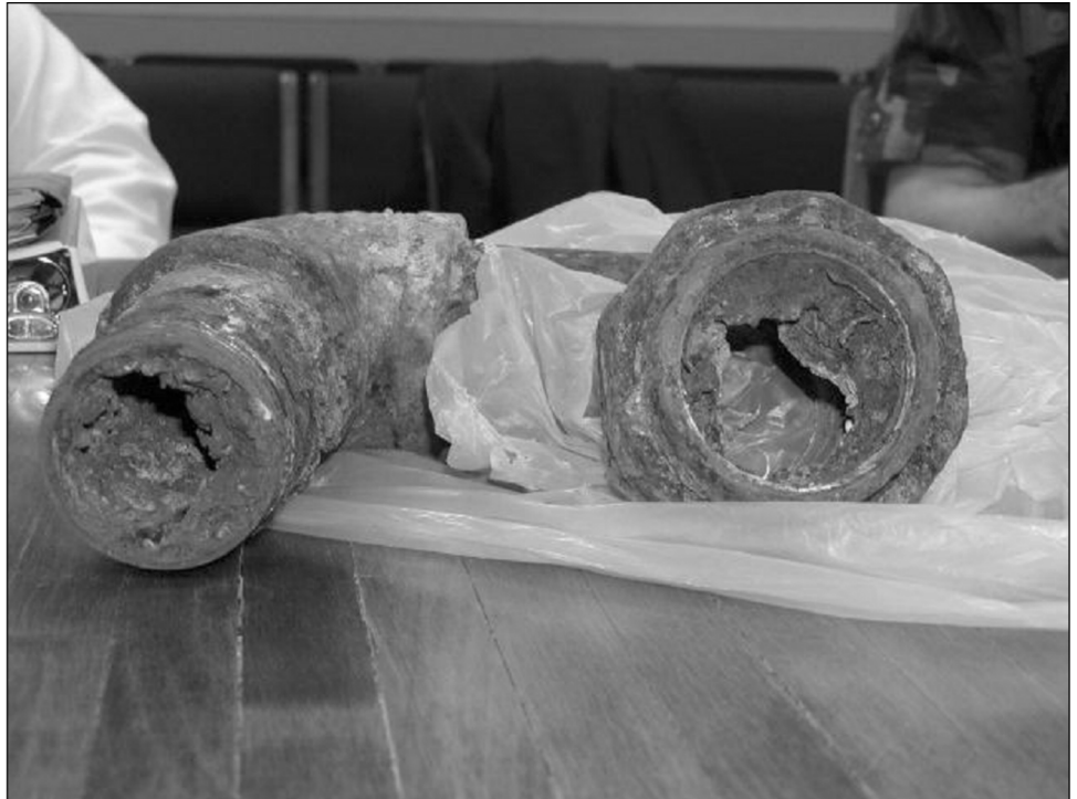
Figure 6: Choked and Clogged Water Pipes at Pope Air Force Base, North Carolina
