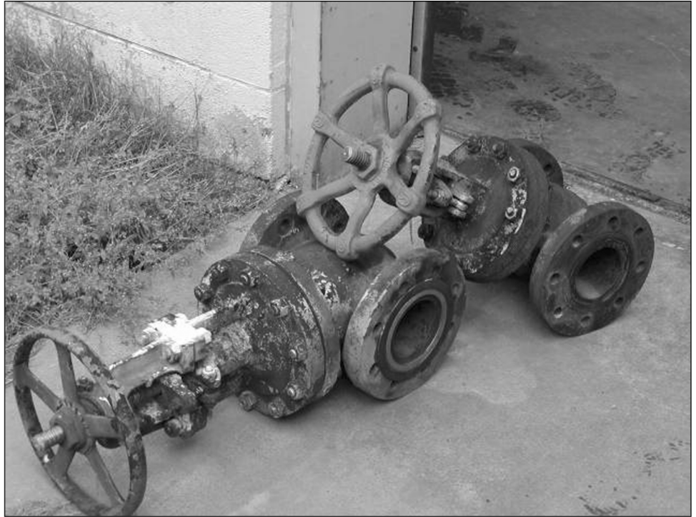
Figure 10: Corroded Air-Conditioning System Valves at Quantico Marine Corps Base, Virginia
