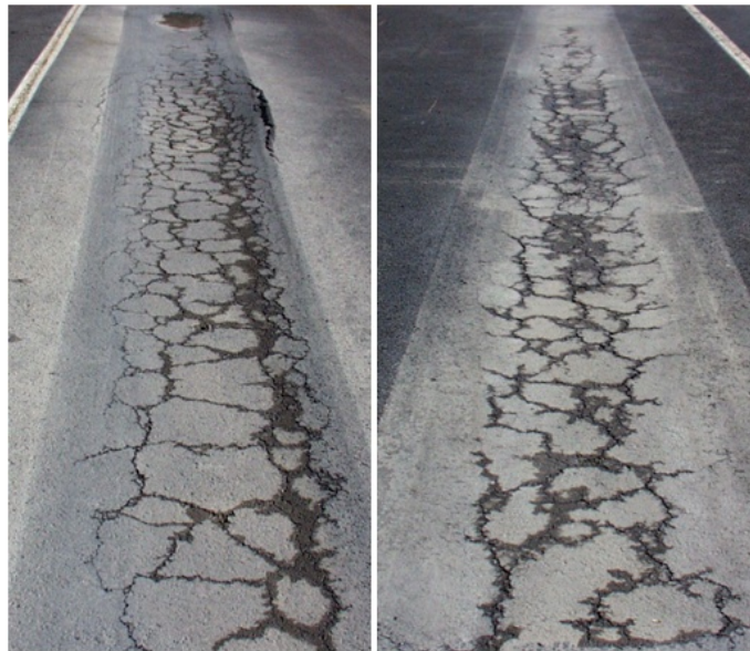
Figure 31. Photo. Typical cracking pattern in loaded ALF wheel paths.
