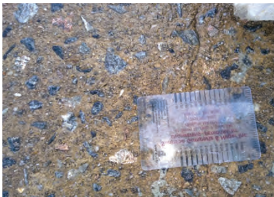
Figure 2. The wearing surface of the I-16 slab section in Dublin, GA, and one of the few cracks present. (It is not known if the crack was present before slab removal.)
