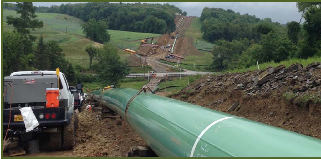
A new 36-inch diameter transmission pipeline segment as it is about to undergo PHMSA inspection in August 2014. Upgrades stretching from this point in Holbrook, PA across the state and several others allow for an increase in natural gas capacity and bidirectional flow capability. Photo by PHMSA Eastern Region.
