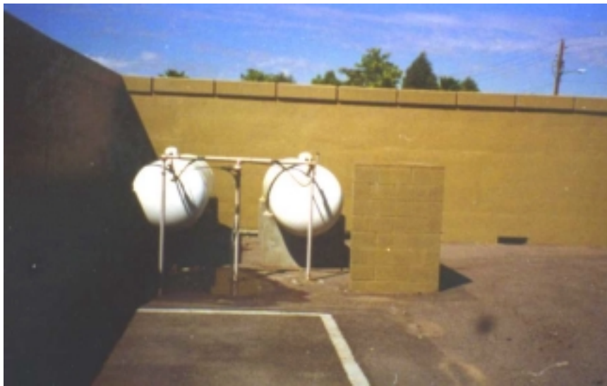
Figure 11-1. Liquid propane tanks for pump station power
