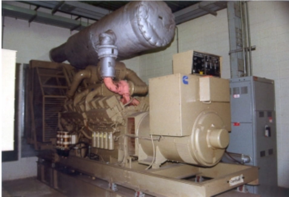
Figure 11-4. Diesel-powered backup generator
