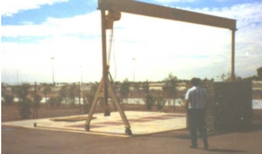
Figure 10-3. Overhead crane over wet well with submersible pumps
