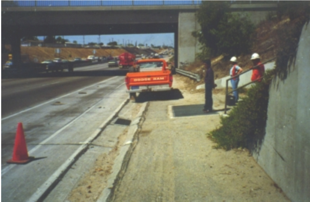
Figure 5-3. Limited access to pump station from shoulder of highway
