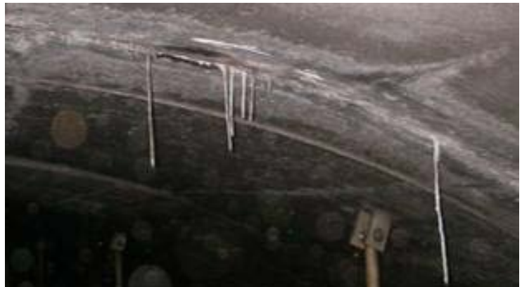
Figure 4.16 – Moderate cracking and efflorescence on the underside of the liner.
