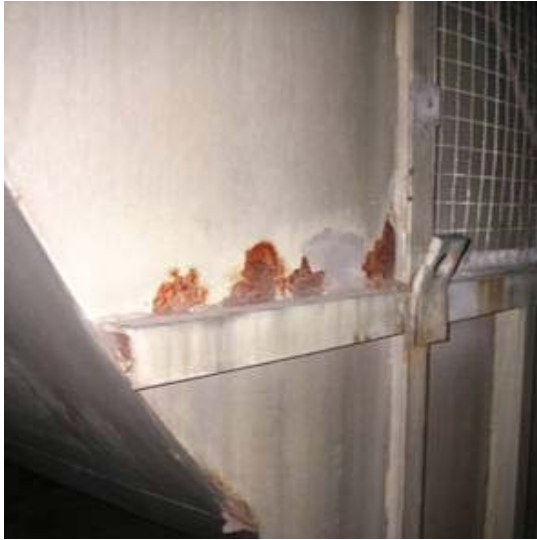
Figure 4.54 – Corroded fan housing.
