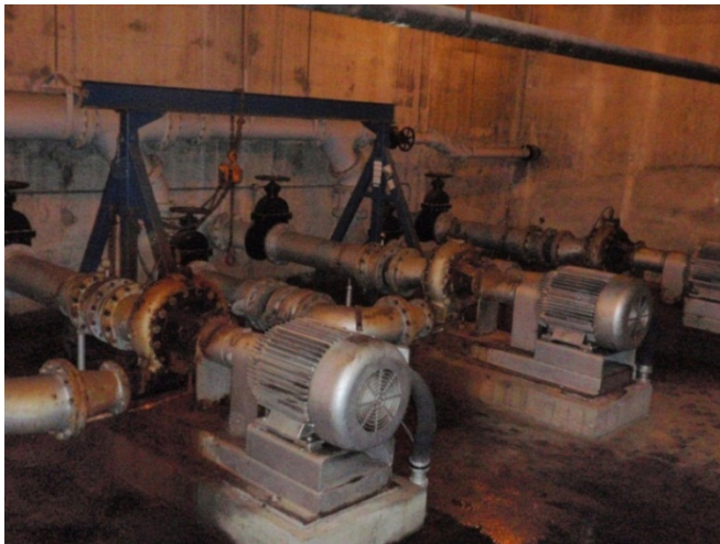
Figure 4.59 – View inside pump room.
