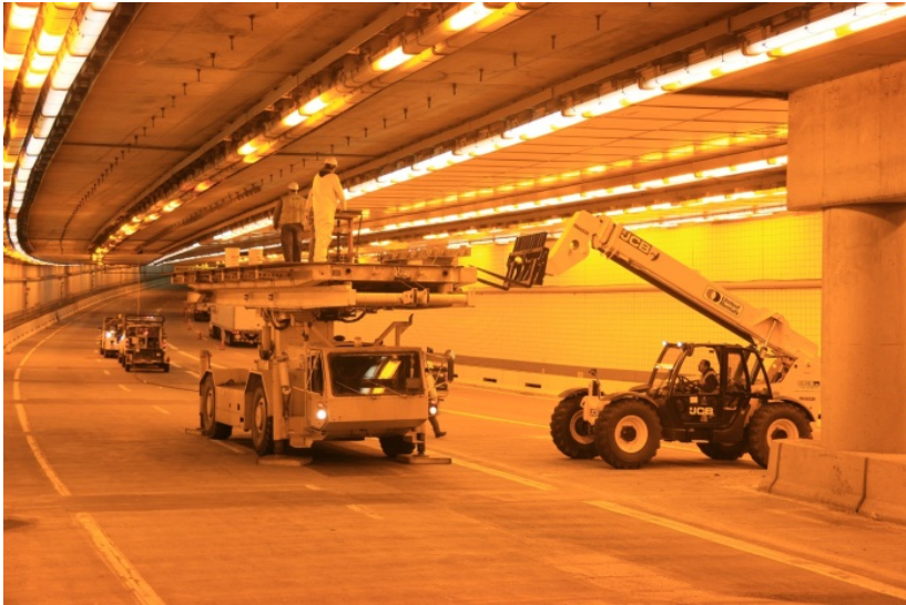
Figure 4.68 – Maintenance and inspection of lighting system.
