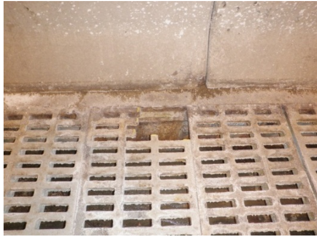
Figure 4.58 – Broken scupper grate.
