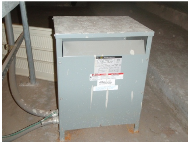
Figure 4.66 – Electrical equipment: Single phase insulated transformer.
