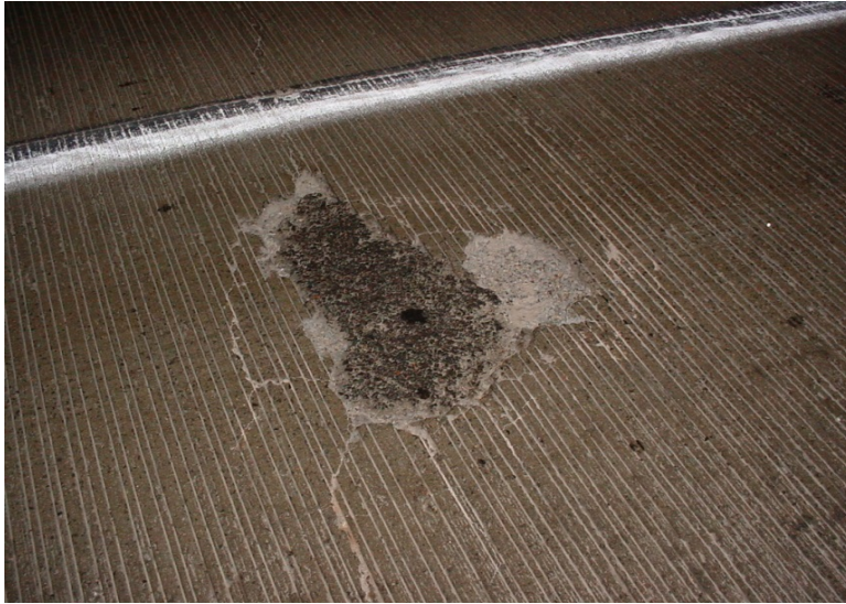
Figure 4.47 – Pothole with cracking in concrete wearing surface.
