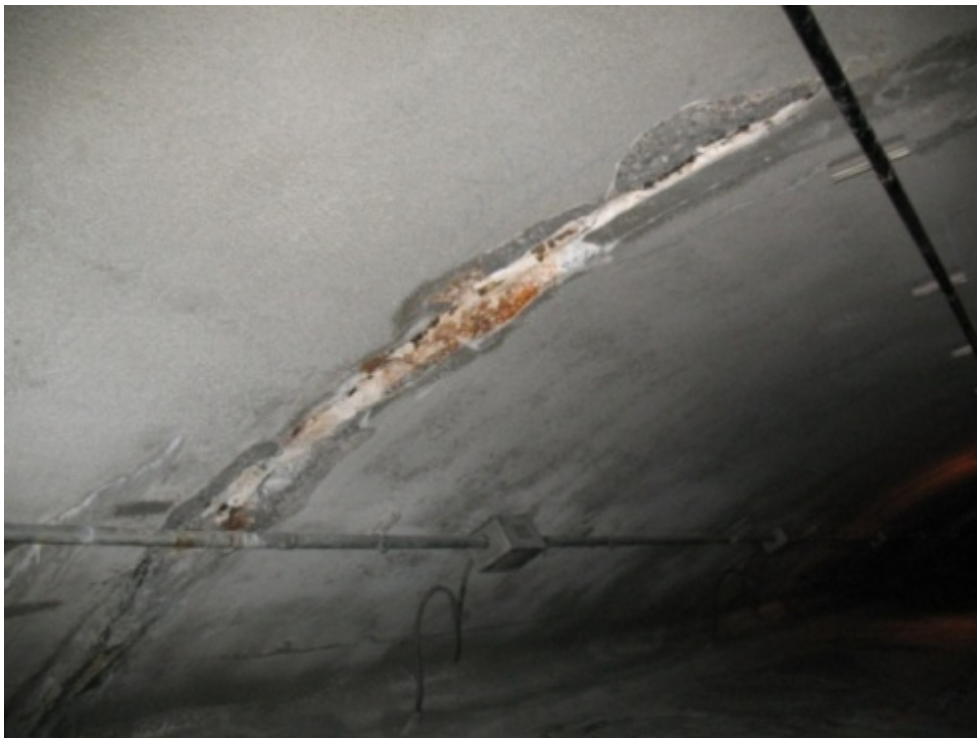
Figure 3.24 – Leakage at a construction joint through the cementitious coating (NCHRP, 2010).
