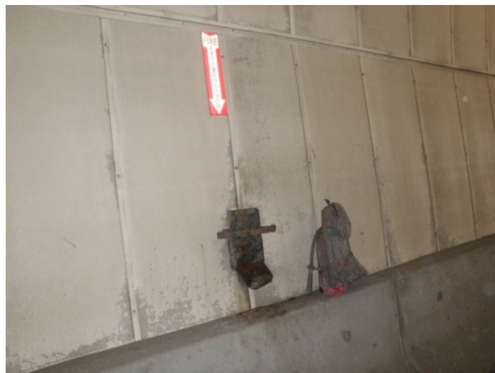
Figure 4.72 – Missing fire extinguisher.
