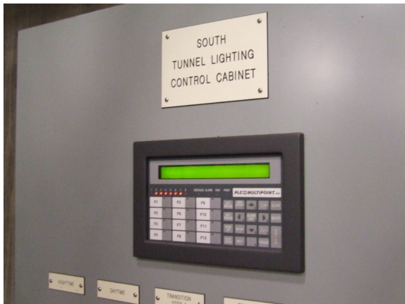
Figure 4.69 – Lighting control cabinet.
