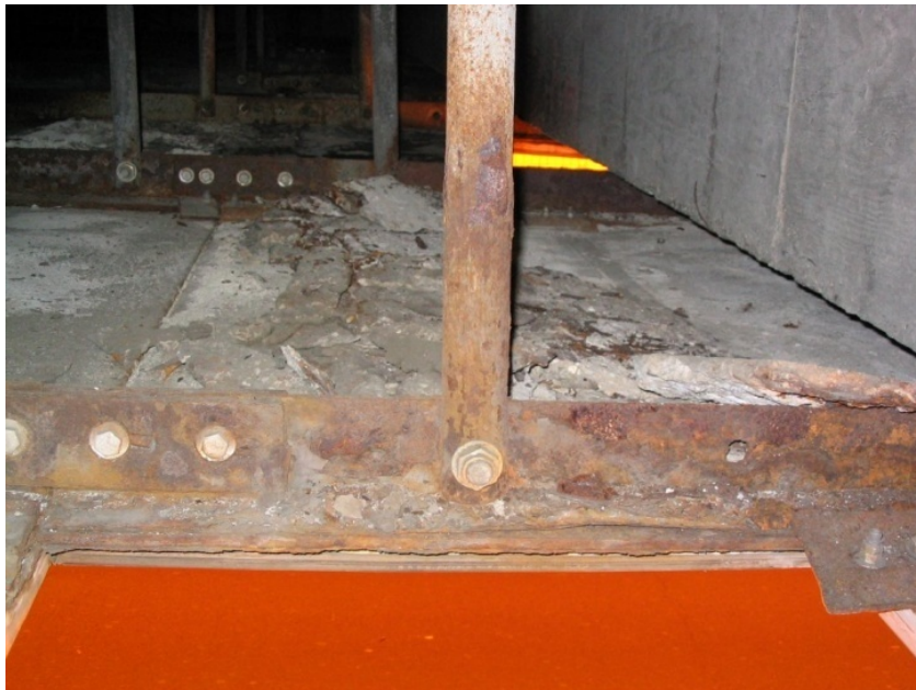
Figure 4.37 – Hangers and ceiling girders exhibiting moderate to heavy rust and minor section loss.
