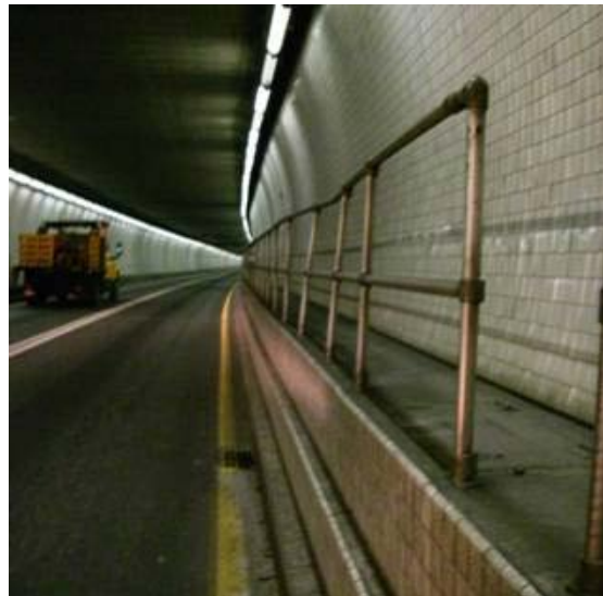
Figure 4.50 – Bent pedestrian railing with missing railing components.
