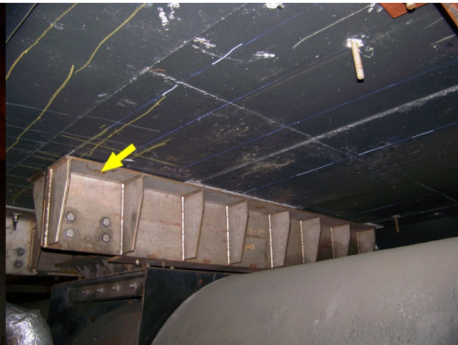
Figure 4.44 – Missing bolt at longitudinal fan support.
