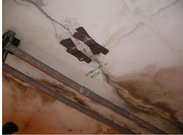
Figure 4.22 – Medium width crack in concrete liner.
