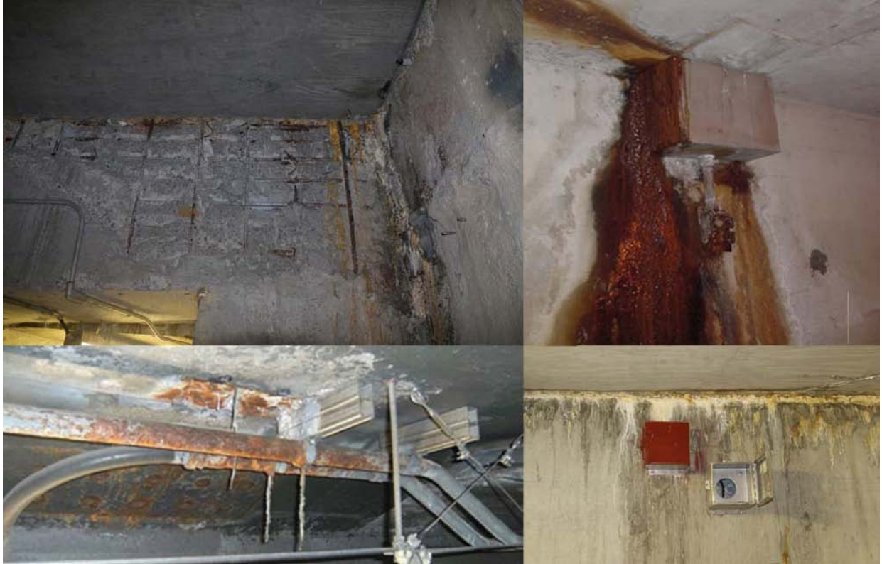
Figure 3.1 – Groundwater induced corrosion and deterioration.
