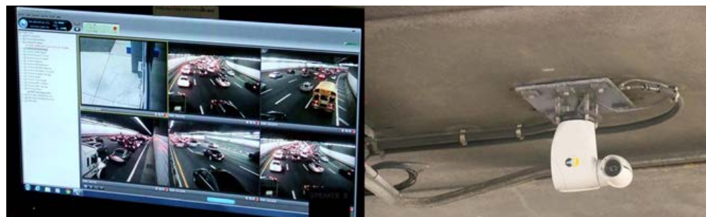
Figure 4.74 – Examples of CCTV camera systems.
