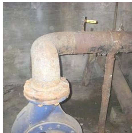
Figure 4.60 – Moderate corrosion to pipes, pipe supports and fasteners.
