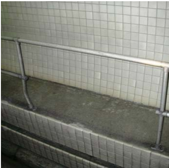
Figure 4.49 – Bent post and missing mid-rail.
