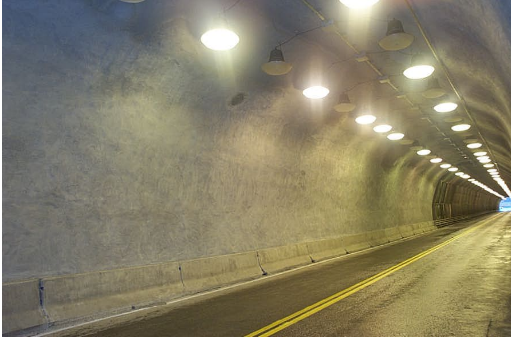
Figure 3.28 – New shotcrete lining over timber supports in rock tunnel. Note timber supports can be seen in the background (NCHRP, 2010).
