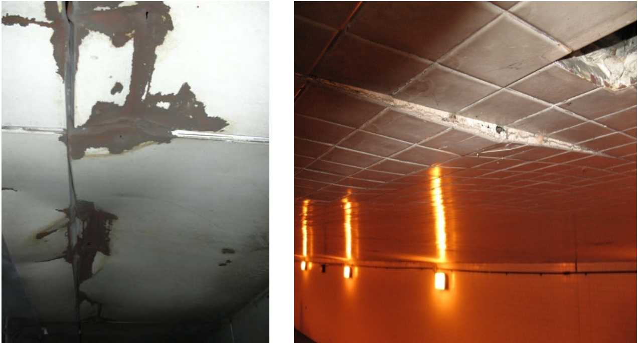
Figure 4.39 – Examples of damaged and deteriorated architectural finishes on underside of ceilings. Photo left is of damaged metal ceiling panels; right is deteriorated ceramic tile.
