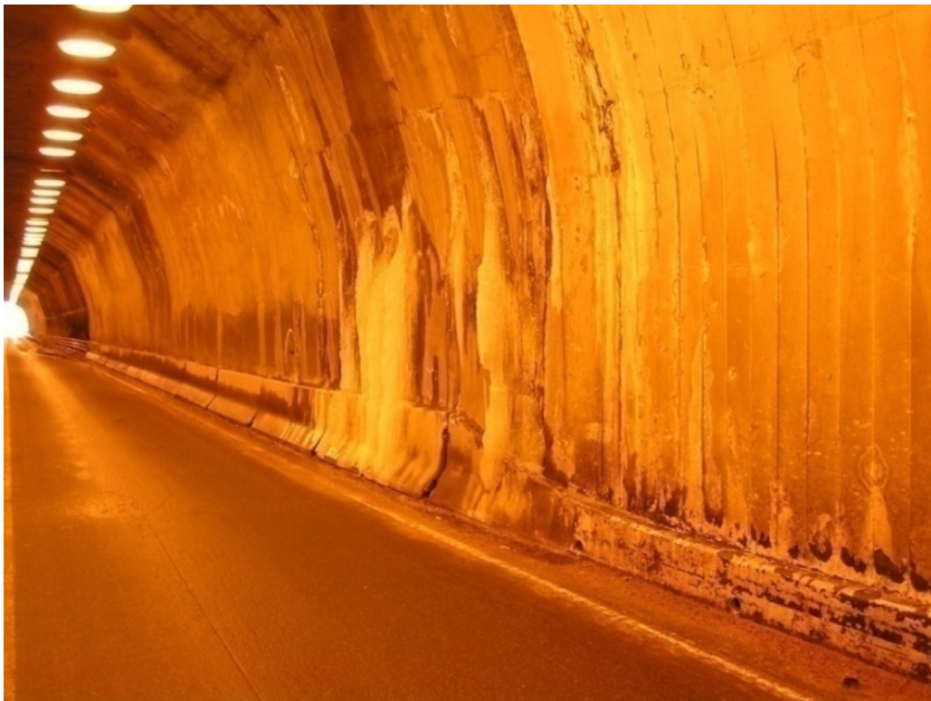
Figure 3.2 – Leakage through shotcrete liner (NCHRP, 2010).
