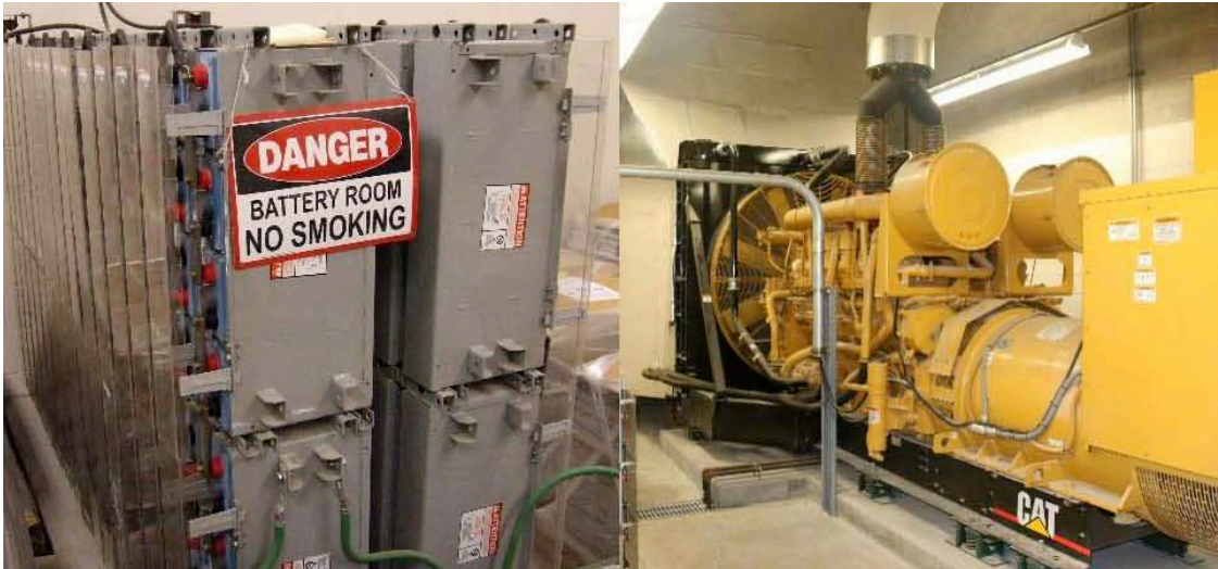
Figure 4.67 – Emergency power supply.
