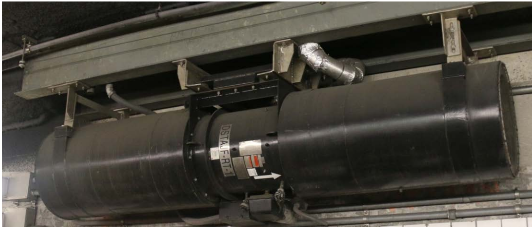
Figure 2.2 – Emergency ventilation fan.
