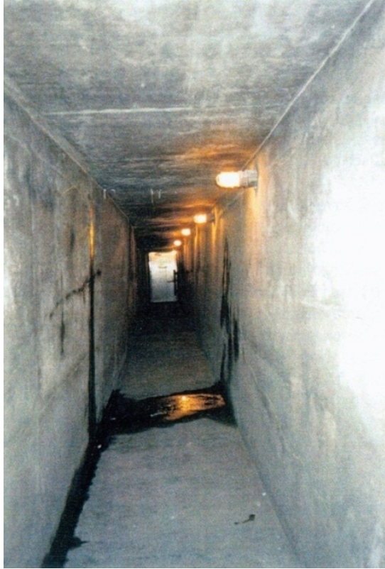
Figure 4.31 – Emergency corridor with minor leakage.
