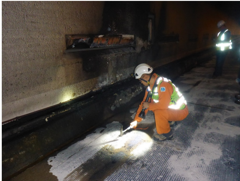
Figure 4.6 – Evaluating fire damage.
