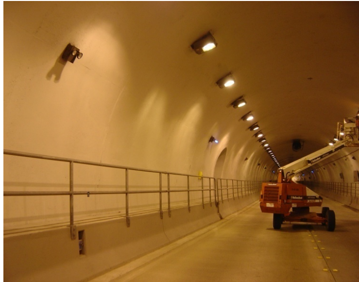
Figure 4.46 – Typical civil elements including wearing surface, traffic barrier, and pedestrian rail and walkway.
