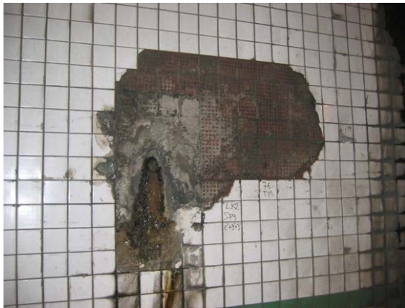
Figure 4.23 – Water leakage through tunnel liner and missing wall tiles.
