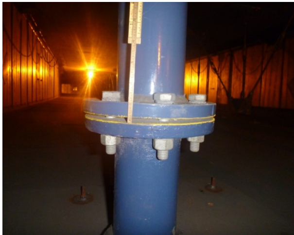
Figure 4.43 – Sign support with gaps at connection.
