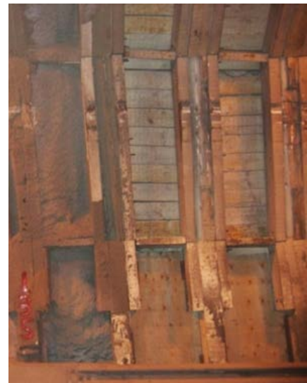
Figure 4.26 – Timber liner in state of deterioration.
