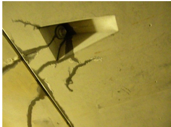
Figure 4.24 – Damp cracks in segmental liner due to improper installation techniques.
