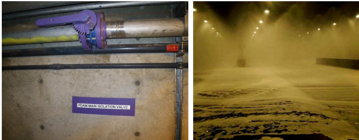
Figure 4.73 – Foam sprinkler system test.
