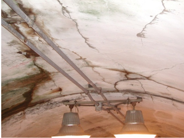
Figure 4.21 – Cracks with rust stains.
