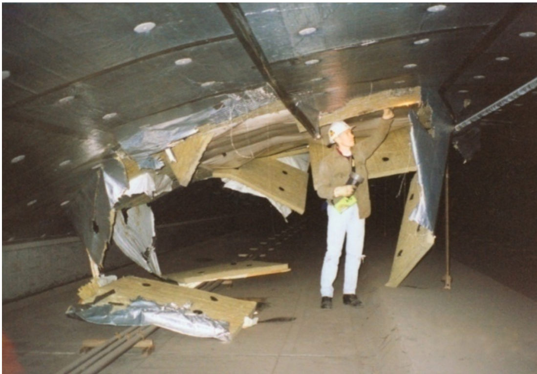
Figure 3.21 – Insulated panels under waterproofing membrane in air plenum region above roadway have dislodged in an isolated location (NCHRP, 2010).
