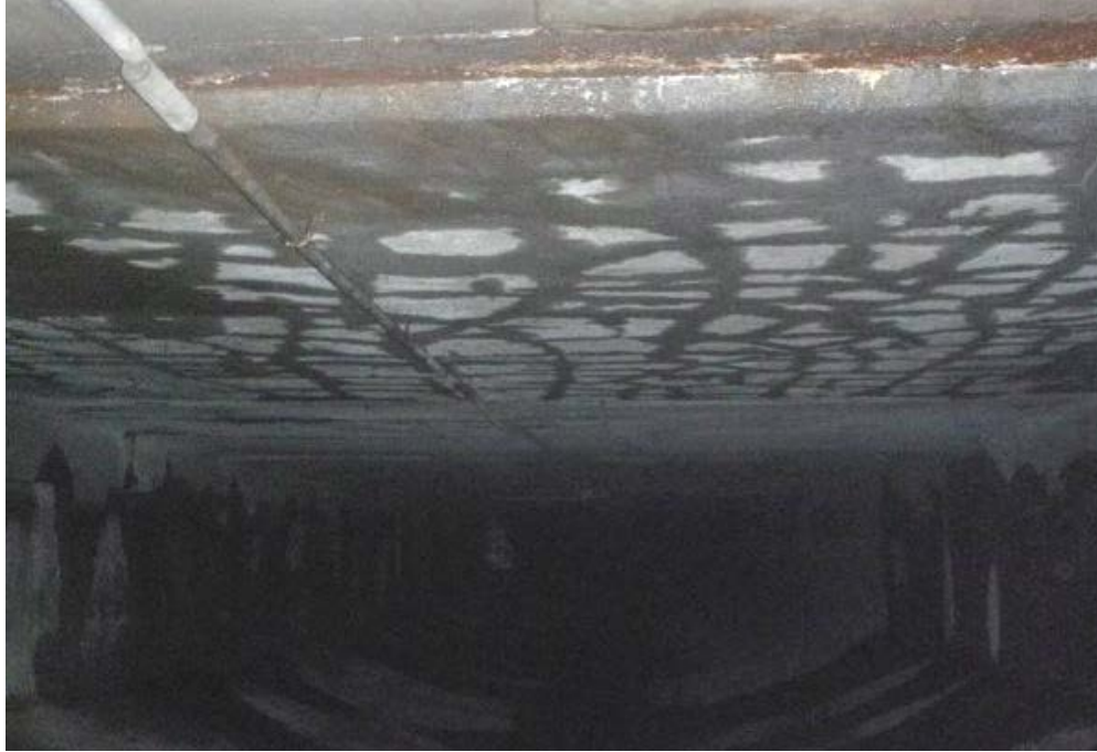
Figure 4.14 – Map or pattern cracks on the underside of an invert slab.
