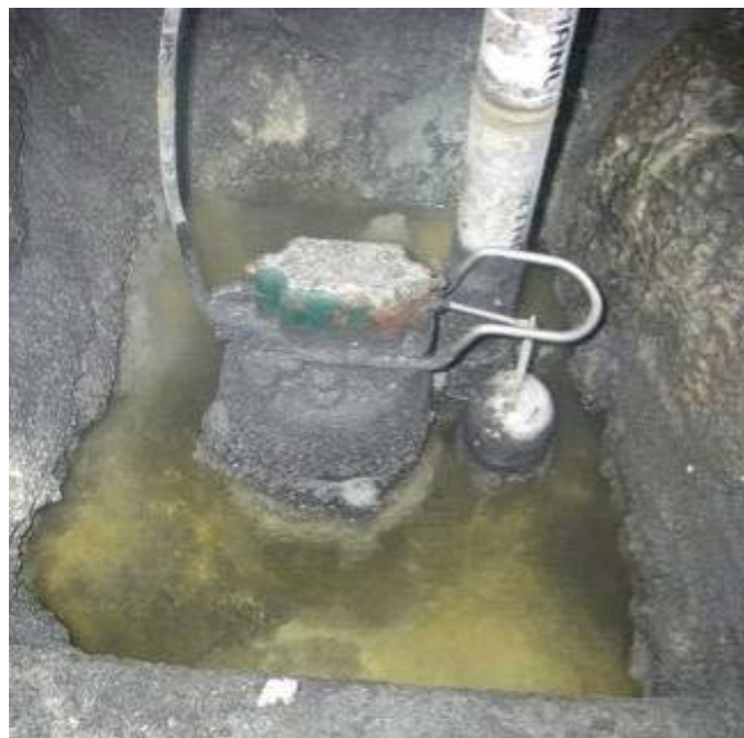
Figure 4.61 – Accumulation of calcium deposits at sump pump.
