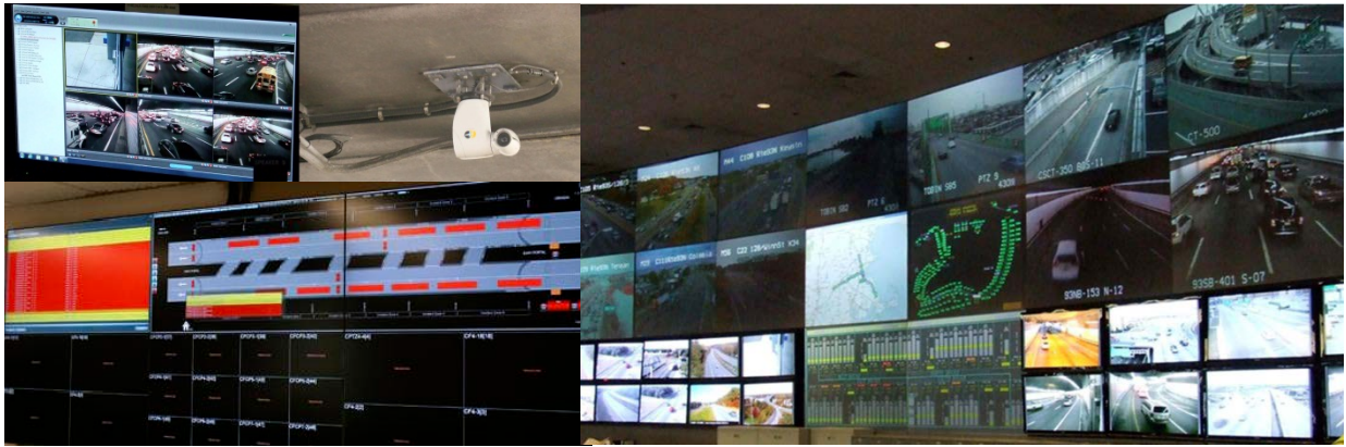
Figure 2.4 – Incident detection systems facilitate a rapid response to the emergency.
