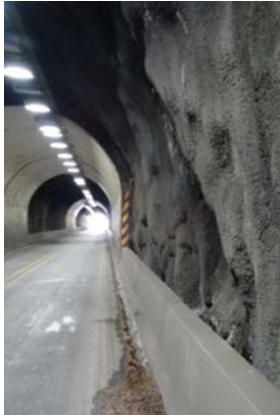
Figure 4.20 B – Shotcrete tunnel liner foreground with adjacent cast-in-place liner concrete liner background.
