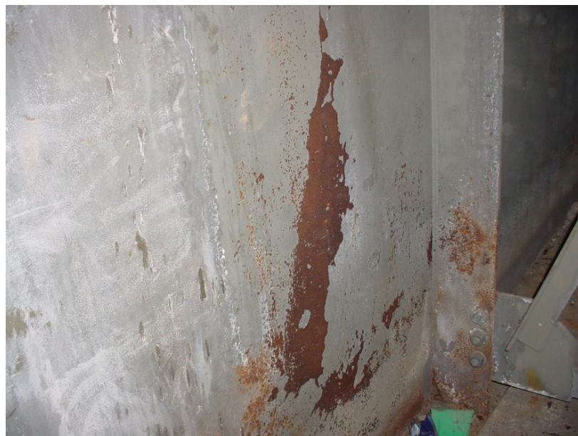
Figure 4.13 – Minor corrosion along roof girder.
