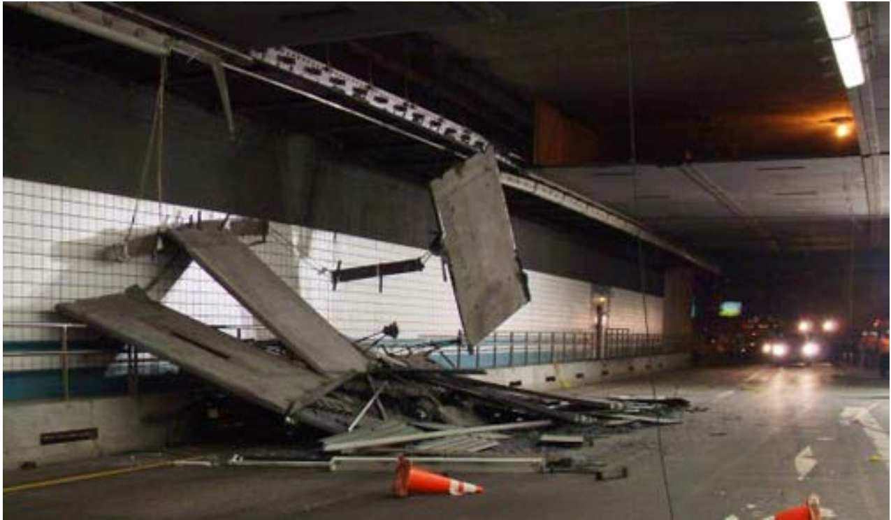
Figure 4.35 – Overhead items such as ceiling panels must be inspected to prevent fatalities.
