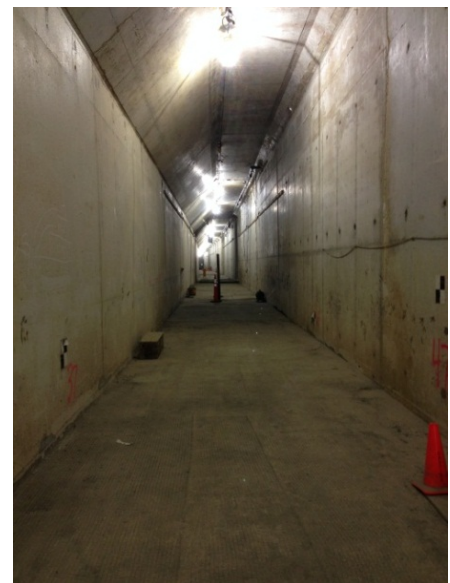
Figure 4.32 – View down emergency corridor. Wall on right is interior wall; wall on left is tunnel liner.
