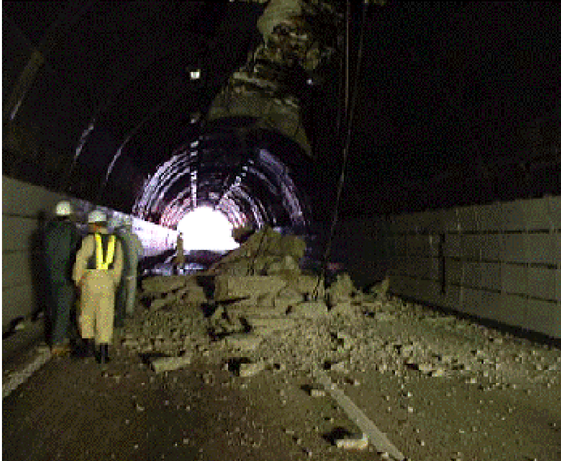
Figure 2.7 – Earthquake damage to tunnels.
