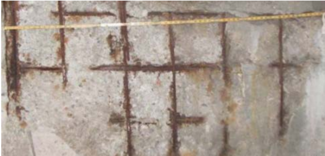
Figure 4.15 – Concrete spalling with exposed reinforcing steel.
