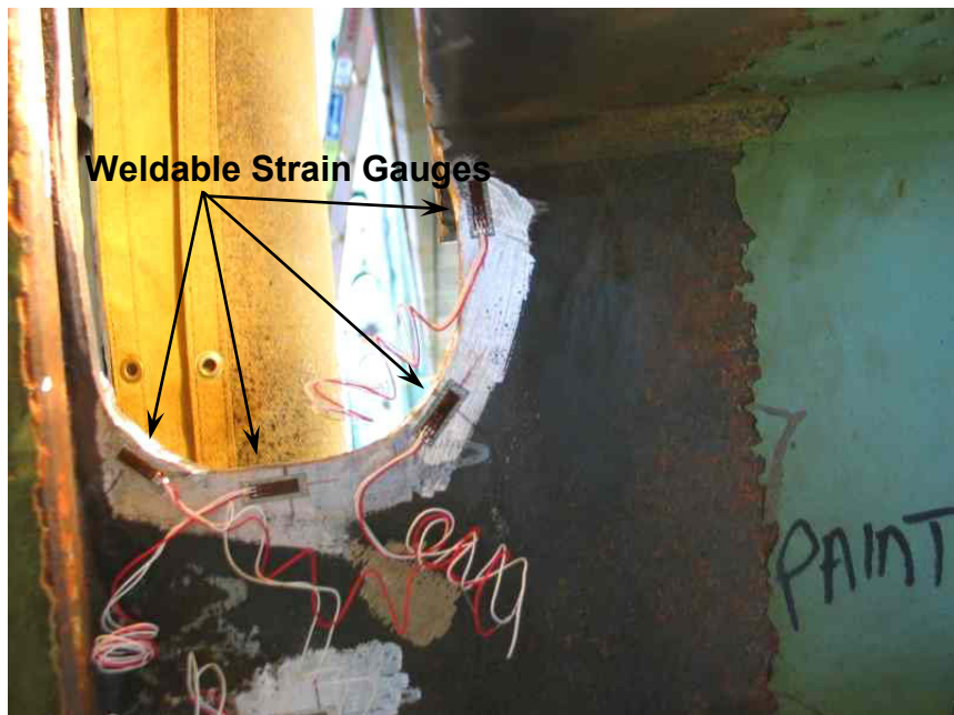
Figure 59. Photo. Weldable strain gauges applied near free edge of retrofit on Girard Point Bridge, Philadelphia, Pennsylvania. Taken from Mahmoud and Connor. (88)
