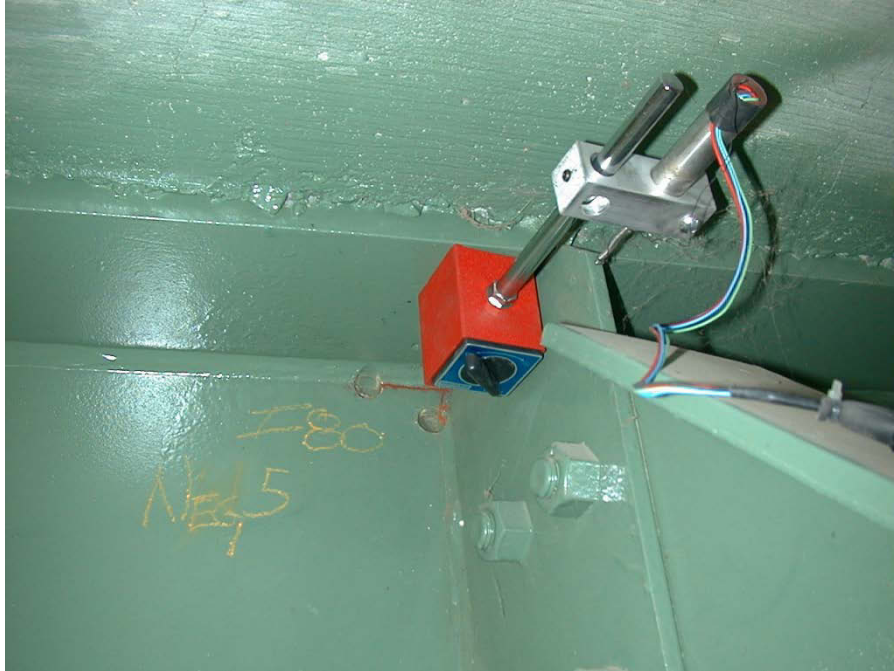
Figure 61. Photo. Magnetic base and LVDT to measure the relative displacement between the girder and connection plate. Photo courtesy of Iowa Department of Transportation.
