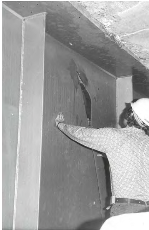
Figure 25. Photo. Full girder depth fatigue crack of Lafayette Street Bridge in St. Paul, MN. Photo courtesy of the Minnesota Department of Transportation.
