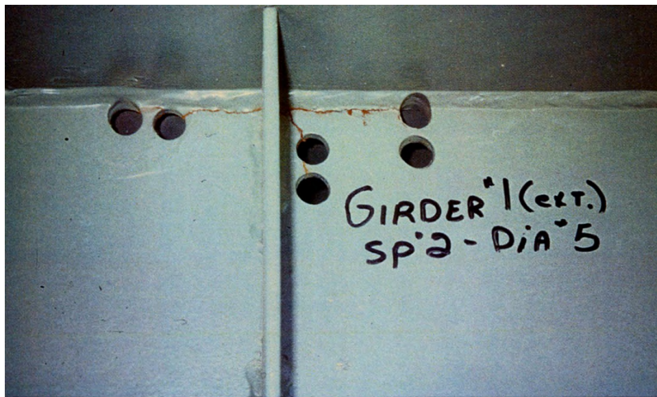
Figure 29. Photo. Picture of multiple drilled holes in the vicinity of the web gap due to crack reinitiation from holes. Photo courtesy of Iowa Department of Transportation.
