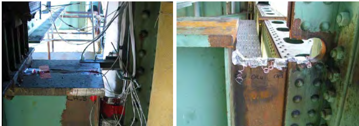
Figure 53. Photo. First retrofit performed on Girard Point Bridge in Philadelphia, Pennsylvania (left) and modified retrofit (right). Taken from Mahmoud and Connor. (88)
