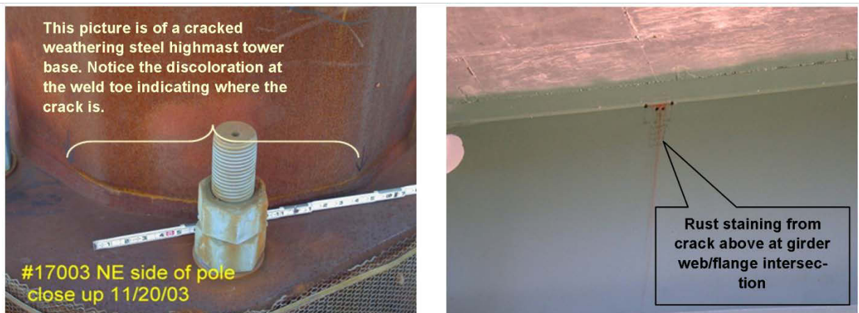
Figure 7. Photo. These two pictures show how cracks can sometimes be found from discoloration or rust staining. Photo courtesy of the Iowa Department of Transportation.
