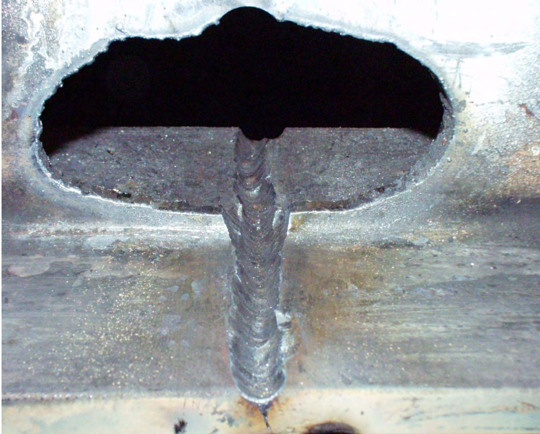
Figure 24. Photo. Air arc gouged flange of a beam for Vee and Weld Repair, which was completely cracked. The hole had to be placed in the web to allow for complete gouging of the flange. The access hole has not been ground smooth as recommended in this manual.
