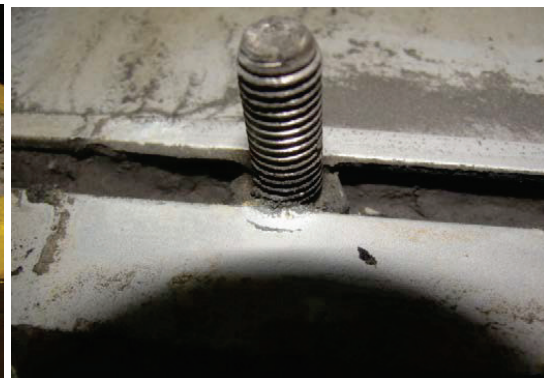
Figure 5. Bolt head in aluminum channel.
