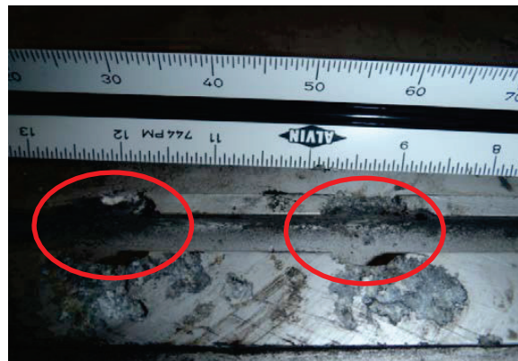
Figure 6. Close up of back of luminaire that fell showing deteriorate aluminum flanges
