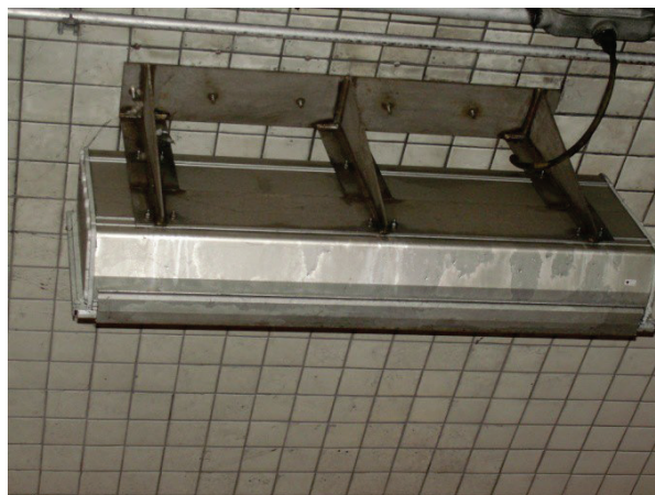
Figure 1. A ceiling mounted luminaire similar to the one that fell.
