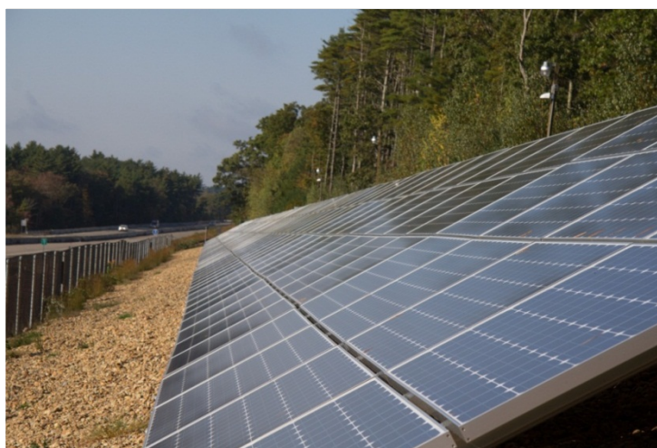
Figure 1: Solar Highway in Carver, Massachusetts
