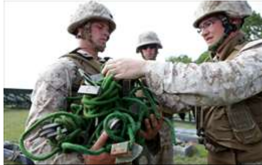
Cpl Colin Smith, a combat engineer with Bridge Co. C, from Memphis, hands out pieces of equipment to build a medium girder bridge during a training exercise here, June 11. The process of putting together an MGB can take upwards of 30 Marines and nearly a day to assemble properly (Photo by Cpl John M. McCall)
