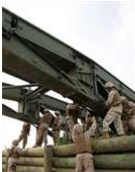
Marines with 6th ESB make adjustments to the underside of a medium girder bridge during a training exercise here, June 11. The base of the bridge must be able to hold massive amounts of weight when it is used to create routes across impassable terrain. (Photo by Cpl John M. McCall)
