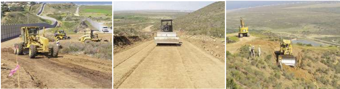
The steep slopes on the west side of Bunker Hill presented a significant challenge as the slump of the concrete varied from three to five.
