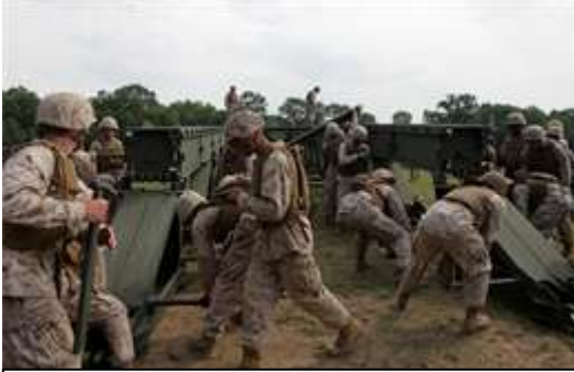
Marines with 6th ESB assemble a medium girder bridge during a training exercise here, June 11. Marines participated in a two-week training exercise that covered basic combat engineer capabilities such as: demolition, construction and bridging. (Photo by Cpl John M. McCall)
