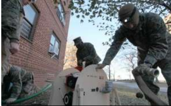
Marines with 8th ESB, 2nd MLG hook hoses up to a pump in order to extract water from a flooded basement of a building while conducting humanitarian operations in Far Rockaway, N.Y., Nov. 4. Approximately 86 Marines with 8th ESB, 2nd MLG were deployed to New York to help with relief of Hurricane Sandy by pumping water out of flooded buildings. (Photo by LCpl Scott W. Whiting)
