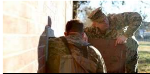
Sgt Justin Armstrong, a Marine with 8th ESB, 2nd MLG, and GySgt Justin Gober, a Marine with 8th ESB, 2nd MLG, examine the depth of a basement in order to pump water out into the street while conducting humanitarian operations in Far Rockaway, N.Y., Nov. 4. Approximately 86 Marines with 8th ESB, 2nd MLG were deployed to New York to help with relief of Hurricane Sandy by pumping water out of flooded buildings. (Photo by LCpl Scott W. Whiting)
