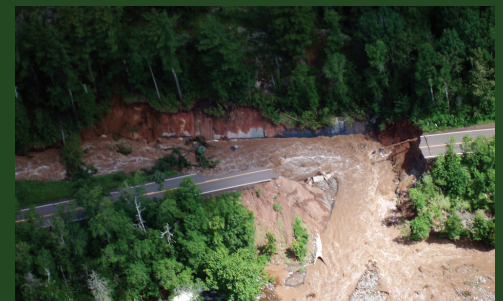
Roadway collapse during flood event. Photo credit: MnDOT.
