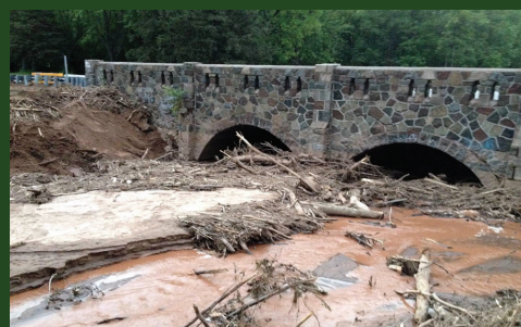
Bridge filled with debris during flood event. Photo credit: MnDOT.
