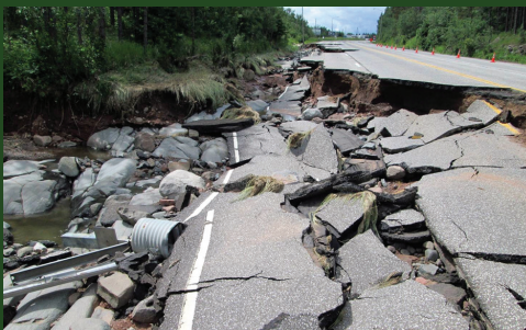
Roadway erosion following flooding event. Photo credit: MnDOT.
