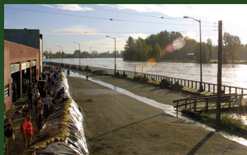
Flood-fighting efforts in Mount Vernon. Photo credit: WSDOT
