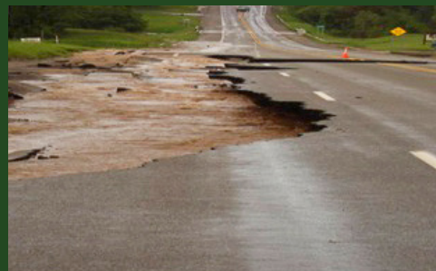
Road collapse in Michigan. Photo credit: MDOT
