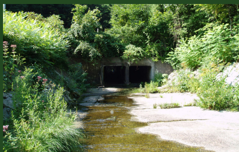
Two cell box culvert in rural Connecticut. Photo credit: ConnDot Hydraulics and Drainage Section.
