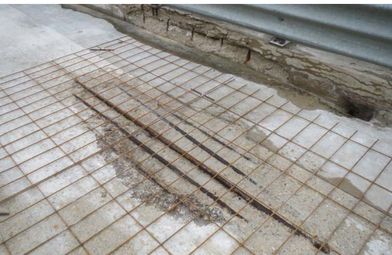
Before the bridge deck was rehabilitated, potholes exposed the deck's top reinforcement.
