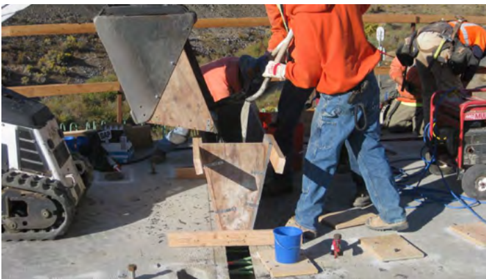
Above: Crews place UHPC in the transverse joints on Oregon's Burnt River Bridge project.
