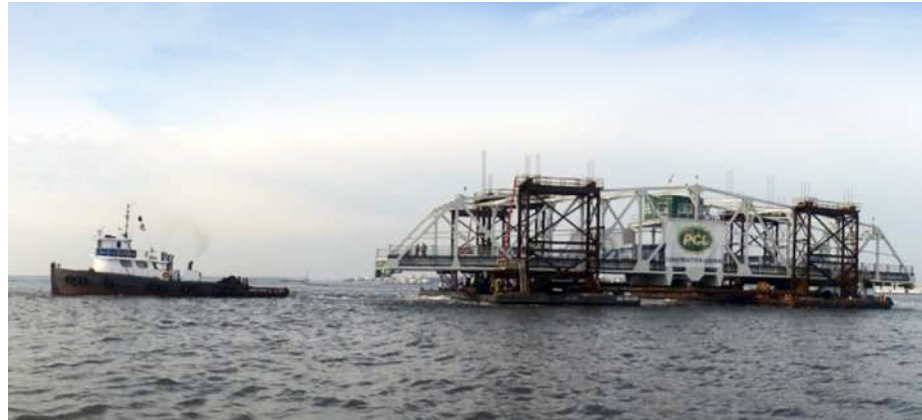
To limit bridge closure time on a South Carolina project, the new swing span was built off-site and moved to the bridge site on a barge.
