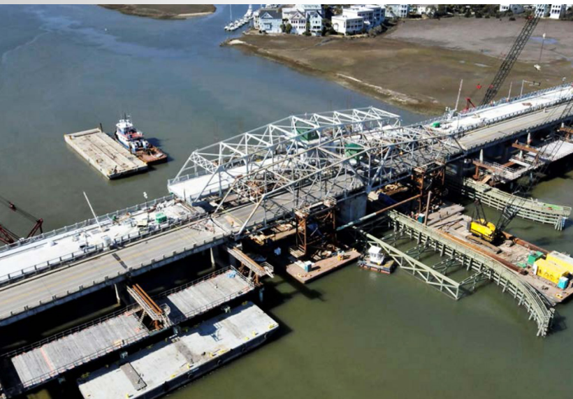
The new superstructure (back) was slid into place after the old one (front) was moved onto temporary supports.
