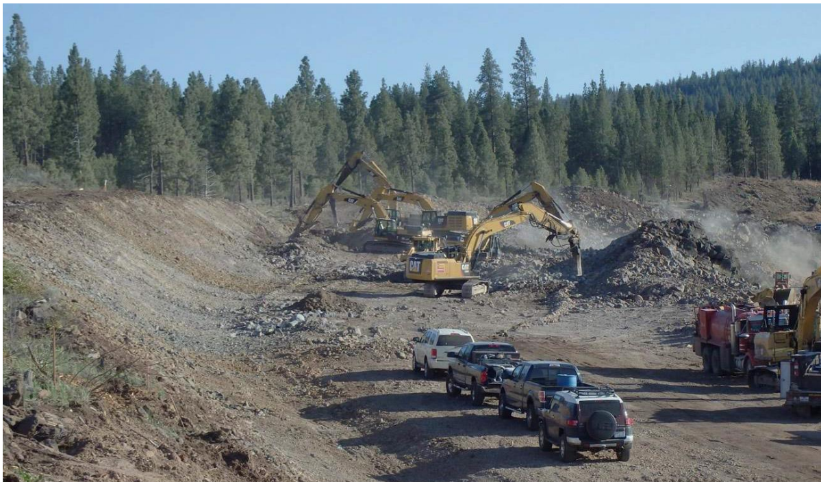
K&E Excavating of Salem, Oregon, used Automated Machine Control from 3D Design on ODOT's Oregon Highway 140 Bly Mountain Project. (ODOT photo, May 2015)
