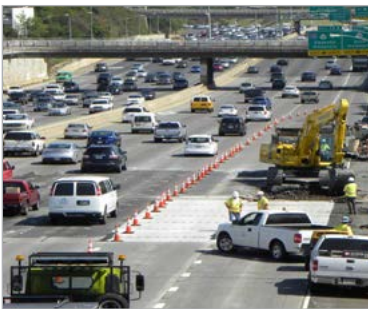
Multiple lane replacement with jointed PCP on Interstate H-1 in Hawaii. (Photo Source: Shiraz Tayabji, ARA Associates, Inc.)
