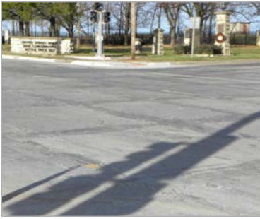
Intersection outside Ft. Leavenworth repaired with PCP. (Photo Source: Shiraz Tayabji, ARA Associates, Inc.)
