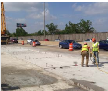
The Illinois Tollway is using PCP for the replacement of bridge approaches to minimize traffic delays. (Photo Source: Illinois Tollway)
