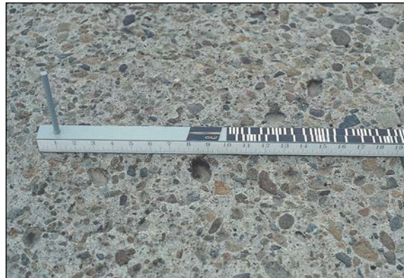
FIGURE 105 Distress Type CRCP 6—Popouts.
