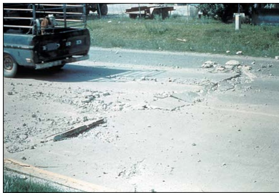
FIGURE 76 Distress Type JCP 11—A Blowup.
