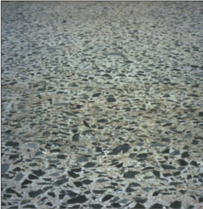
FIGURE 103 Distress Type CRCP 5—Polished Aggregate.
