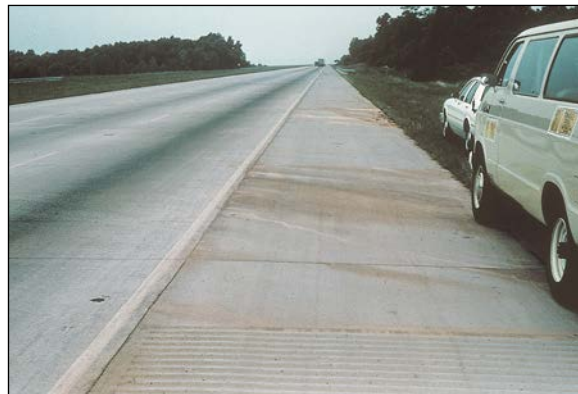
FIGURE 131 Distress Type CRCP 14—Water Bleeding and Pumping.
