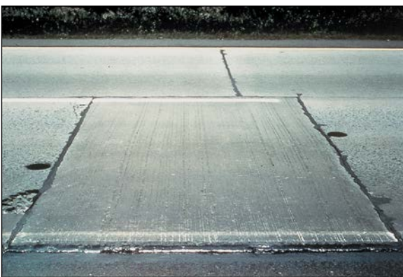
FIGURE 88 Distress Type JCP 15—Large, Low Severity PCC Patch.
