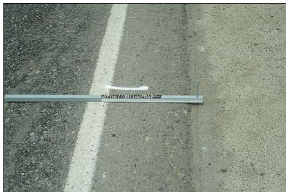
FIGURE 44 Distress Type ACP 14—Lane-to-Shoulder Dropoff.
