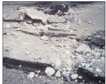
FIGURE 108 Distress Type CRCP 7—Close-up View of a Blowup.
