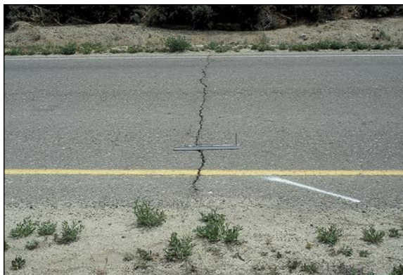
FIGURE 21 Distress Type ACP 6—High Severity Transverse Cracking.
