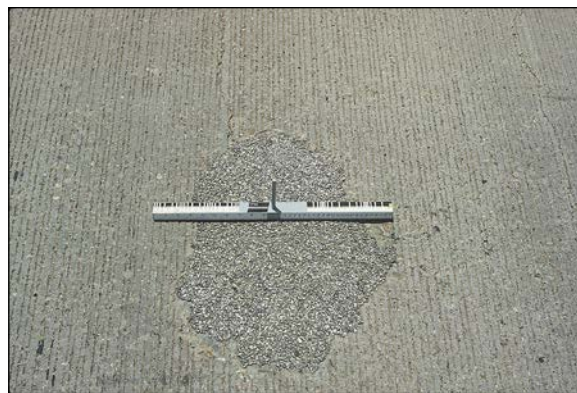
FIGURE 119 Distress Type CRCP 11—Small, Low Severity AC Patch.
