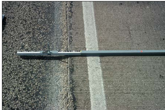
FIGURE 80 Distress Type JCP 13— Lane-to-Shoulder Dropoff.
