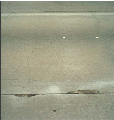
FIGURE 130 Distress Type CRCP 13—Moderate Severity Spalling of a Longitudinal Joint.
