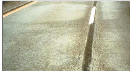
FIGURE 92 Distress Type CRCP 1—High Severity “D” Cracking at Longitudinal Joint.
