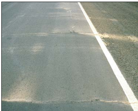
FIGURE 46 Distress Type ACP 15—Fine Material Left on Surface by Water Bleeding and Pumping.
