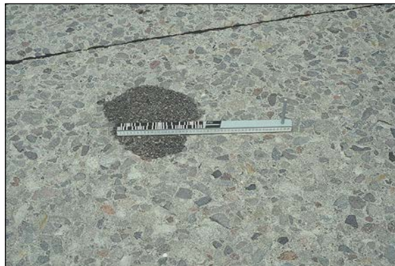
FIGURE 85 Distress Type JCP 15—Small, Low Severity AC Patch.
