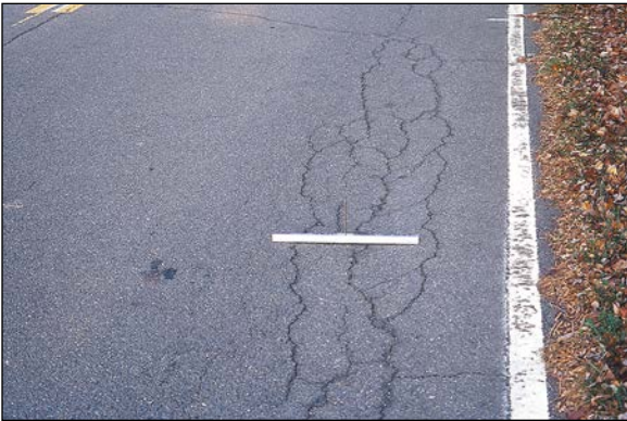
FIGURE 6 Distress Type ACP 1—Moderate Severity Fatigue Cracking.
