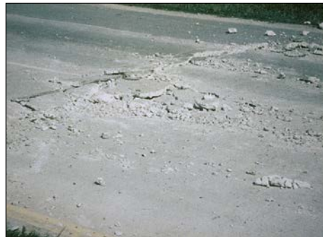
FIGURE 107 Distress Type CRCP 7—A Blowup.
