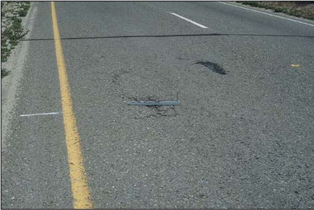
FIGURE 27 Distress Type ACP 8—Low Severity Pothole.
