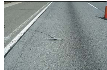
FIGURE 50 Distress Type JCP 1—Moderate Severity Corner Break.
