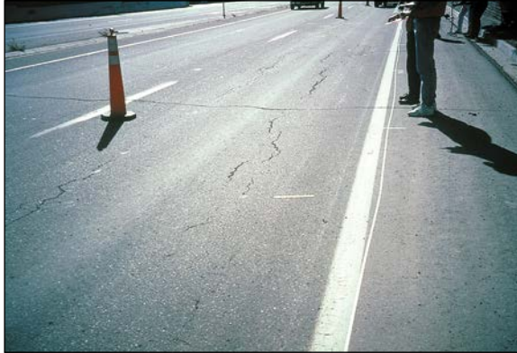
FIGURE 5 Distress Type ACP 1—Low Severity Fatigue Cracking.
