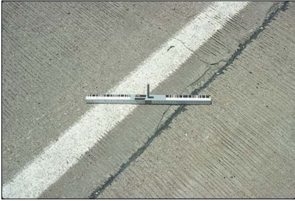
FIGURE 128 Distress Type CRCP 13—Close-up View of Low Severity Spalling of a Longitudinal Joint.
