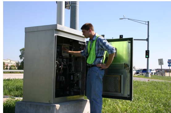
Operation Green Light technician adjusts signal timing at traffic signal cabinet. (Courtesy Mid-America Regional Council)
