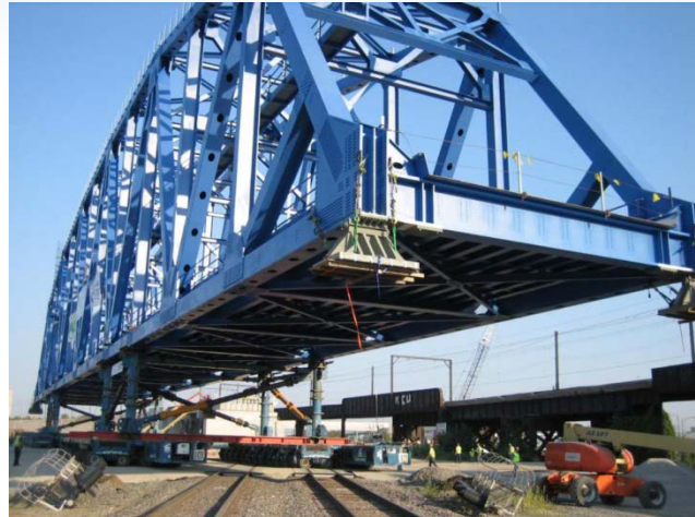
CREATE grade separation project GS15a under construction at 130 th St. and Torrance Ave. in Chicago
