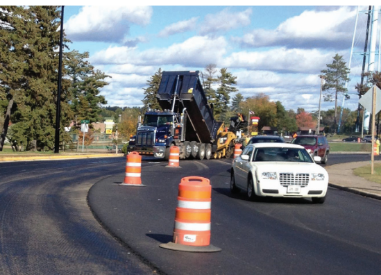
Wisconsin DOT applies a pavement preservation treatment using the Guidelines for the Preservation of High-Traffic-Volume Roadways. | Photo courtesy WisDOT
