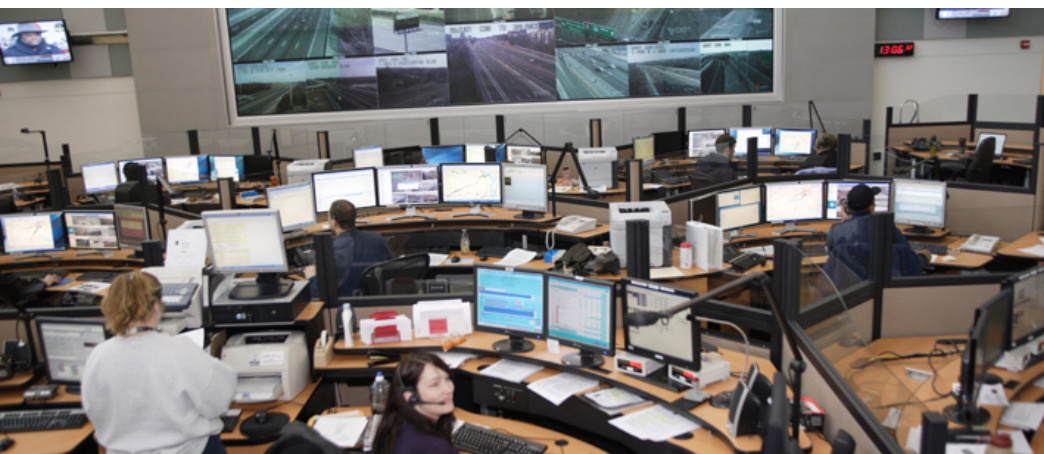
A traffic operations center in Fairfax County, VA | Photo courtesy Trevor Wrayton, VDOT
