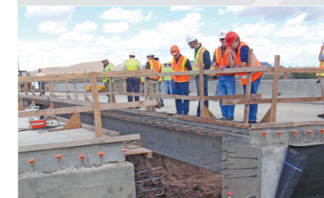
Engineers observe the "side-slide" bridge project at the Gila River Indian Community in Sacaton, AZ during a showcase event for Innovative Bridge Designs for Rapid Renewal . | Photo courtesy Finn Hubbard, Fish & Associates
