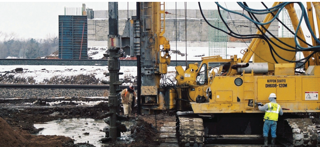
Knowing the proper soil conditions before construction begins is critical to keeping on budget and on schedule. | Photo courtesy Ryan Berg
