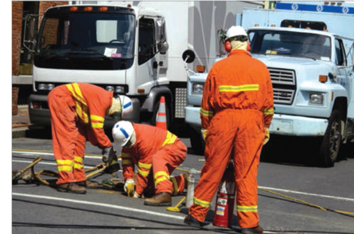
Gas company employees repairing a utility line on a road in Alexandria, VA | Photo courtesy Liz Roll, FEMA
