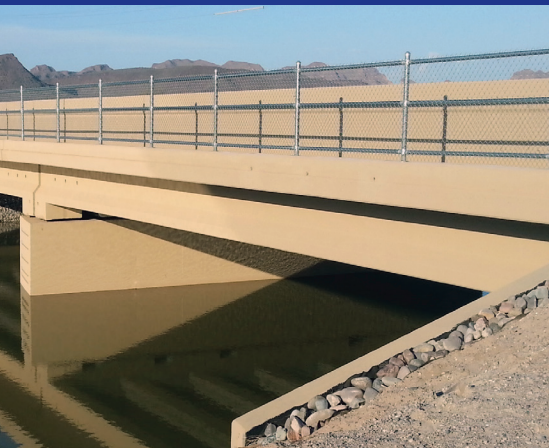
The Sacaton Bridge was replaced using the Innovative Bridge Designs toolkit and was the first "bridge slide" project used by a tribal nation. | Photo courtesy Gila River Indian Community
