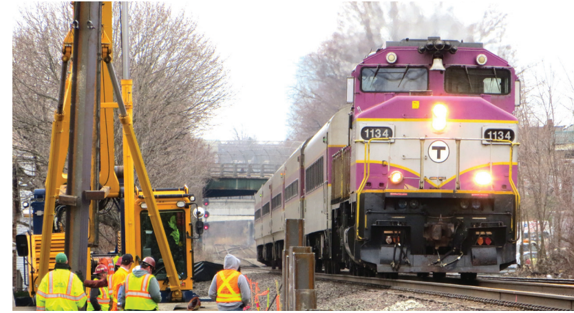
To coordinate a bridge removal project in Oregon over Burnt River and the Union Pacific Railroad, transportation officials used SHRP2's Railroad DOT Mitigation Strategies . | Photo courtesy FHWA
