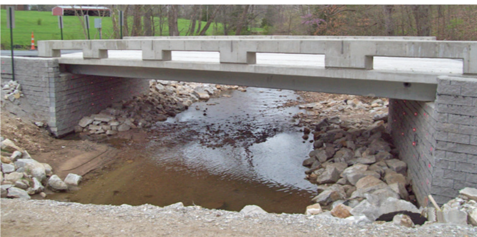
The completed Rustic Road Bridge, Boone County, MO | Photo courtesy Derin Campbell
