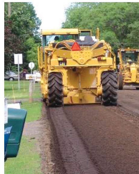
Performance specifications can result in faster project delivery, minimal disruption, and greater durability. | Photo courtesy Gallivan Consulting, Inc.
