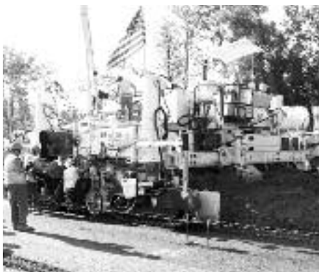
Sustainable strategies applied to the concrete pavement construction on I-90 included the use of fly ash in the concrete.
