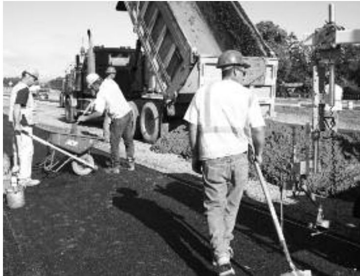
Long-life concrete pavement under construction along a section of I-90 near Syracuse, NY.
