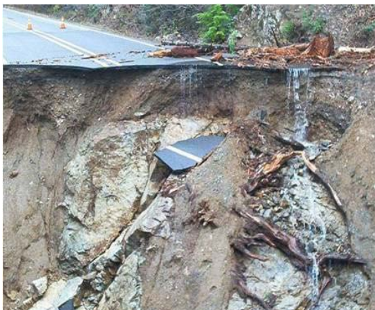
Slope Failure. SR 12. Source WSDOT
