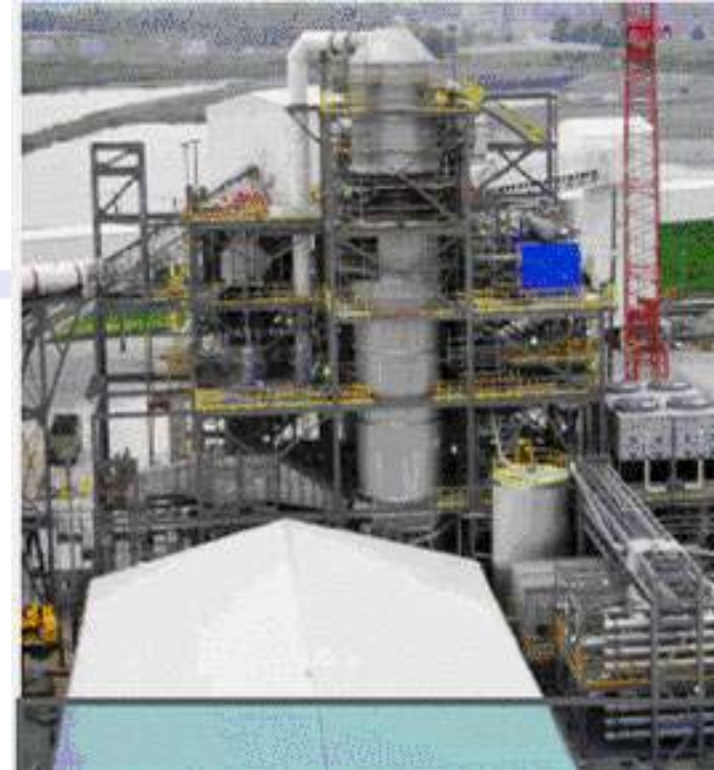
Alstom's Chilled Ammonia Process at AEP's Mountaineer Plant, 5-21-09
