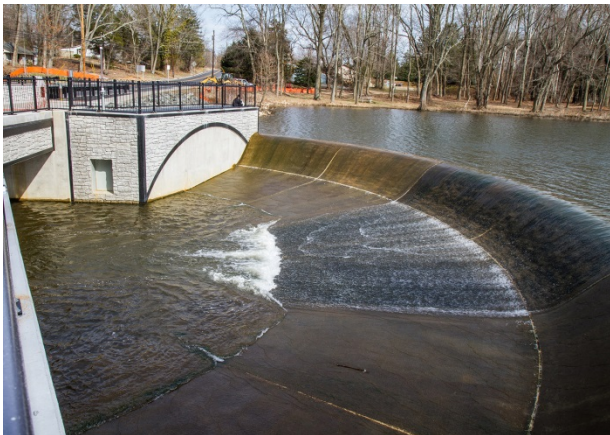
Figure 1: The newly designed bridge, dam, and spillway provide safety and resiliency while allowing for new recreational opportunities for local residents. (Image courtesy of NJDOT)
