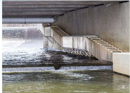
Figure 2: Prior to Tropical Storm Irene, fish could not properly migrate upstream. The US 322 Bridge Project provided NJDOT with an opportunity to correct this design error. (Image courtesy of NJDOT)
