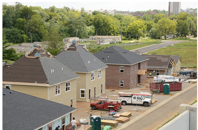
Figure 3: Construction of housing in Davis Park (Photo courtesy of Bernadette Dupont, FHWA)
