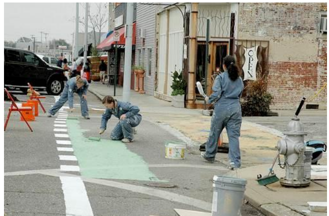
Figure 13: Painting a temporary bicycle lane for the weekend event, A New Face for An Old Broad . (Image courtesy of ioby )
