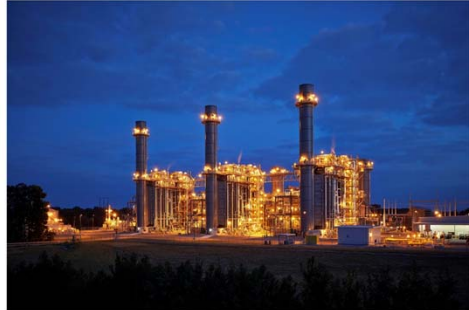
Photo credit: Duke Energy H.F. Lee natural gas plant 1; Goldsboro, NC Taken on September 24, 2013
