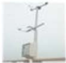
weather monitoring system
