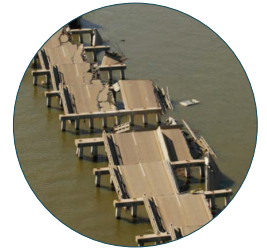
Hurricane Damage from Wave Action to Highway 90 in Bay St Louis, MS Source: Illinoisphoto.com
