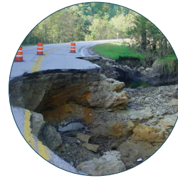
Roadway collapse from flooding from heavy rain in Minnesota Credit: Minnesota DOT
