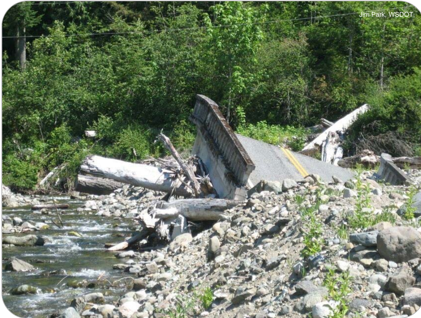
Scour and damage to structures - Just off US 12 Davis Creek
