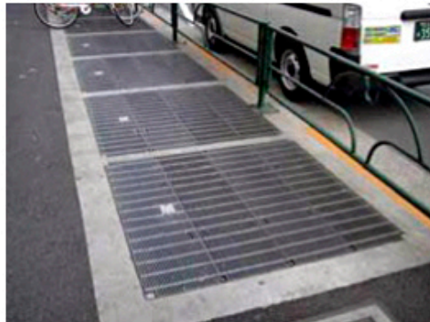
Outlet of a Ventilation Duct
