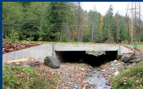
Box culvert in place replaced a small culvert on SR 542, improving drainage and fish passage. Photo courtesy of WSDOT.
