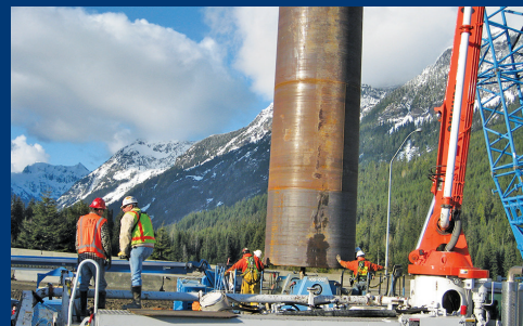
Drilled shafts support new bridge at Gold Creek on I-90, improving resistance to high-velocity flooding. Photo courtesy of WSDOT.
